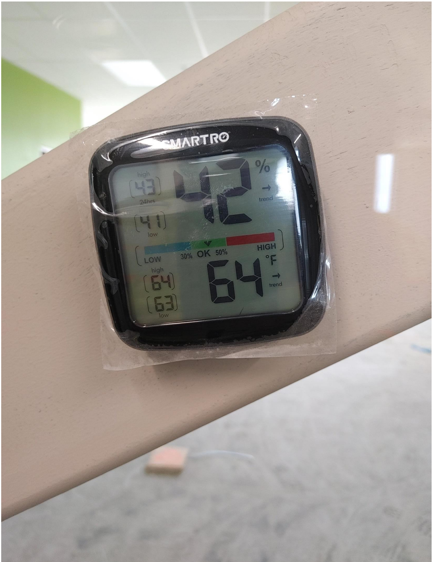
Photo 14 - Digital Temperature & Humidity Monitor on the 2nd floor of Area A
