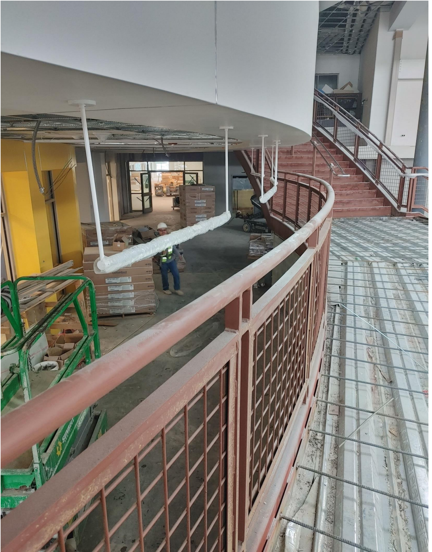
Photo 20 - Lights accessible from Grand Staircase Landing.
