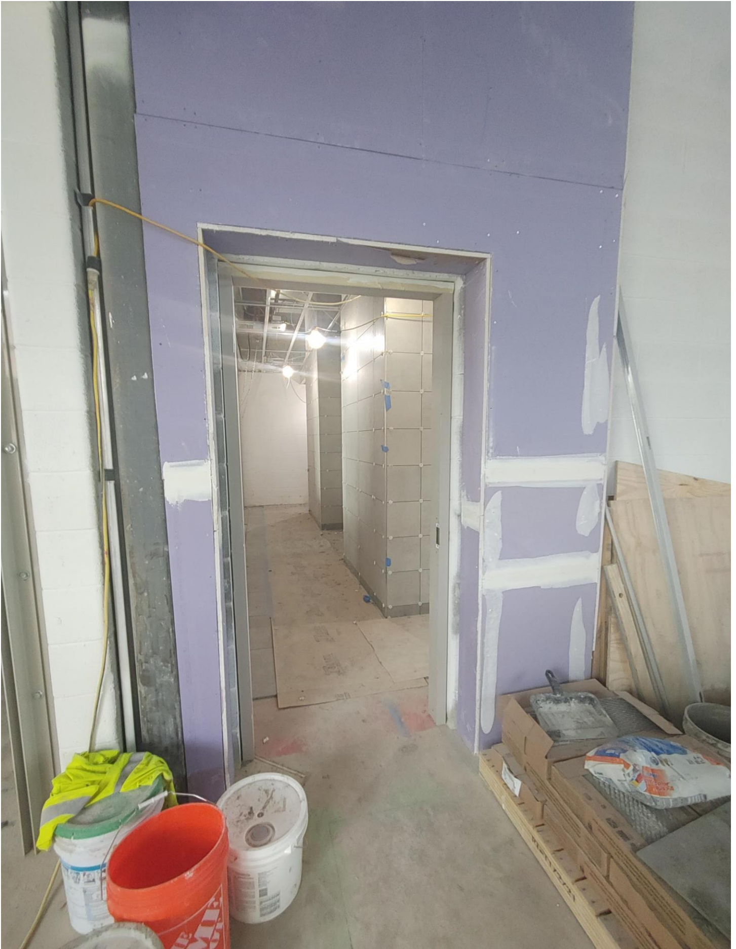
Photo 10 - Wall tile has been set in Vestibule E105. Still needs to be grouted.
