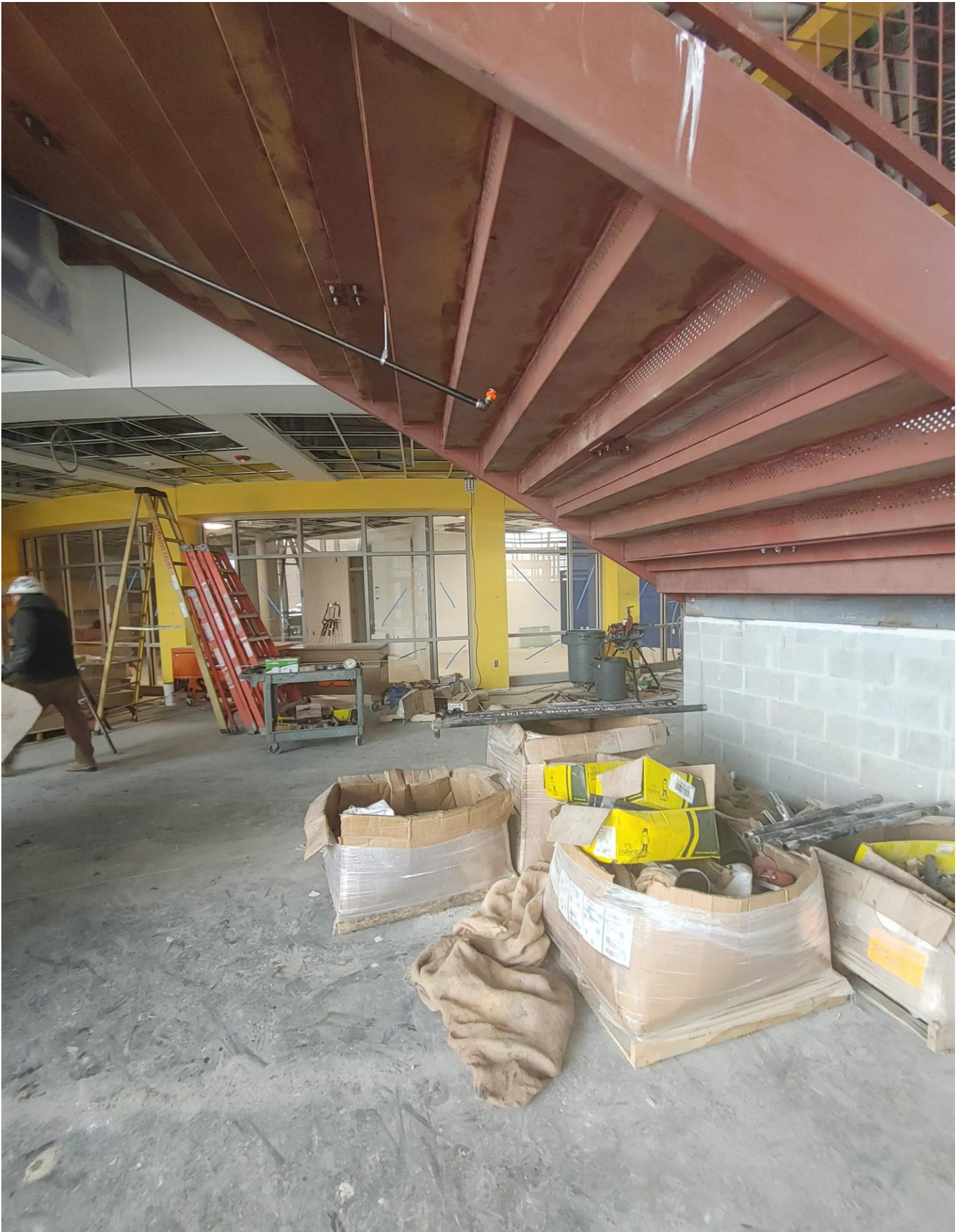
Photo 19 - Sprinkler pipe and head under Grand Staircase.
