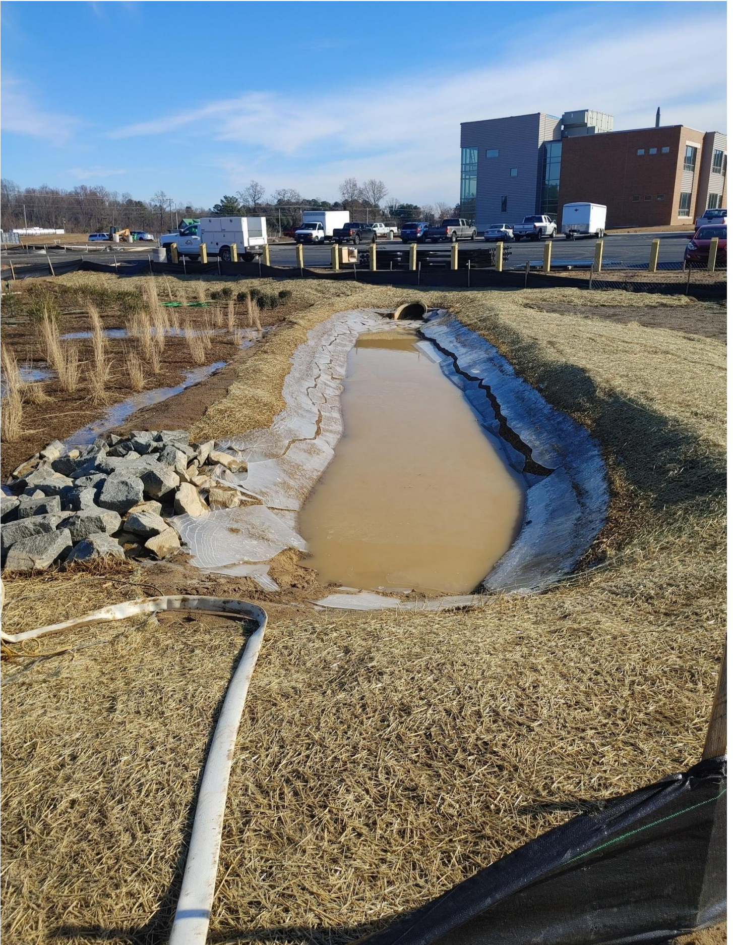
Photo 16 - Bio-Retention Pond on West side of Site.
