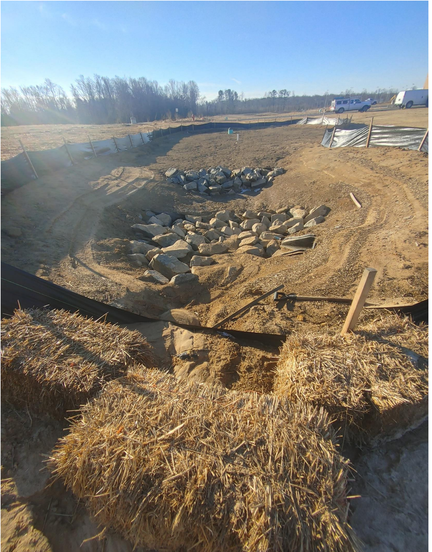
Photo 1 - BMP2B silt fence in need of repair.
