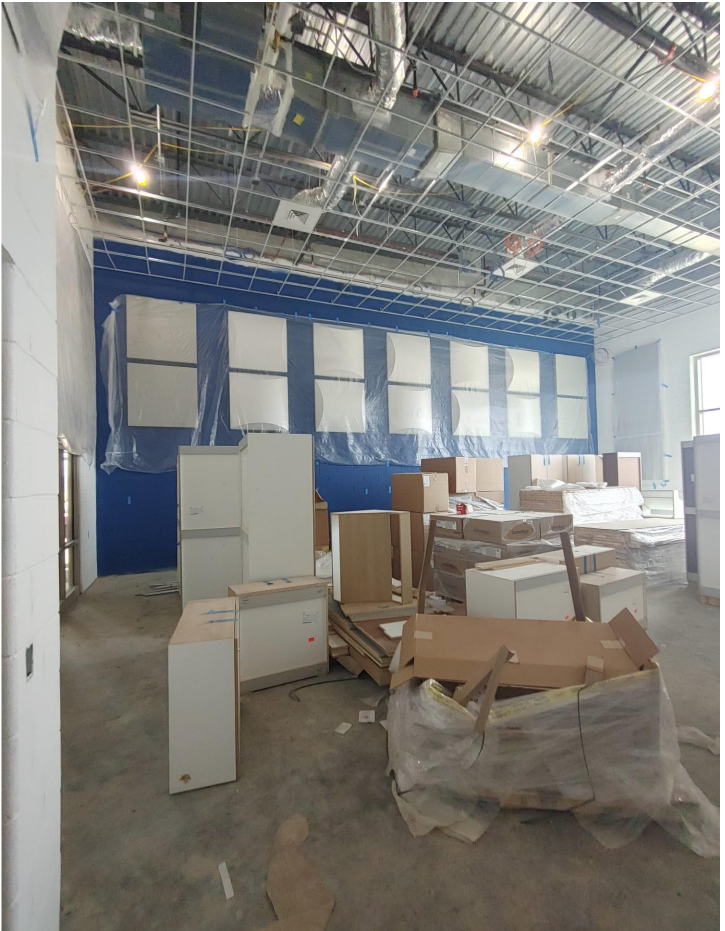
Photo 7 - Acoustical Panes have been hung on the East wall of D127
