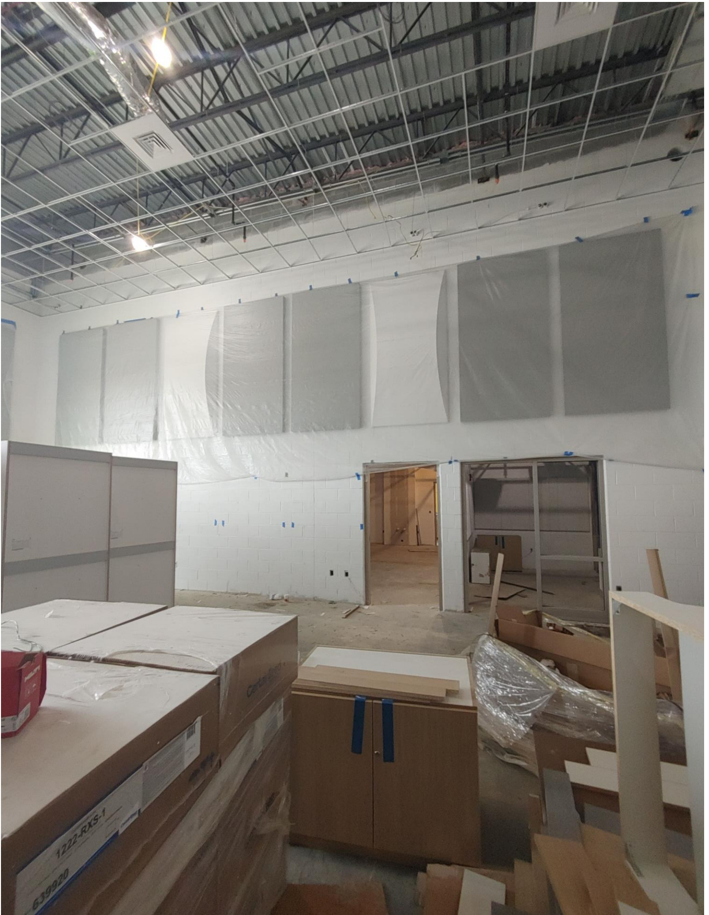
Photo 8 - Acoustical Panes have been hung on the West wall of D127
