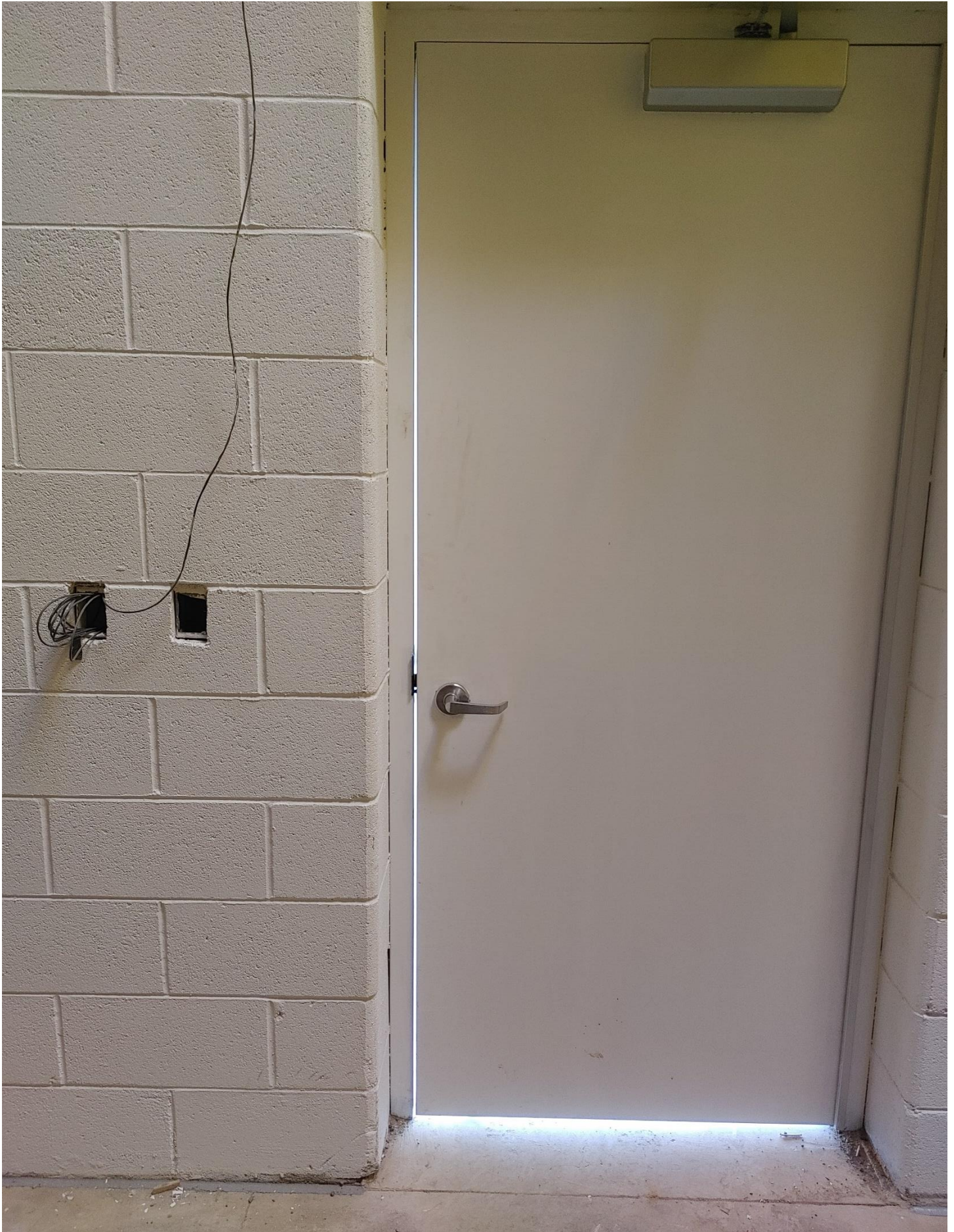
Photo 11 - XD09 is out of Plumb and will not latch.
