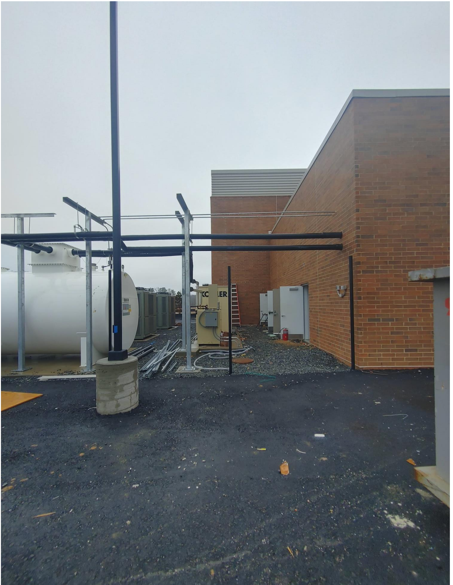
Photo 12 - Piping from Fuel Tank to Mechanical Room appears to be sagging. Is additional bracing needed?
