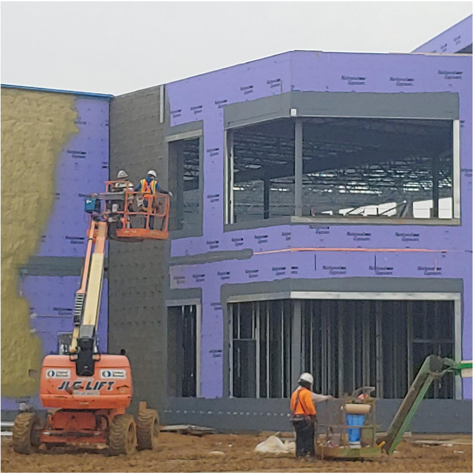
Photo 3 - Bent Galvanized Metal being installed for Storefronts on the Northside of Area A
