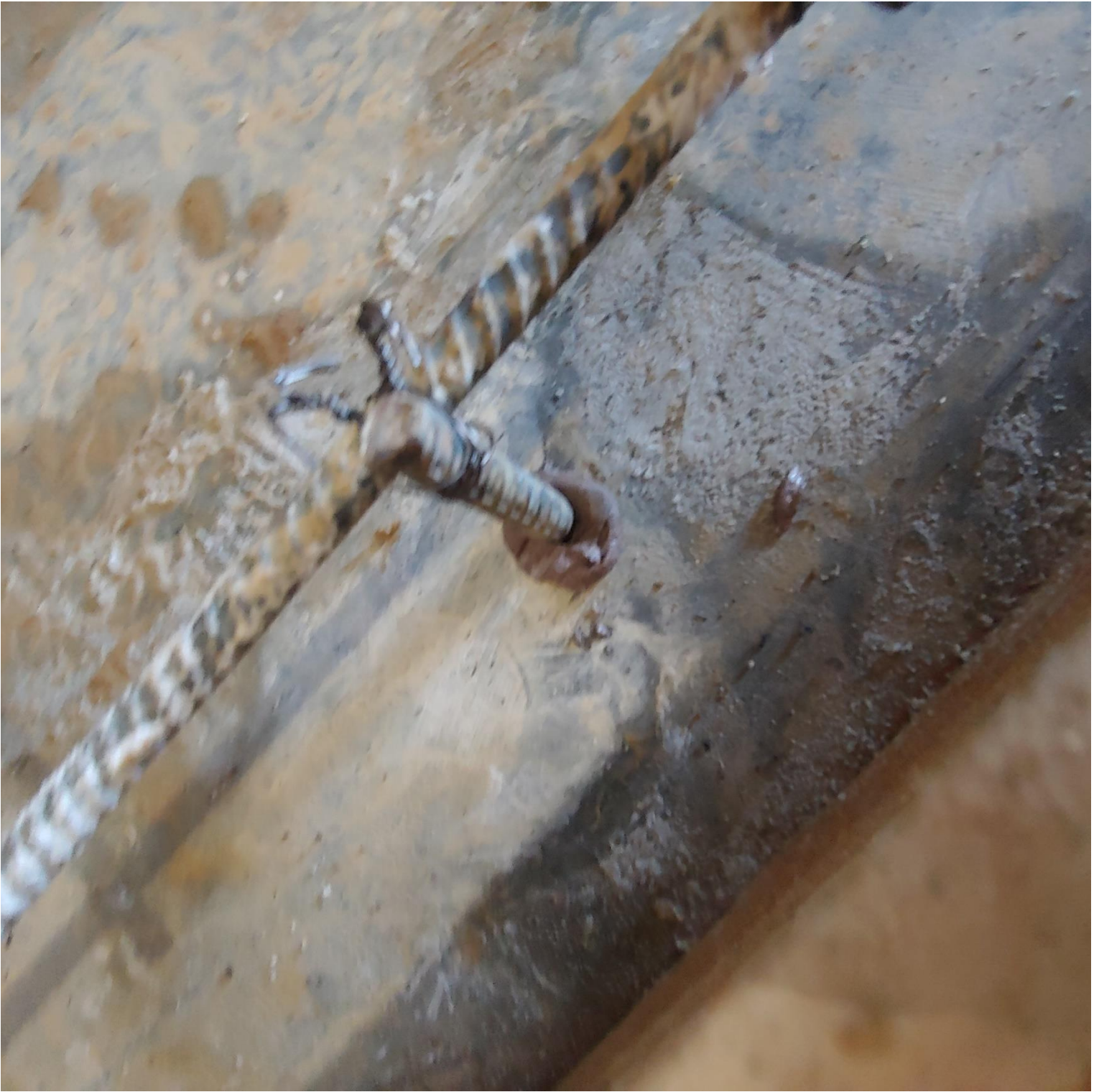
Photo 7 - Verification that epoxy was used to secure steel in the Electrical room D158 forms.
