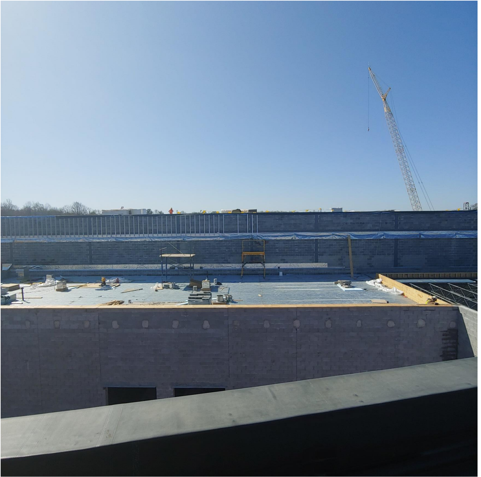
Photo 4 - Roofers installing Foam Board on the High Roof of Area D and Flashing being installed on the low Roof of Area D
