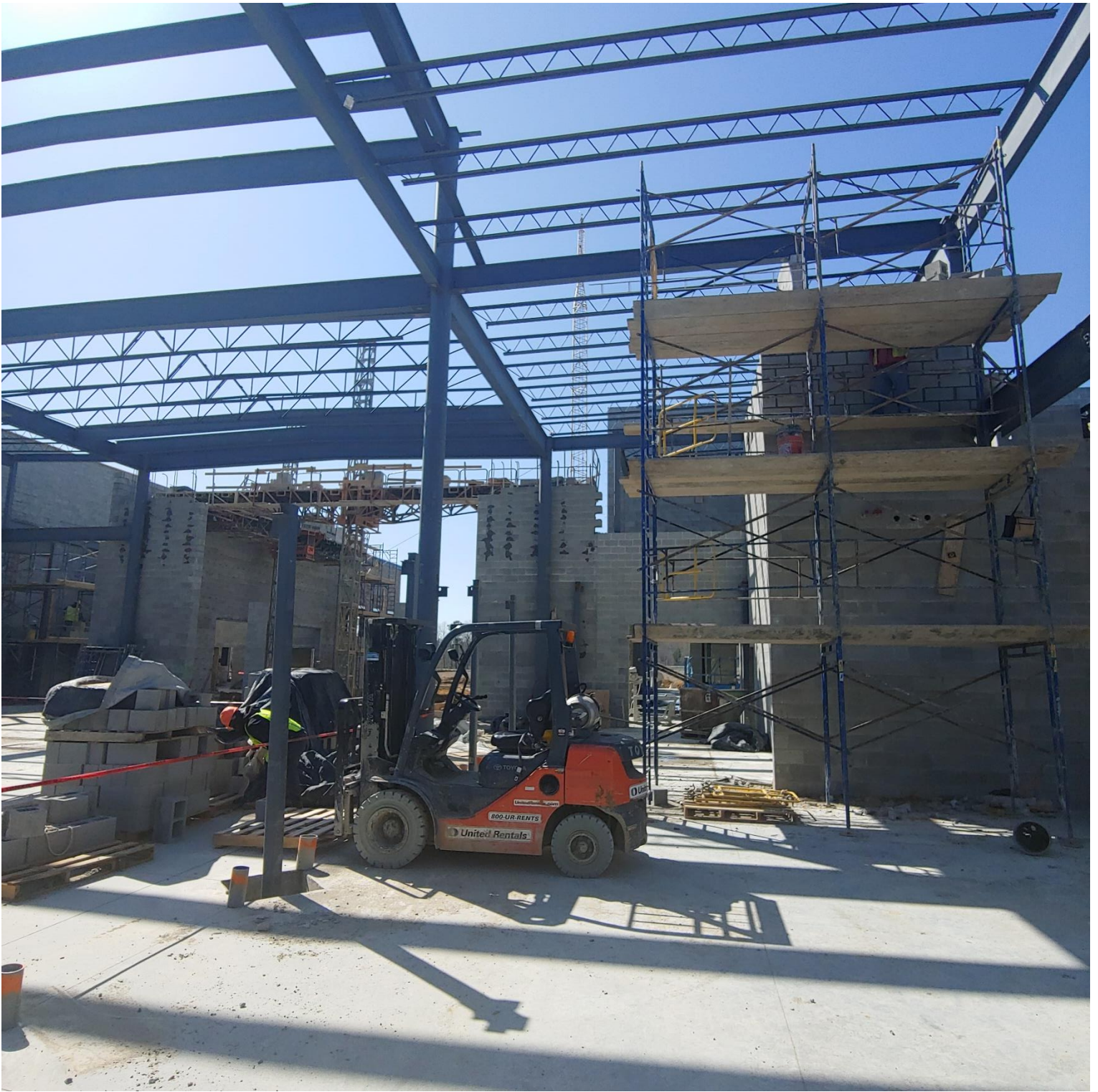
Photo 7 - Block grouted on the South exterior wall of Area C and Block being laid in E103 and E104
