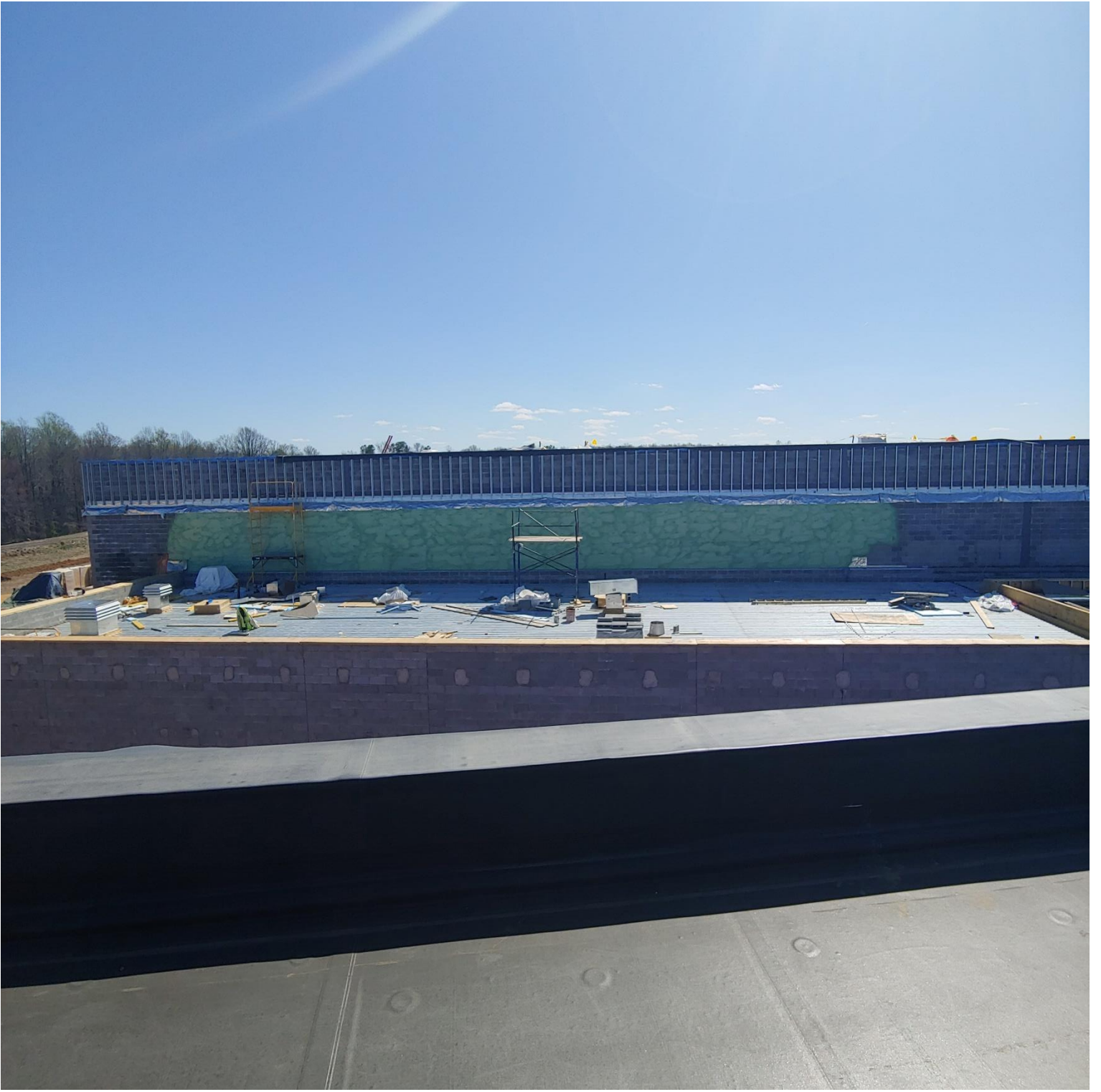
Photo 7 - A section of the North wall of the Auditorium has been spray foamed.
