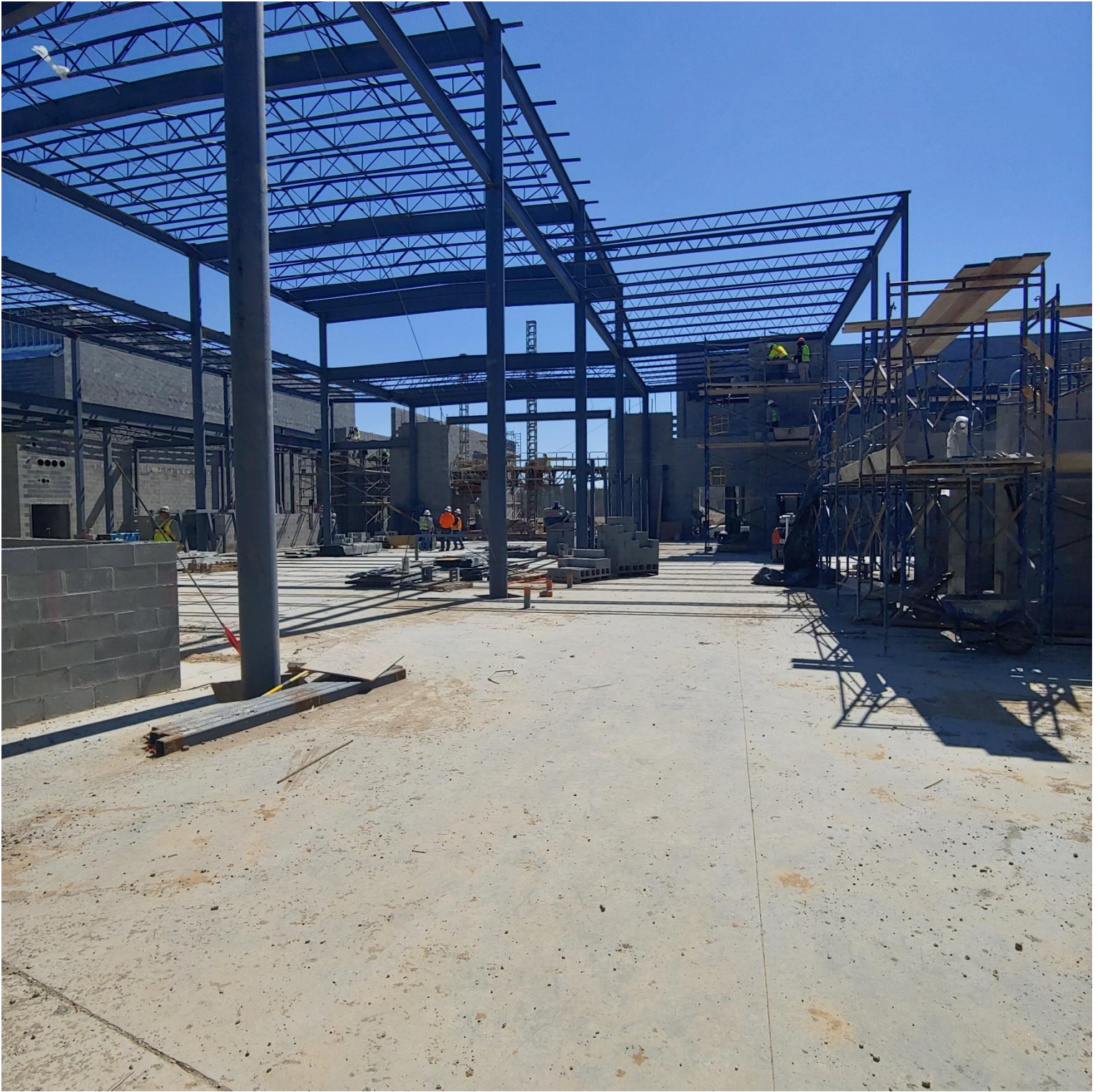
Photo 1 - Steel is being welded in Area C and the Masons are laying block in Areas D & E.
