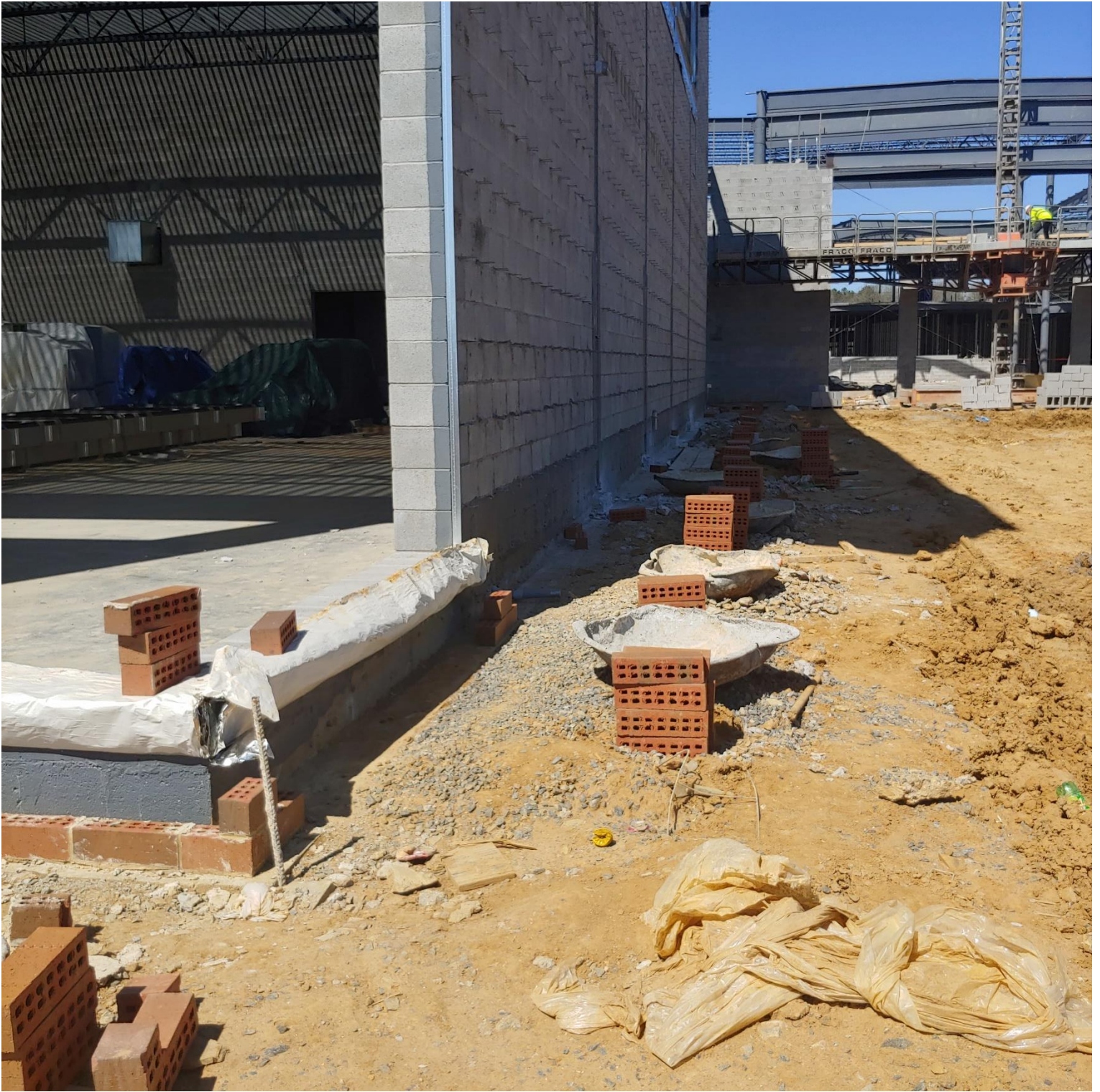
Photo 5 - Brick continues to be laid on the Eastside of the Gym, Area E.
