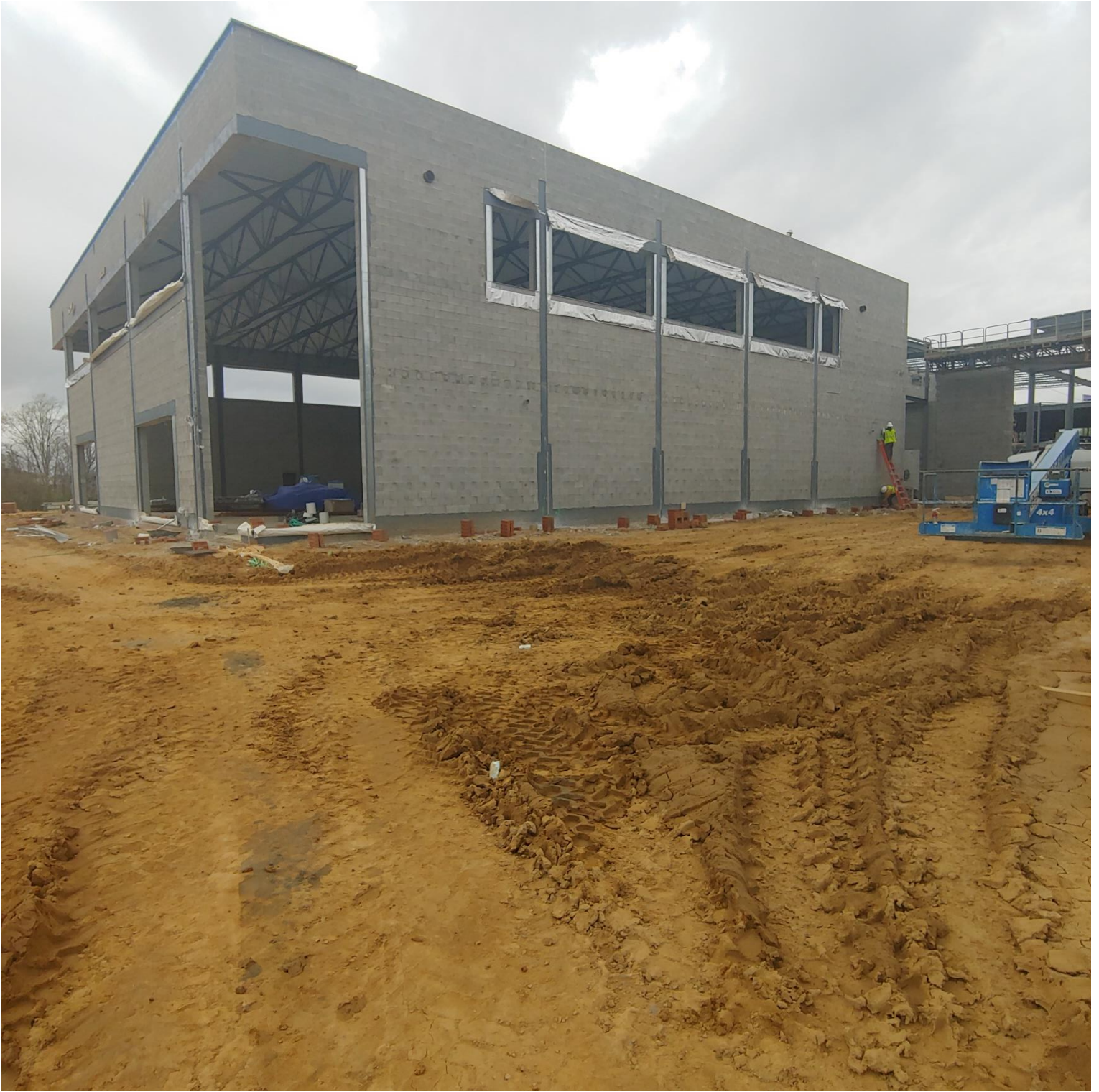
Photo 4 - Electrician running conduit on the Eastside of Area E for exterior lighting
