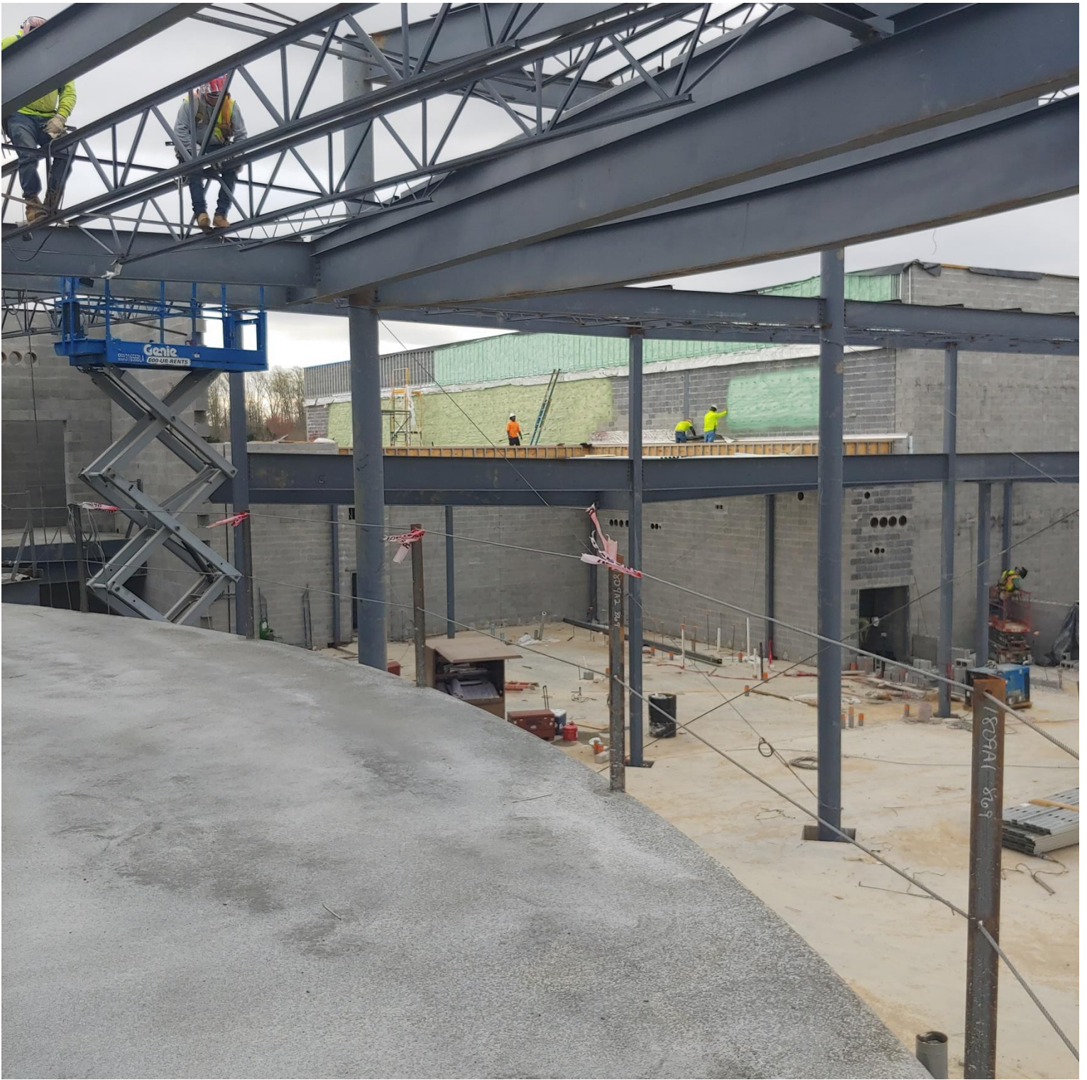
Photo 2 - Lateral Truss Bracing being set and welded in Area A & C. Flashing being installed on the low roof of Area D.
