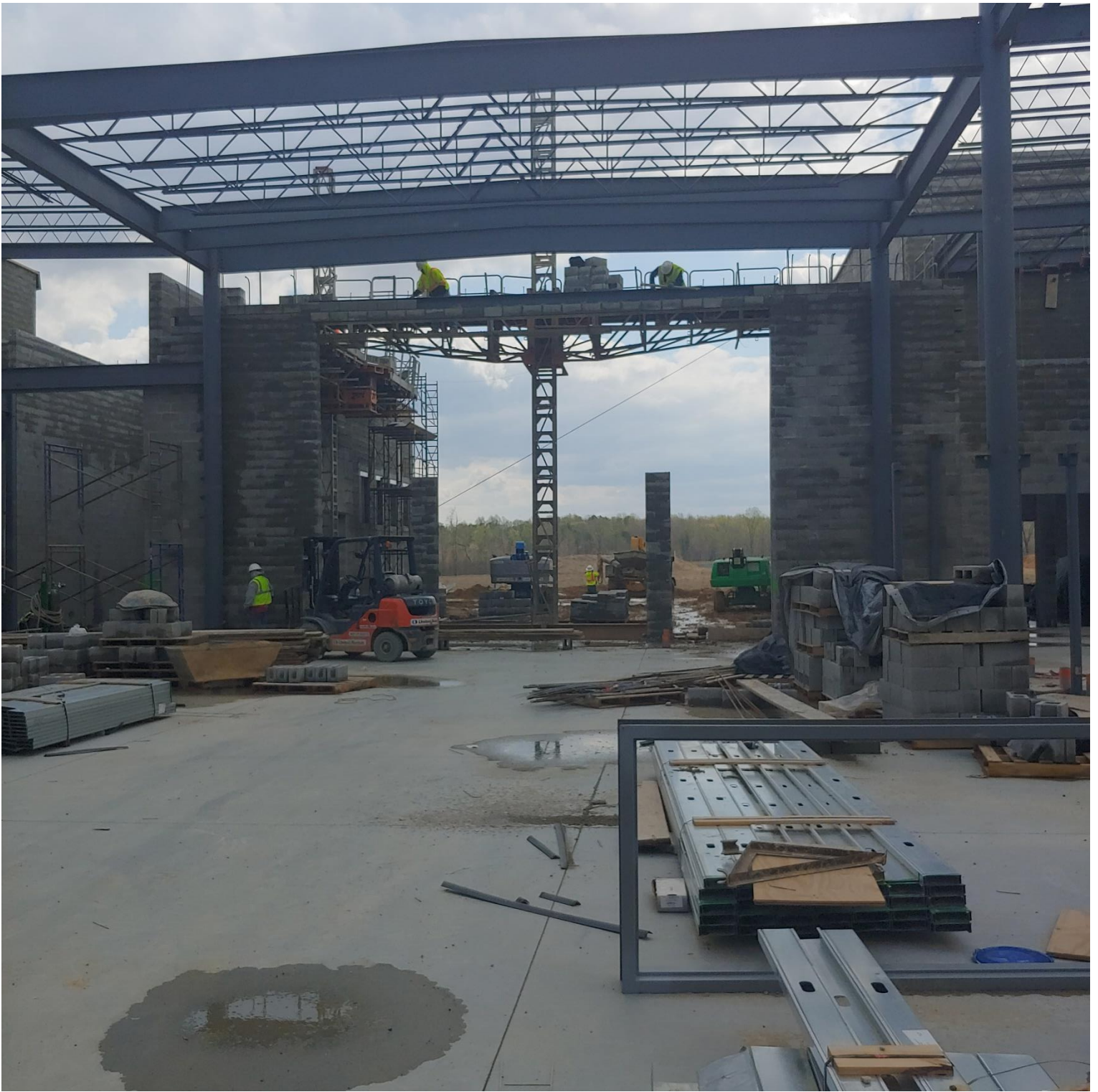
Photo 3 - Masons laying block above XC03 & XC04, Southside exterior wall of Area C
