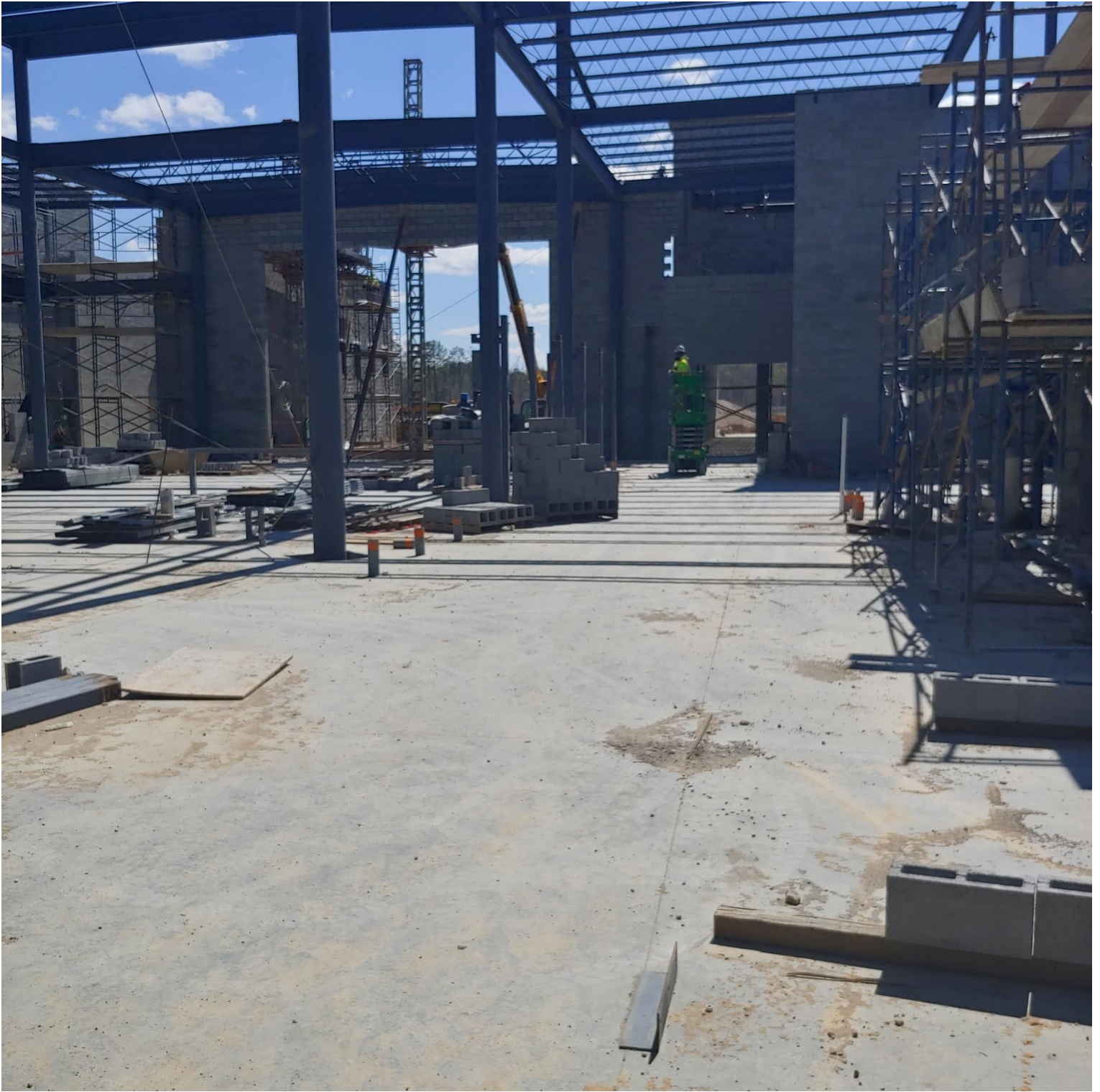
Photo 2 - Masons are finishing the blockwork on the South wall of Area C
