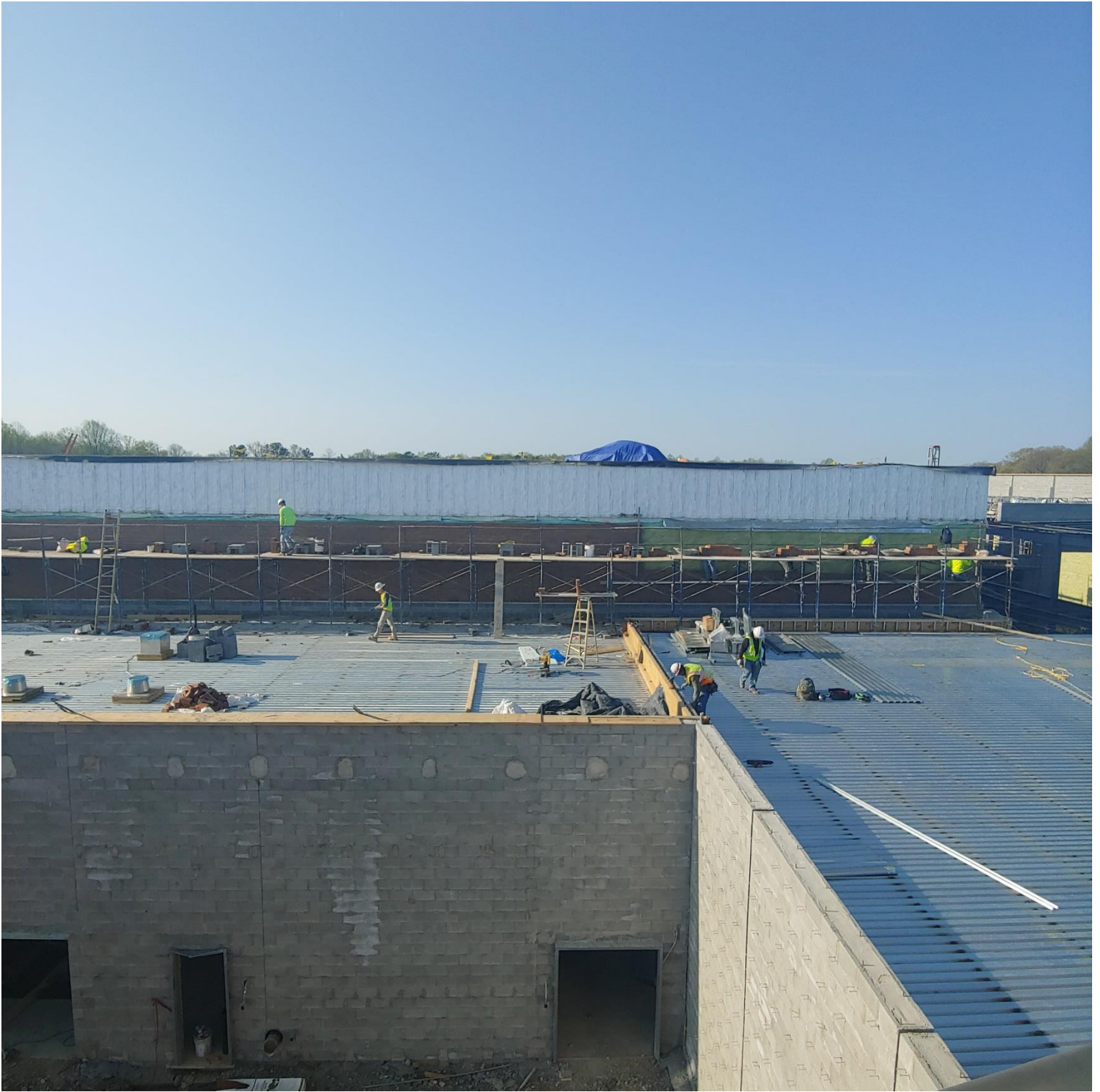
Photo 5- Brick being laid on the Northside of Area D and Parapet wall being constructed between Areas C & D..
