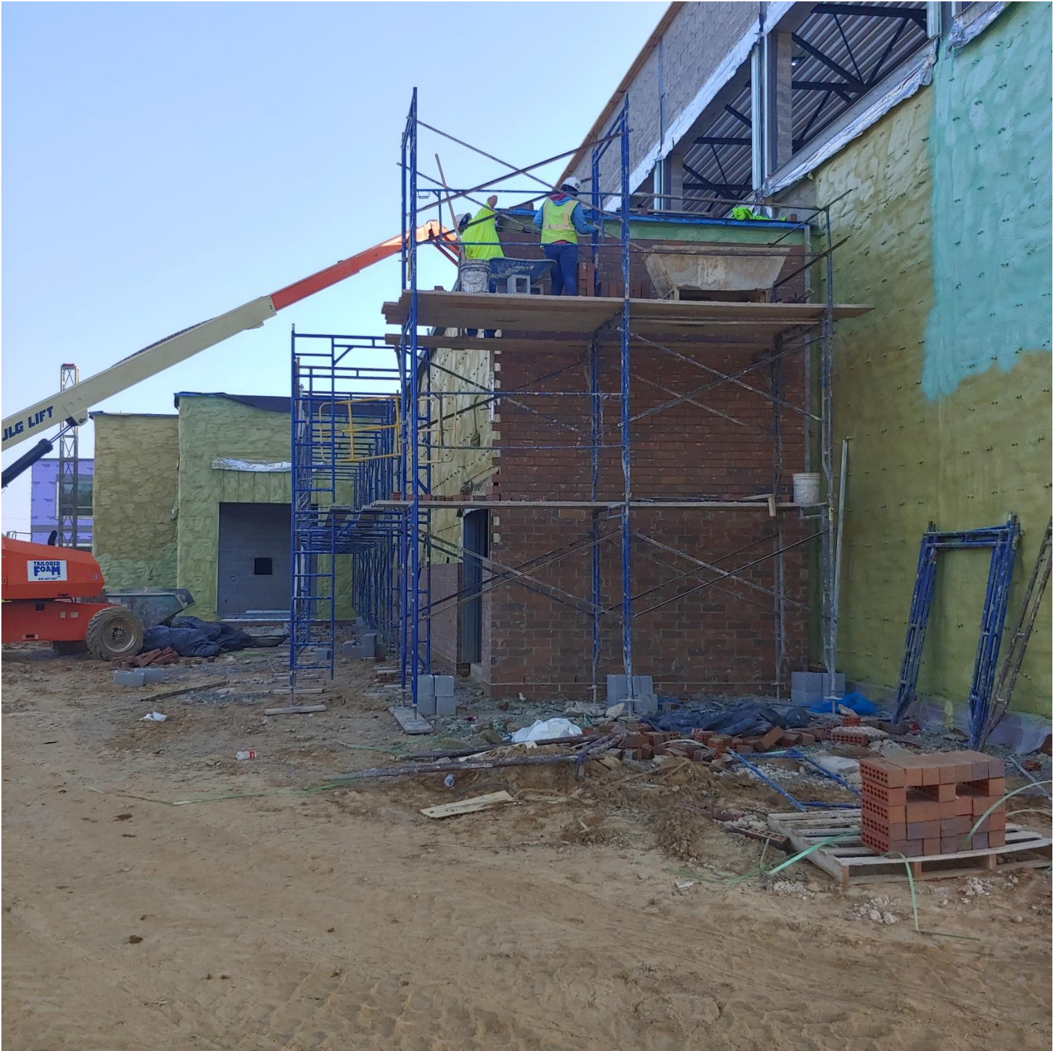
Photo 2 - Brick continues to be laid on the Southwest side of Area E
