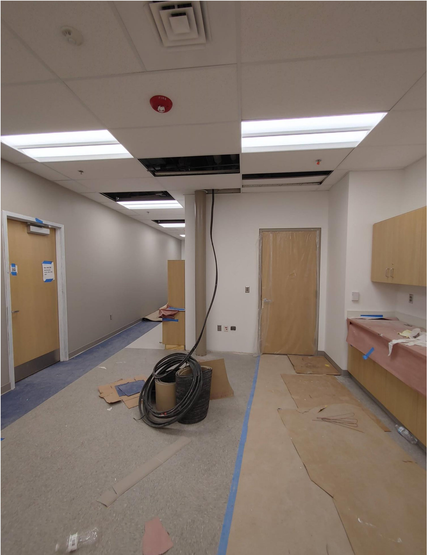
Photo 6 - Antenna Wire (Equipment scheduled to arrive in early June. Wire to be curled up in ceiling until equipment arrives).
