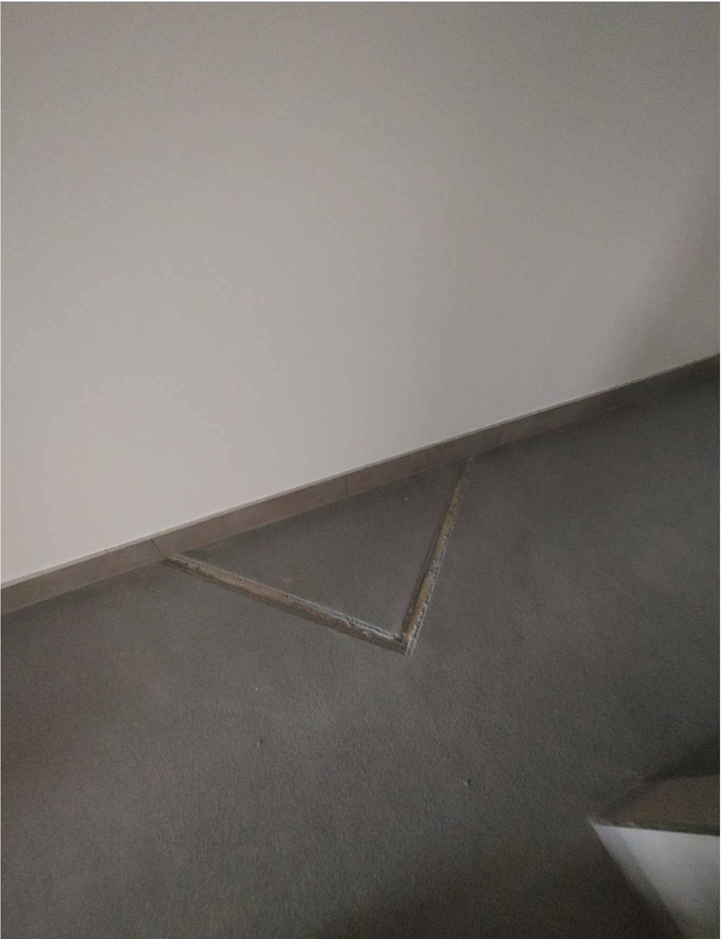
Photo 7 - Diamonds in Bathrooms. Brach says their Sub will fill Diamonds and skim coat entire floor so everything matches.
