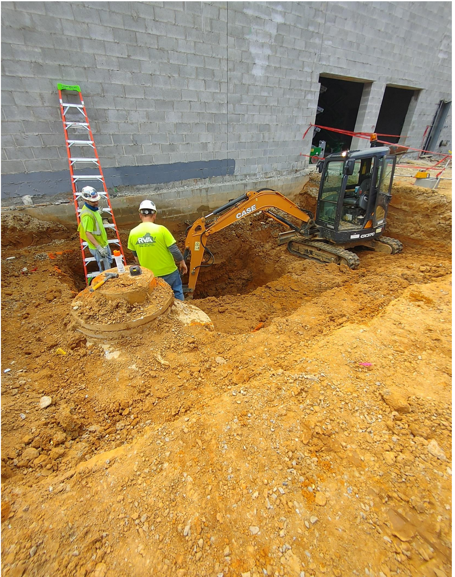
Photo 4 - Excavation has begun for Grease Trap on the Northside of Area D
