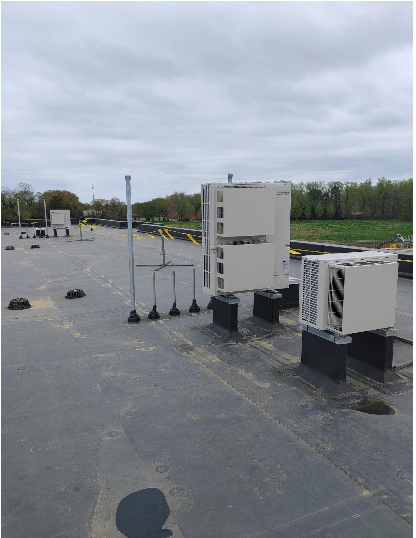
Photo 3 - HVAC Units set on the roof of Area A
