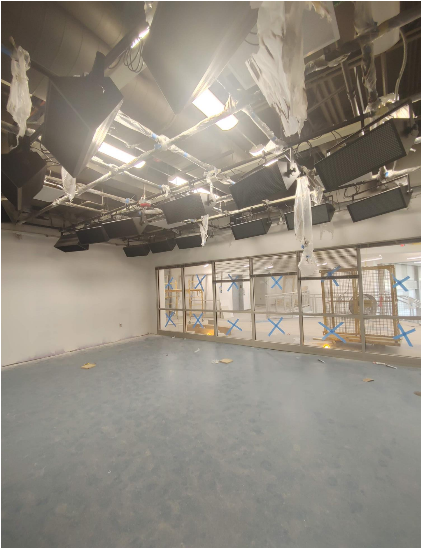
Photo 17 - Equipment installed in A221
