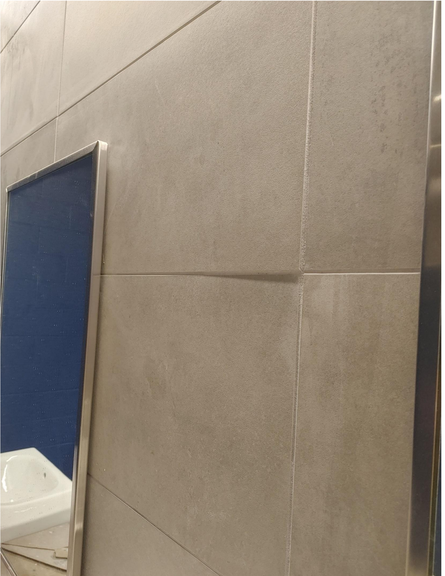
Photo 11 - Tile in Boys Toilet E103 – Several areas will need attention
