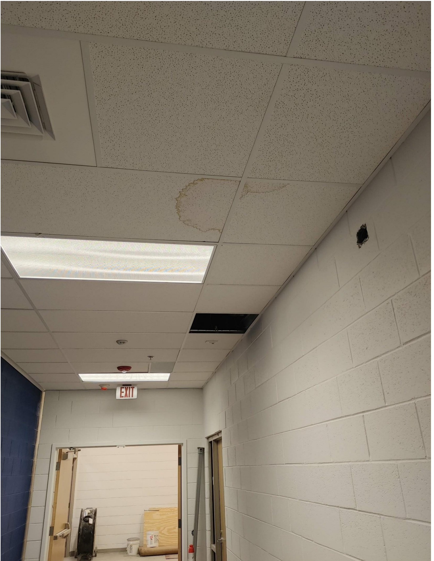
Photo 12 - Discolored Tile in Corridor E12
