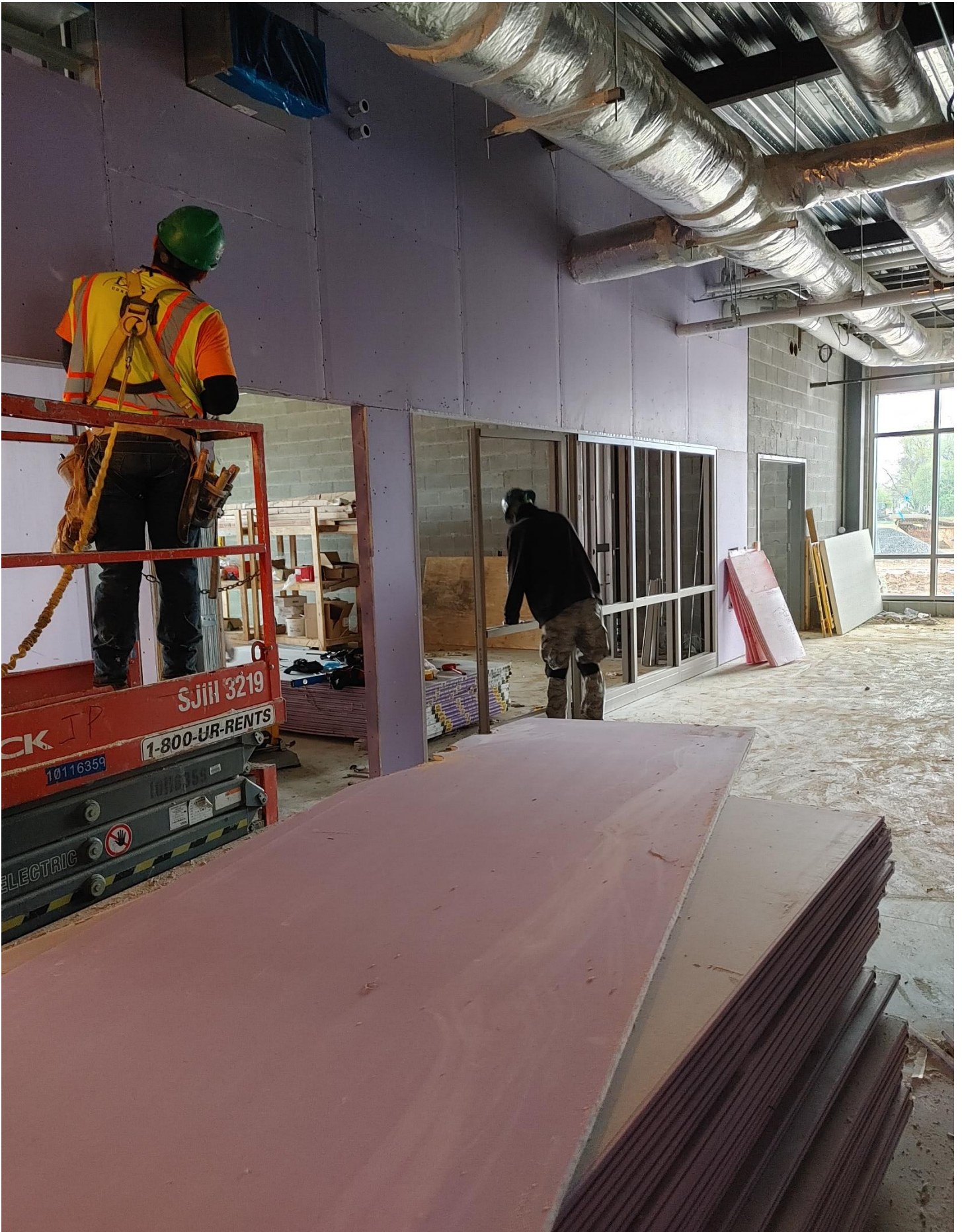
Photo 2 - Gyp Board being hung and the Glass frame being installed for Learning Studio A105 in Area A
