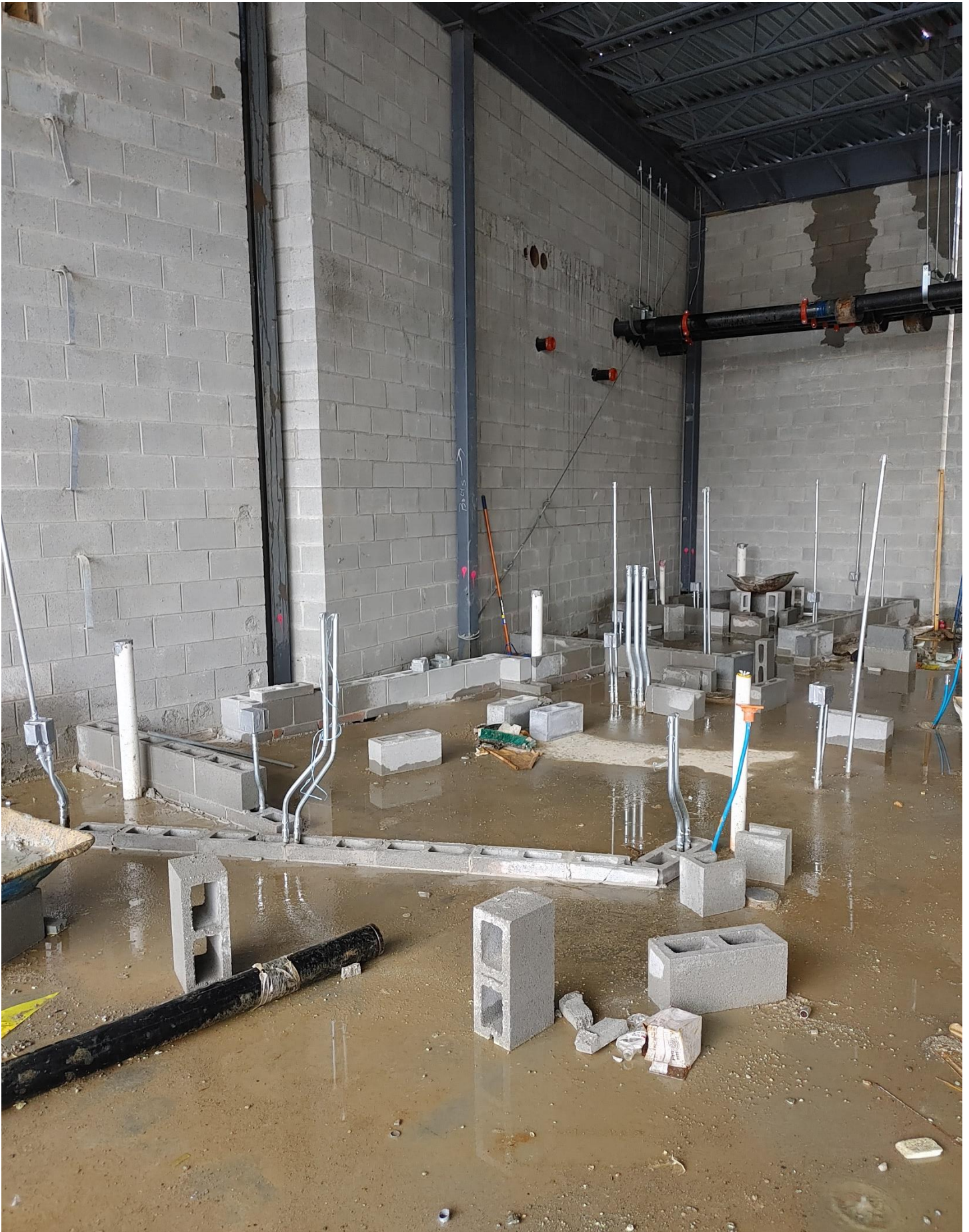
Photo 4 - Masons and Electricians laying block and running conduit in rooms C103, C104A & C104B Kitchen Area
