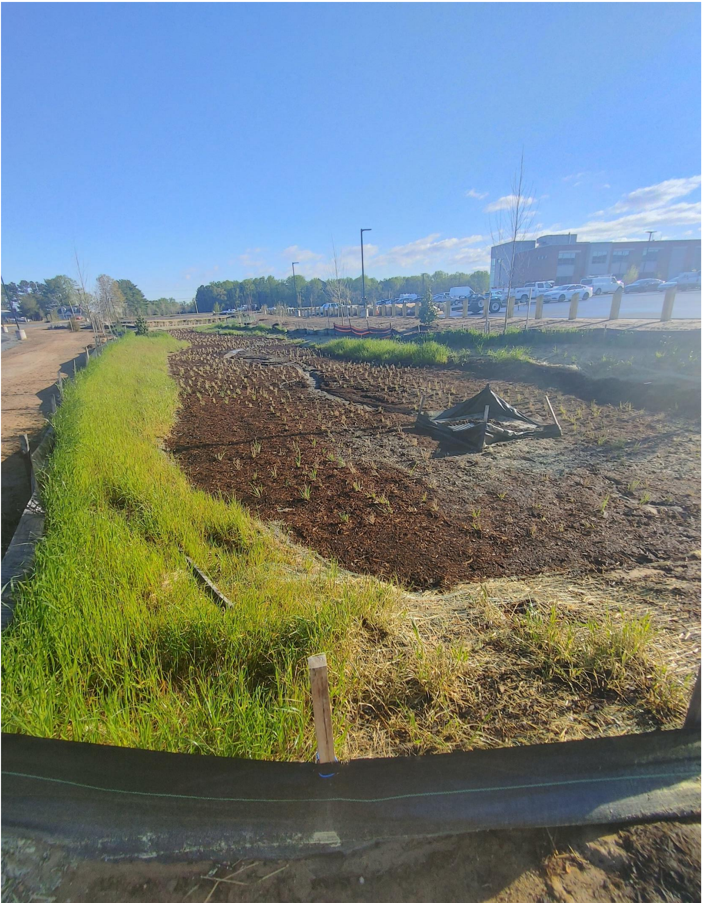
Photo 4 - Taken 4/19/2022 - Inlet Protection Failed.
