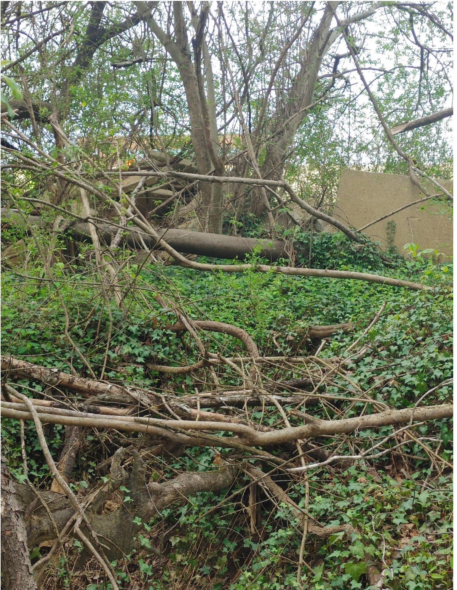
Photo 9 - Concrete is piled up in Spillway of Farmer's Property
