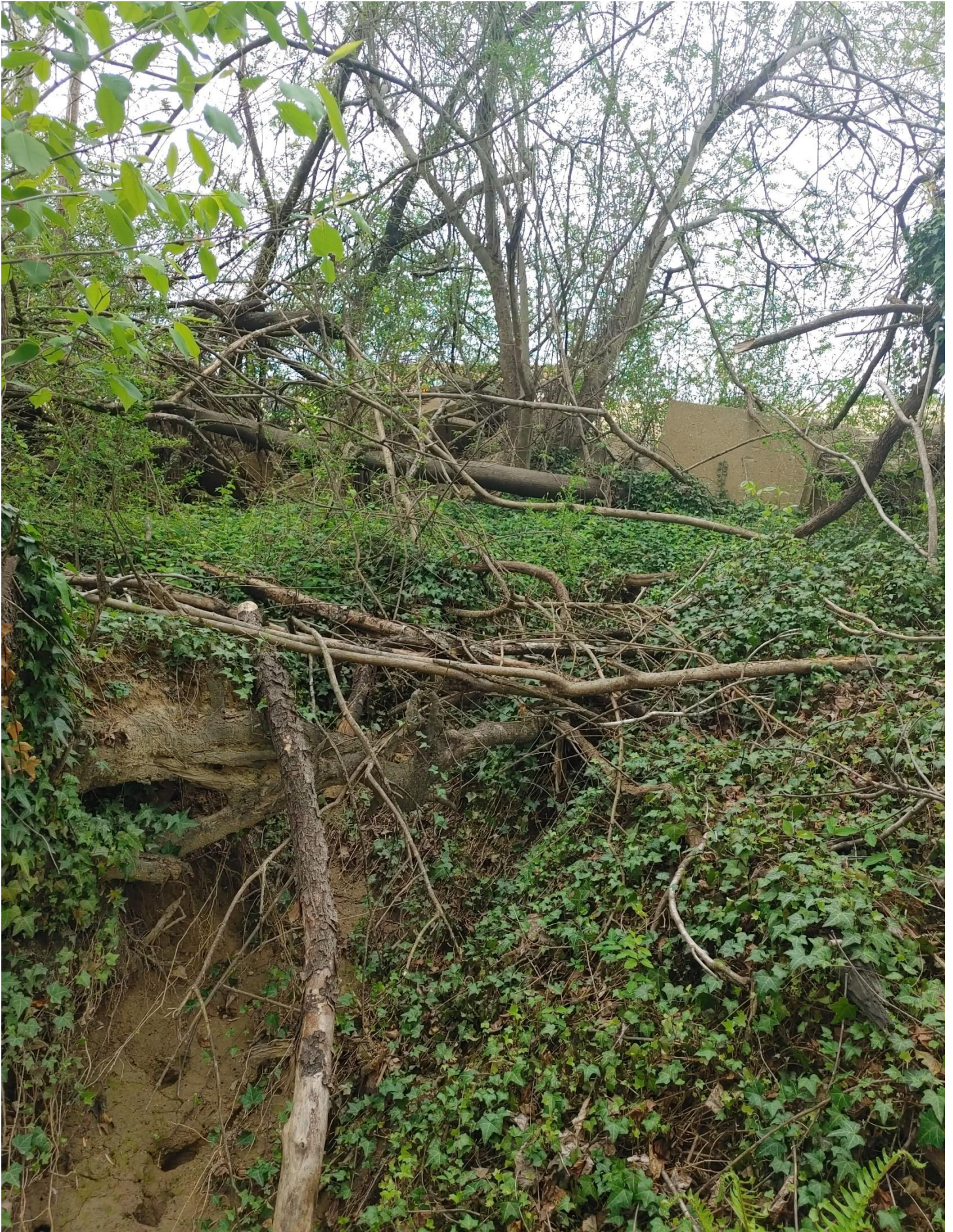
Photo 8 - Concrete blocking Spillway on Farmers Property
