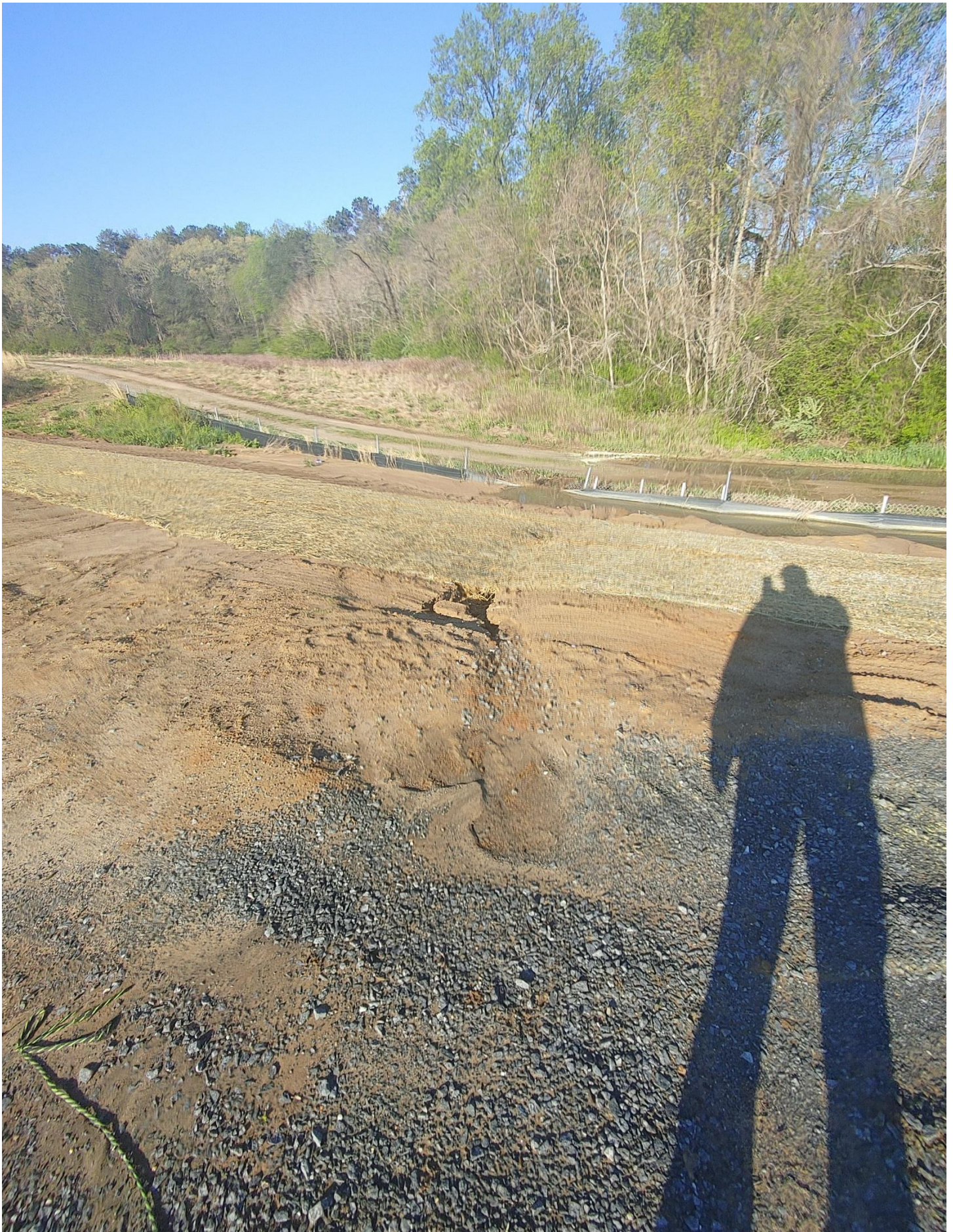
Photo 2 - Super Silt Fence Failed - Taken 4/19/2022
