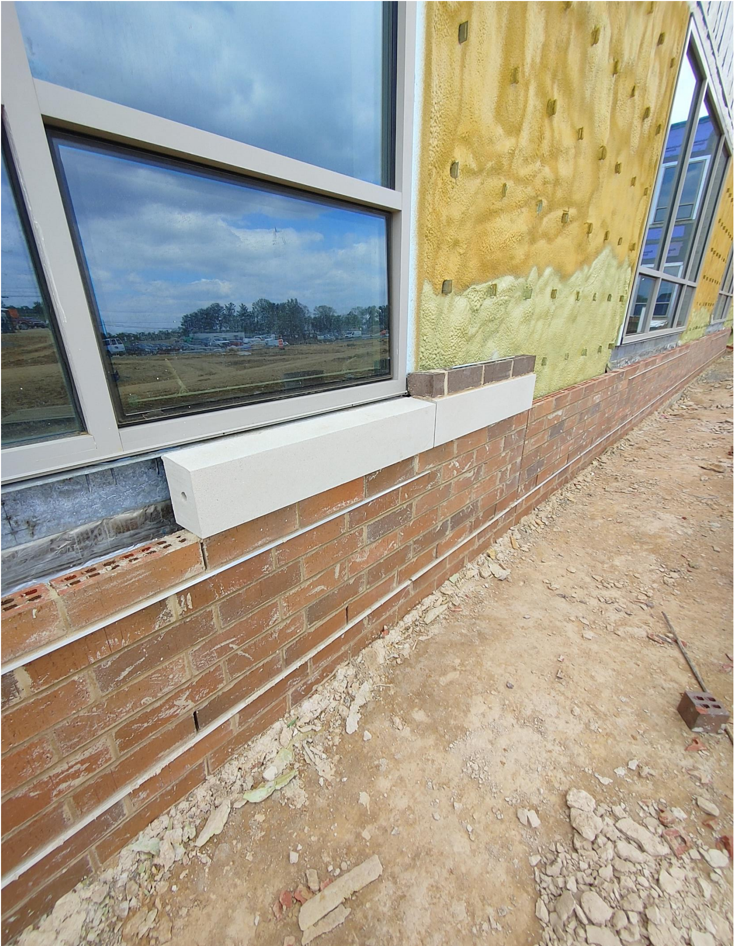
Photo 2 - Brick being laid on the Northside of Area A. Flashing is in place and weep holes are open.
