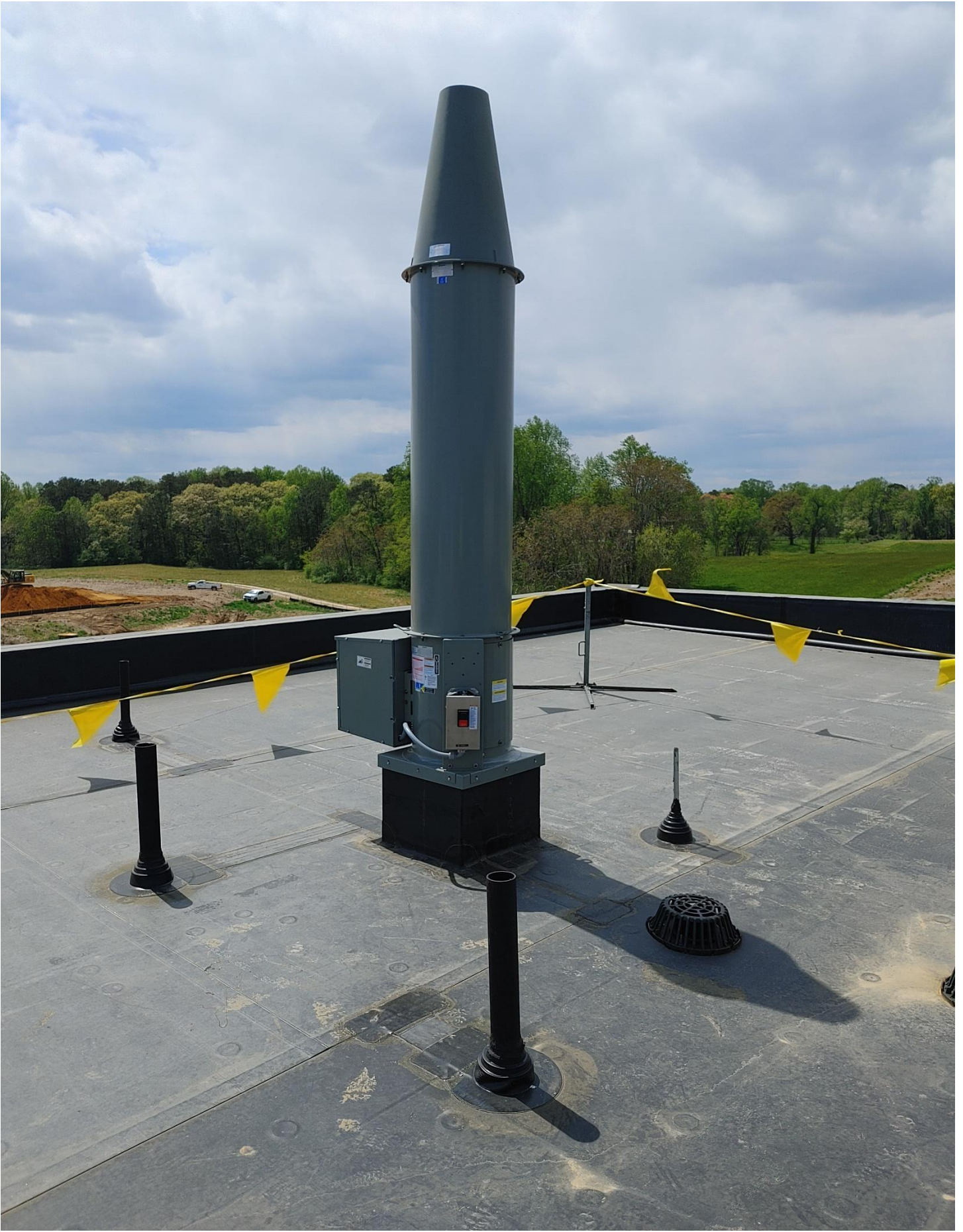
Photo 12 – Fume Hood has been installed Area B
