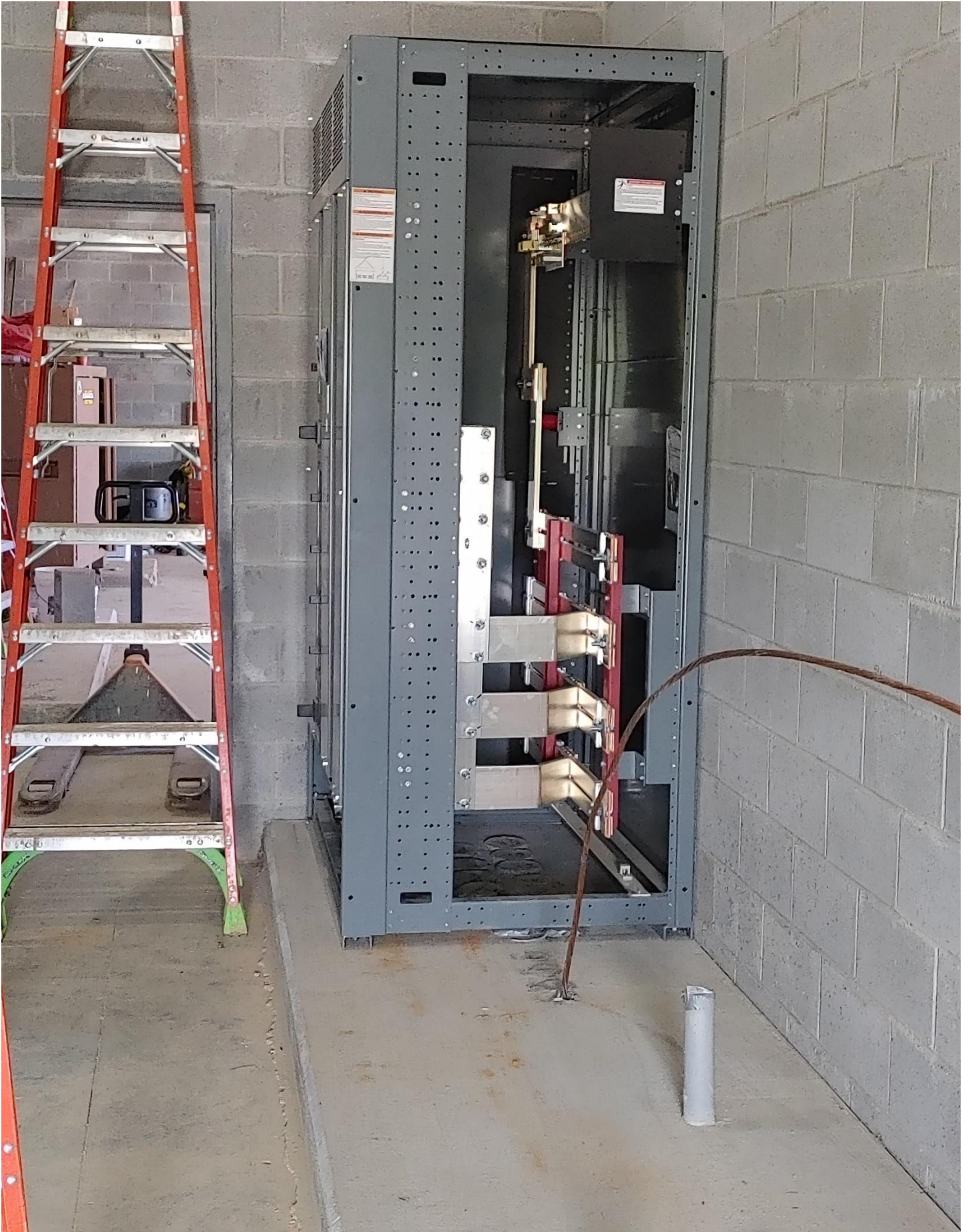
Photo 7 - Hazzard Electric has set one of the Switch Gears in the Electrical Room, Area D.
