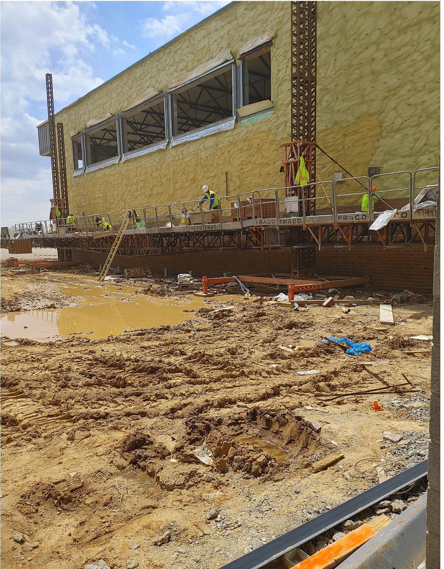
Photo 8 - The Masons are laying Brick on the East side of Area E
