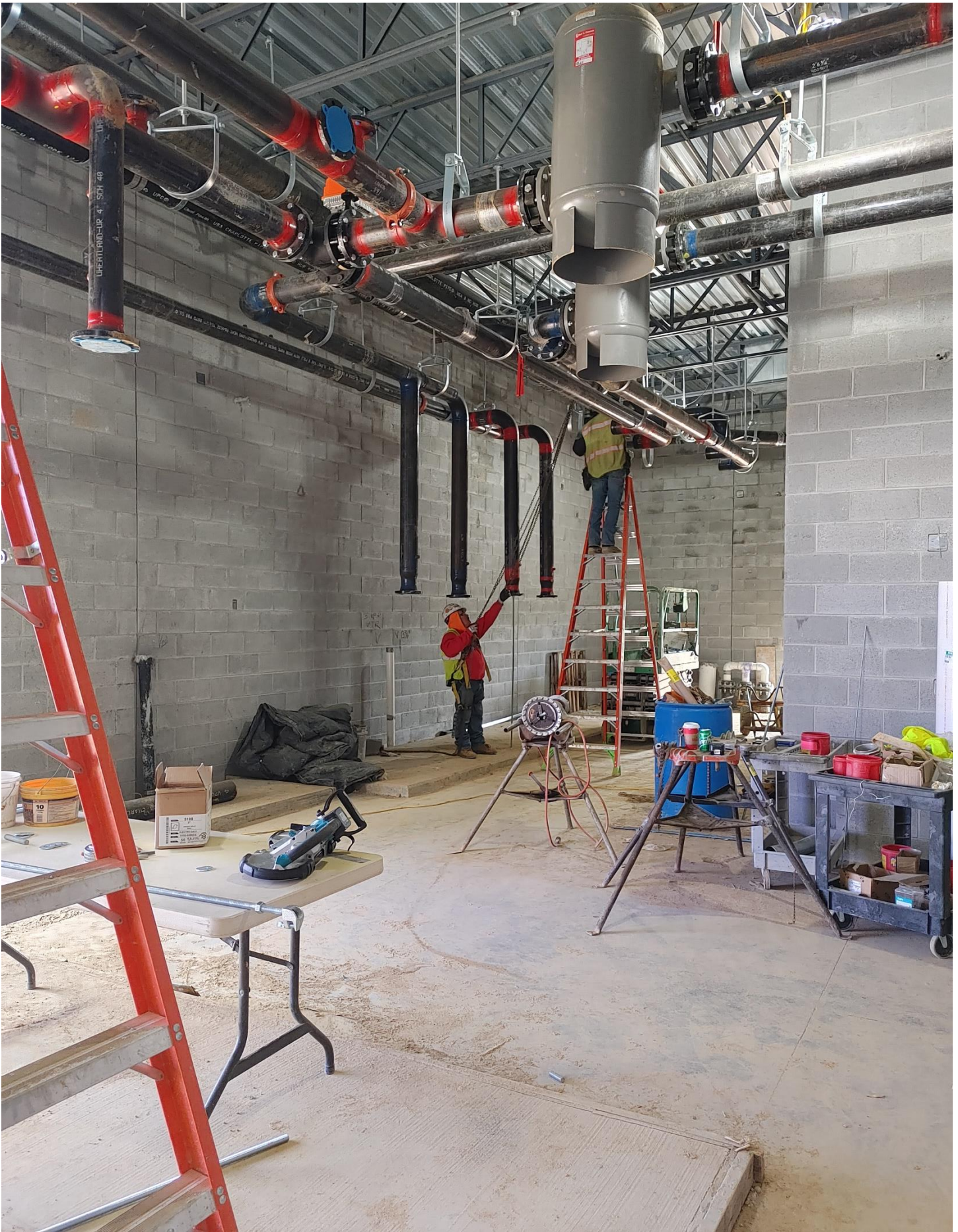
Photo 5 - Colonial Web running pipe in the Mechanical room, Area D.
