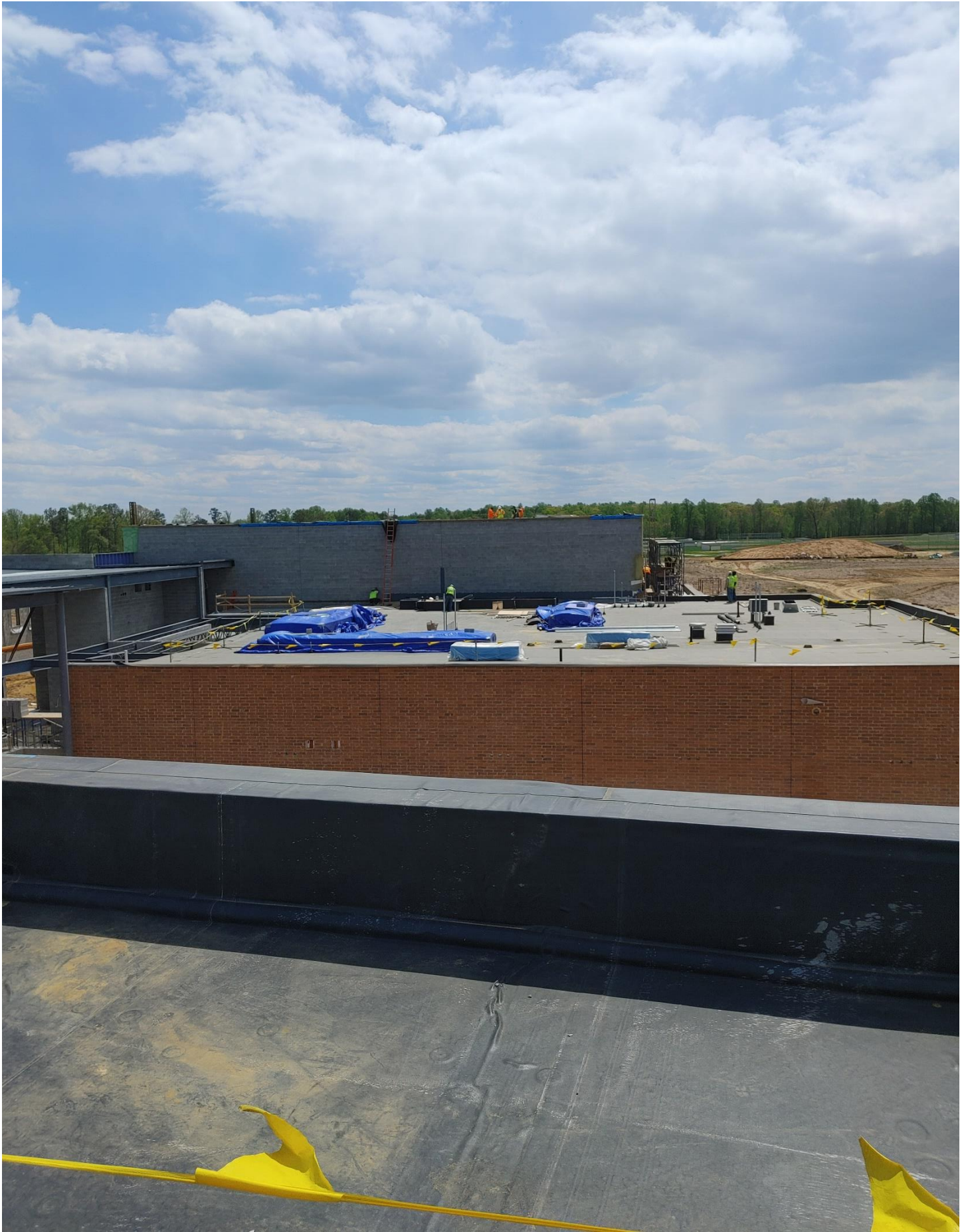
Photo 13 -Roofers are working on the high roof of Area E and the area between the high and low roof is being flashed.
