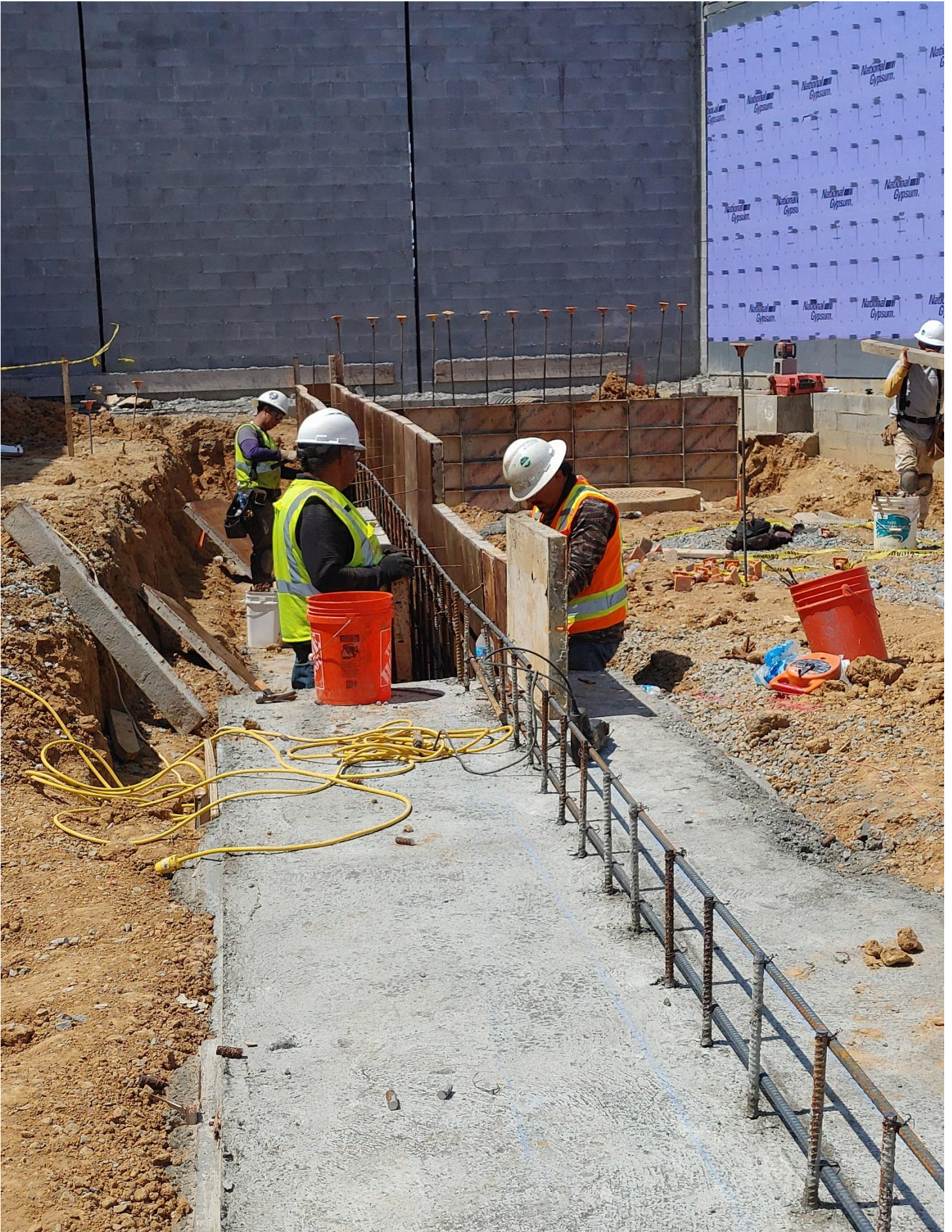
Photo 6 - Industrial Concrete is setting Metal Forms for the Loading Dock Retaining Wall.
