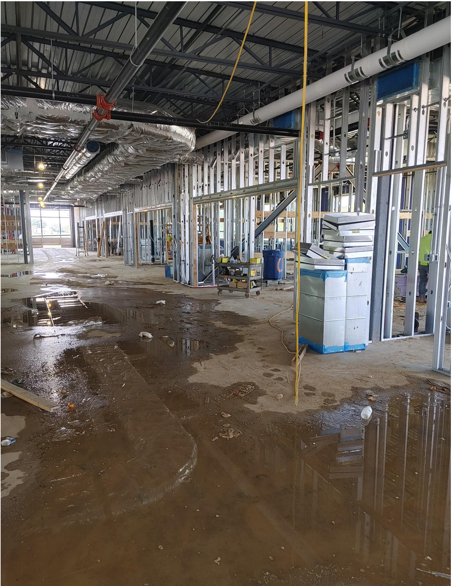
Photo 11 - Storefront Rough openings are being furred out with plywood for anchoring purposes in Area B.
