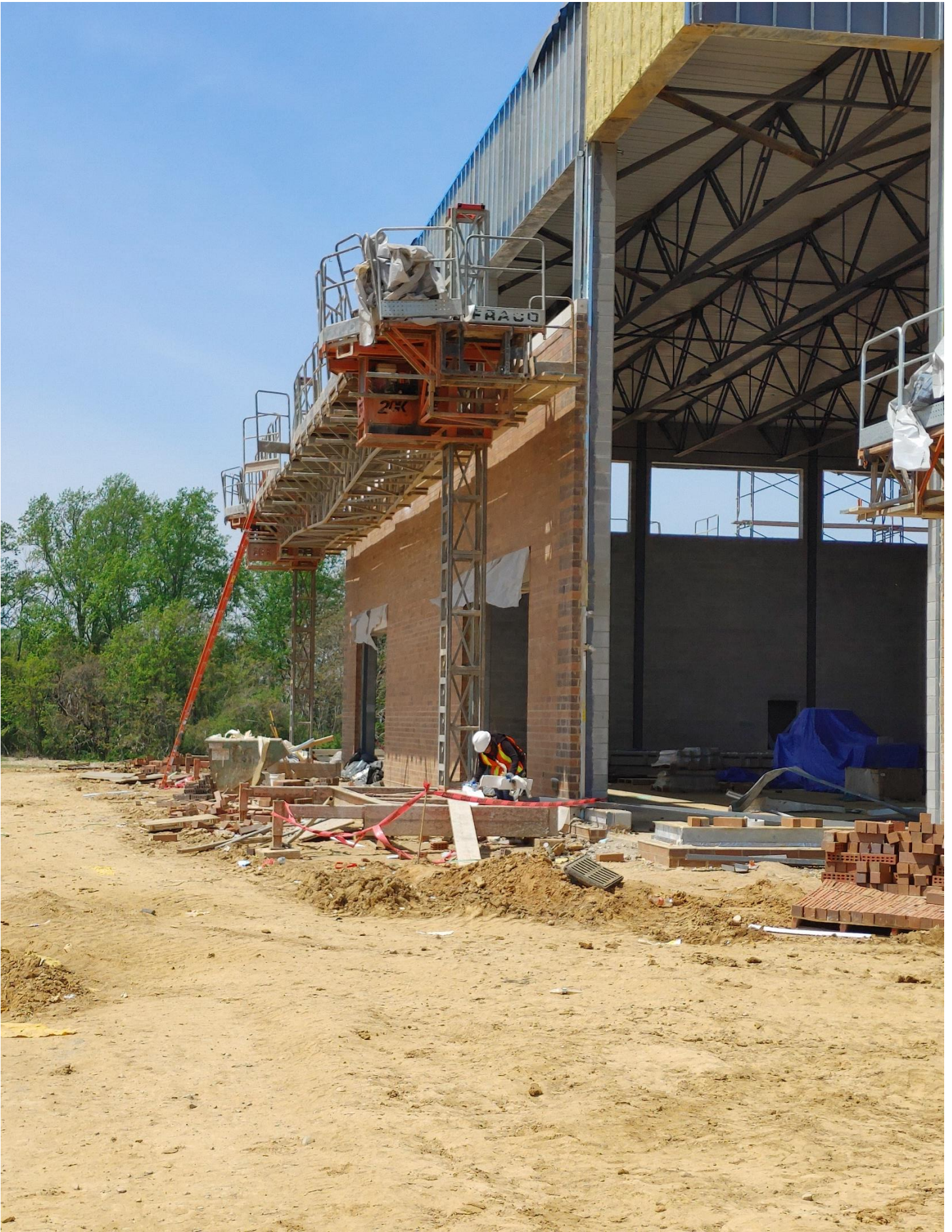
Photo 4 - Pre Cast has been set under the windows of the Gym on the South side.
