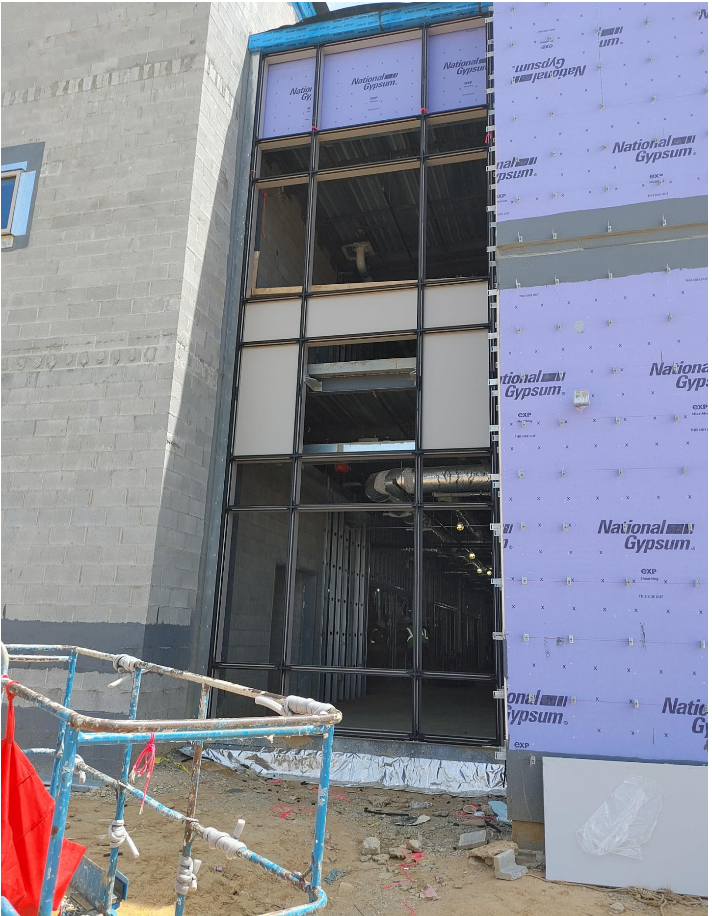
Photo 1 - FM&G continues to work on the Curtain Wall on the West side of Area B
