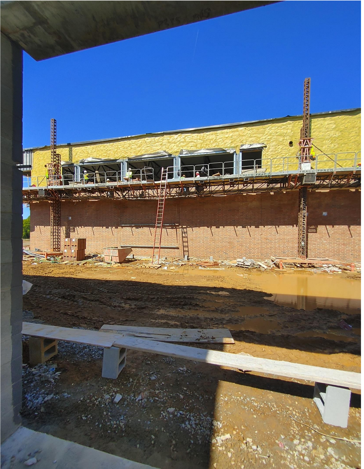
Photo 2 - J. D. Long are laying Brick on the East side of Area E.
