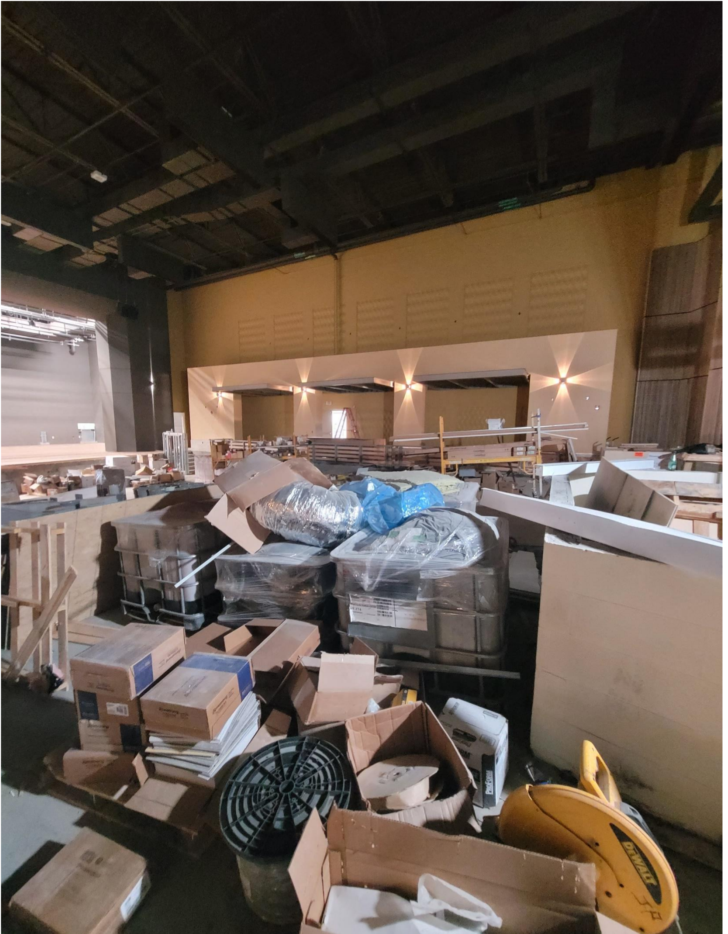
Photo 5 - Side wall lighting has been installed in Auditorium
