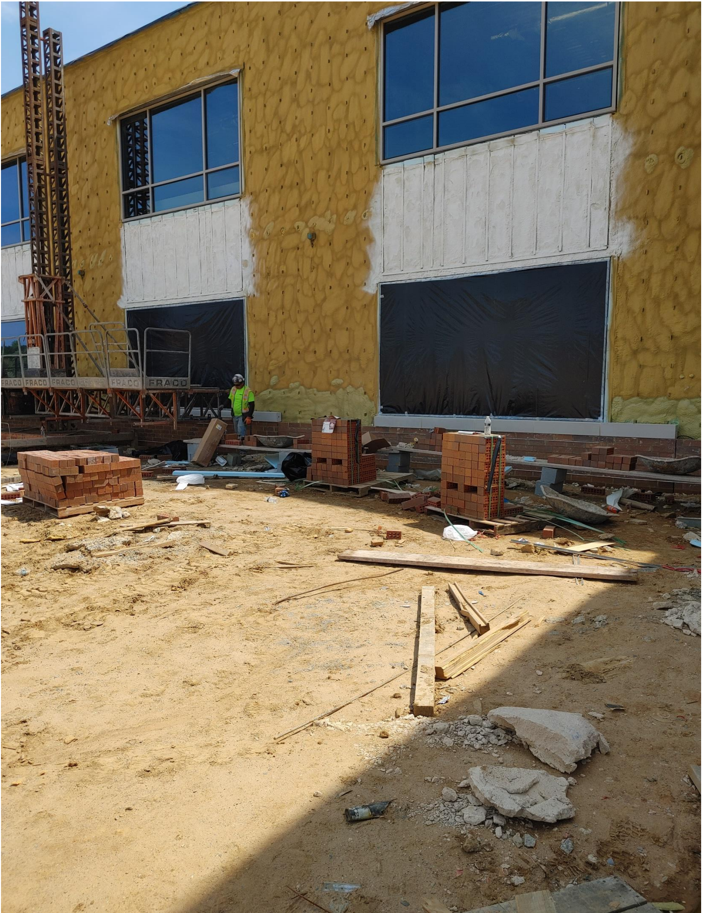
Photo 8 - Poly being placed over glass and frames to protect them when Brick is laid.
