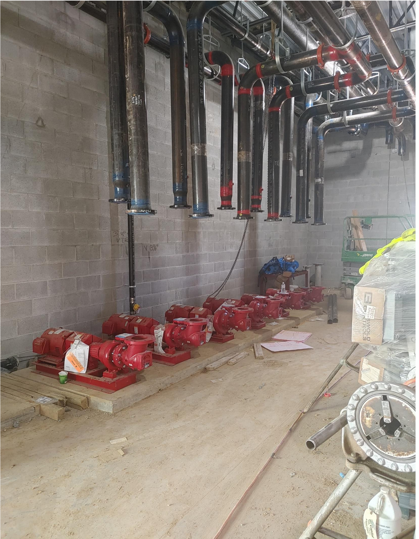
Photo 3 - Circulating Pumps set in Area D
