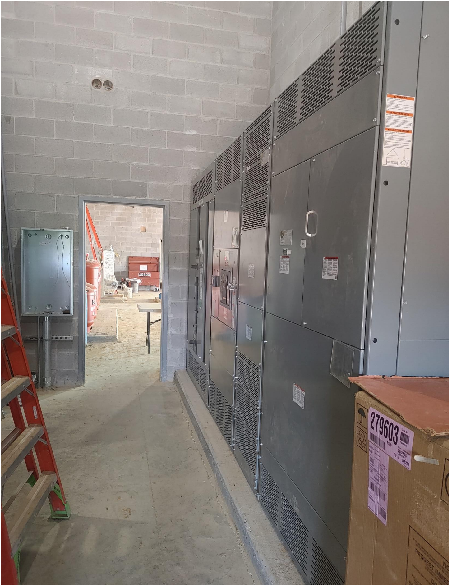
Photo 5 - Switch Gears in the Electrical Room of Area D
