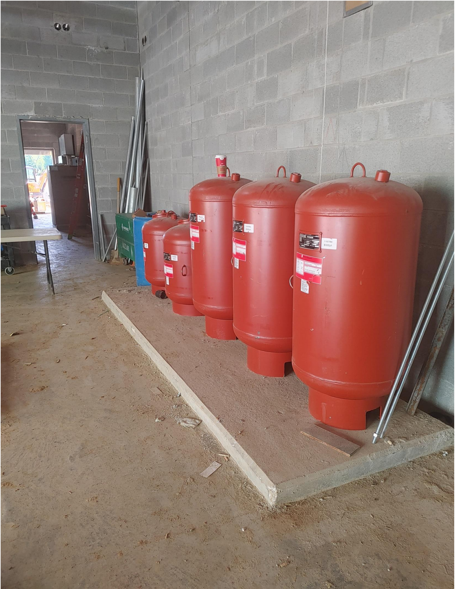
Photo 4 - Expansion Tanks Set in Area D
