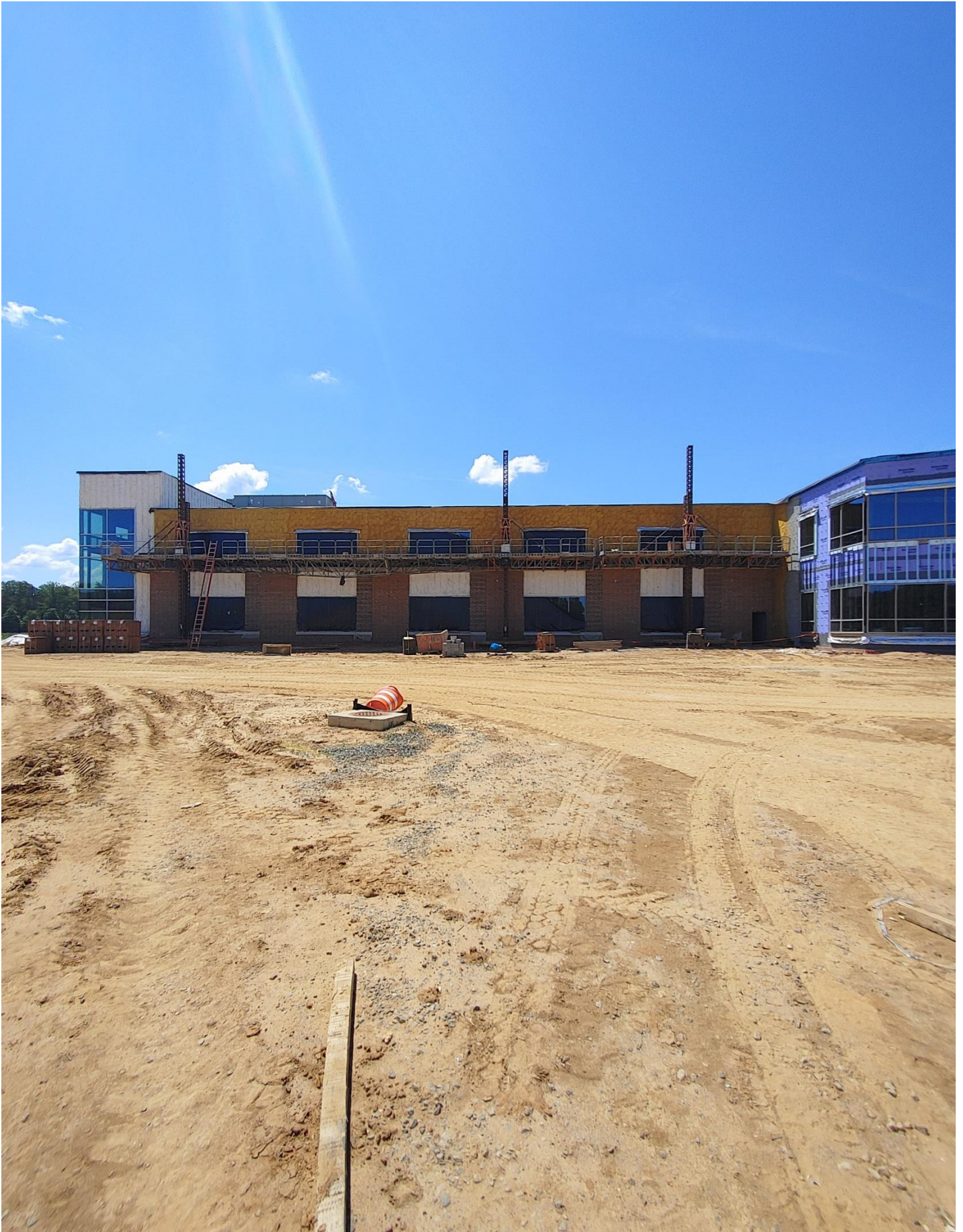
Photo 1 - Brick continues to be laid on the North side of Area A
