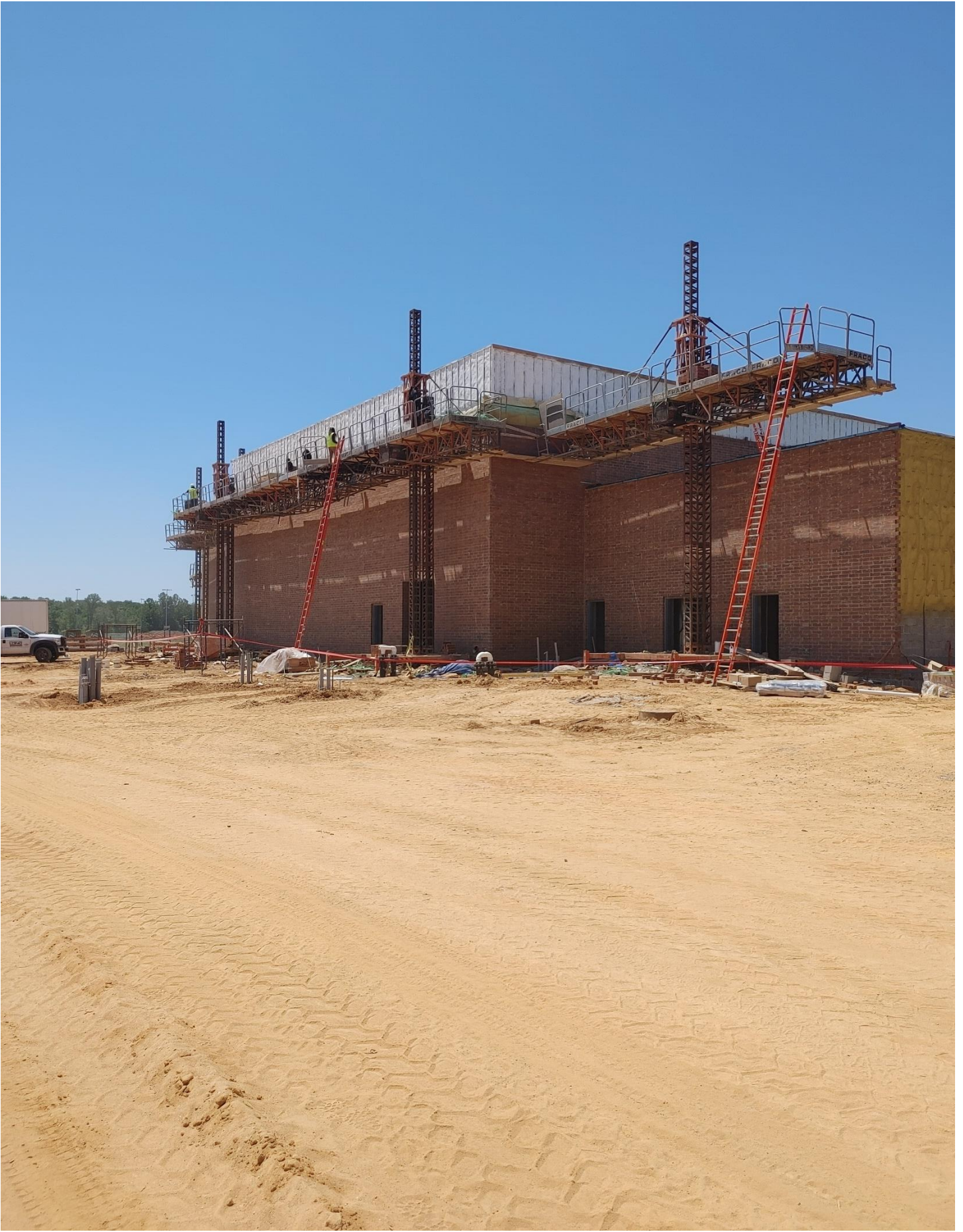
Photo 1 - Brick continues to be laid on the East side of Area D
