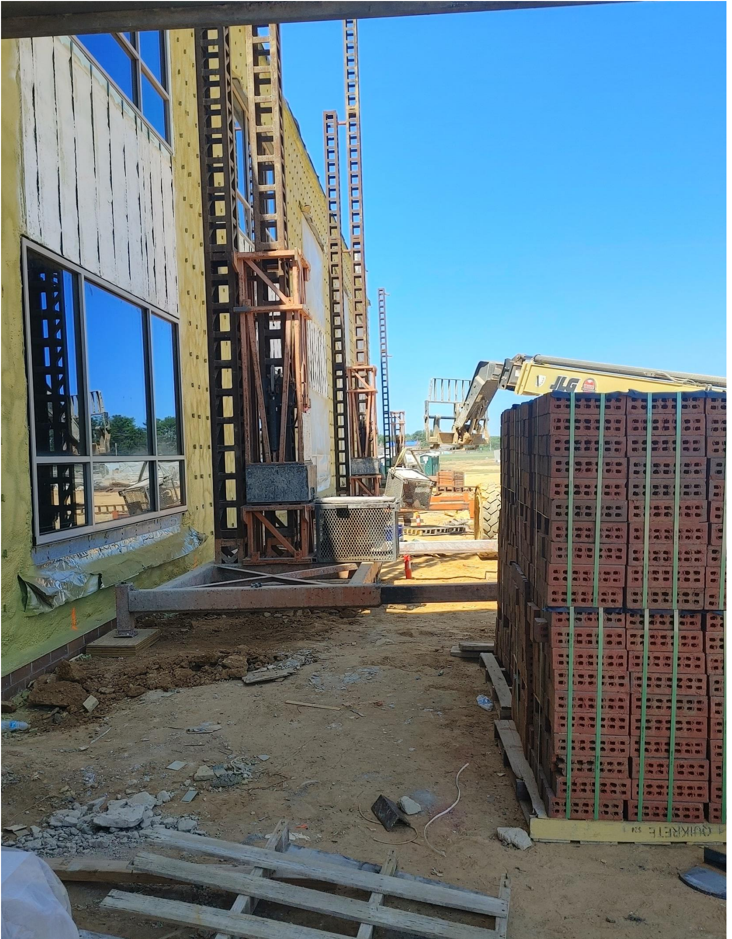
Photo 2 - Fraco Scaffolding is being erected on the North side of Area B
