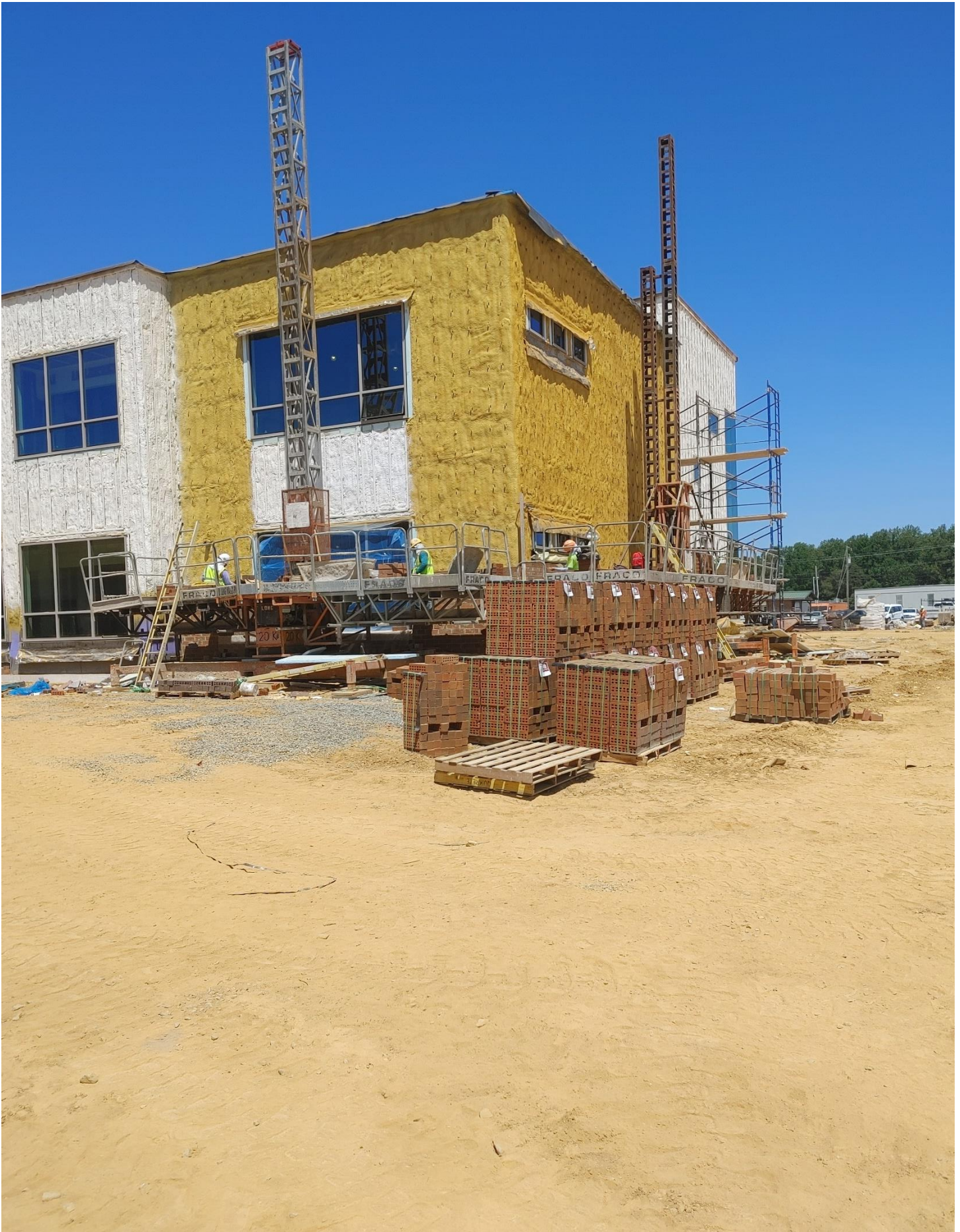
Photo 6 - Brick being laid on the South and East side of Area A
