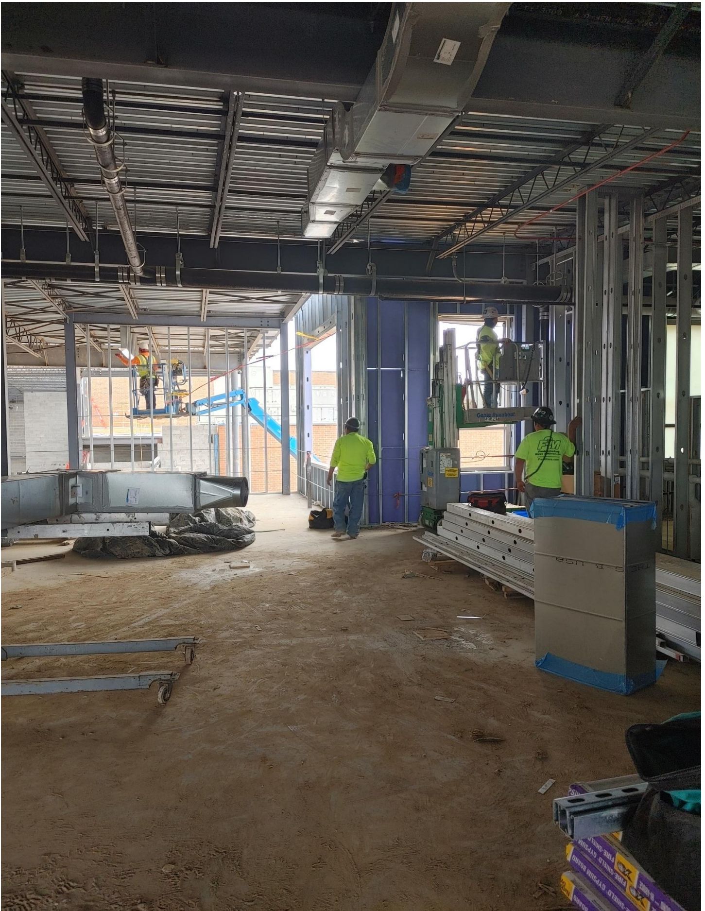
Photo 8 - Glass being installed in Area B and Framing of Metal Studs in Area C, background.
