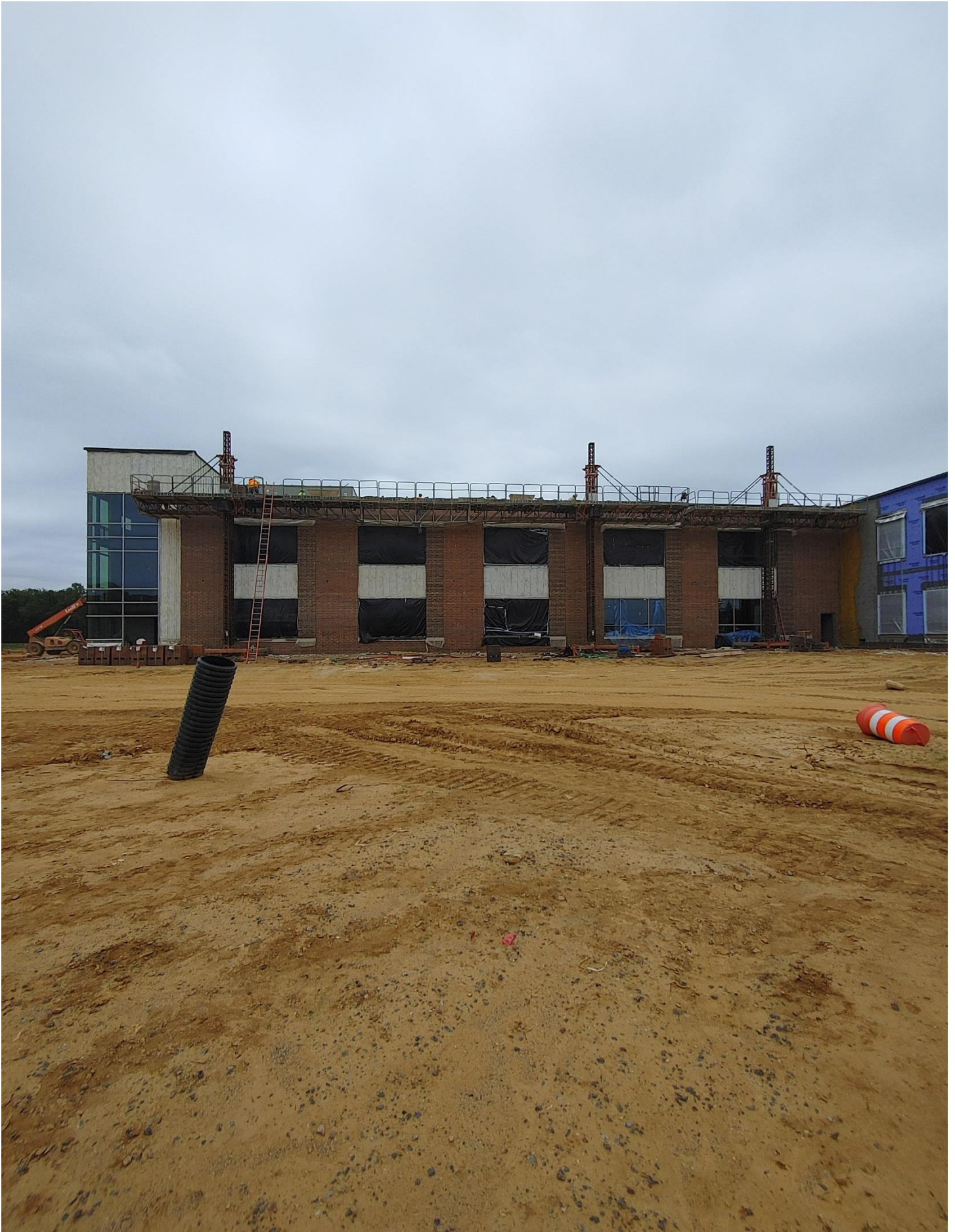
Photo 1 - Masons continue to lay Brick on the North side of Area A
