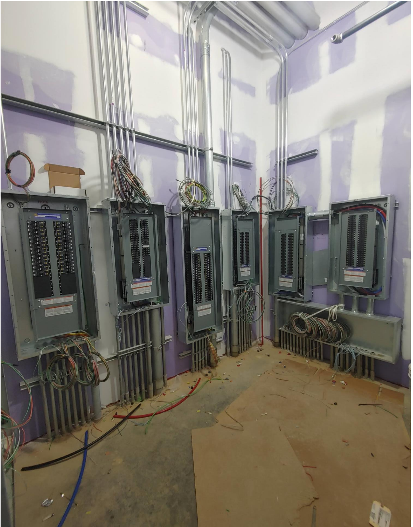
Photo 5 - Electrical Panels have been installed on the 1st Floor of Area A, A113.
