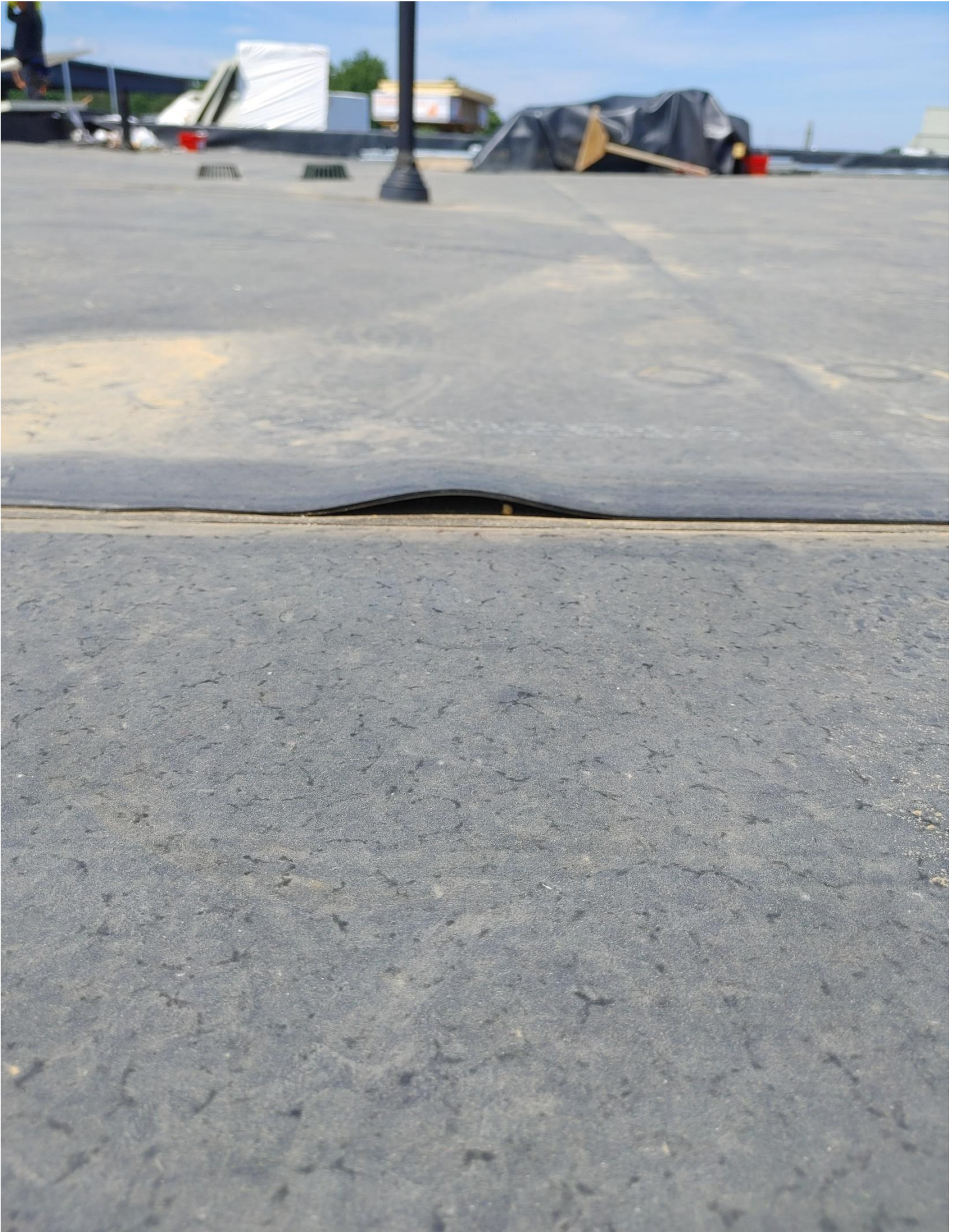
Photo 5 - A small section of the roof membrane overlap joint did not adhere properly on the roof of Area A.
