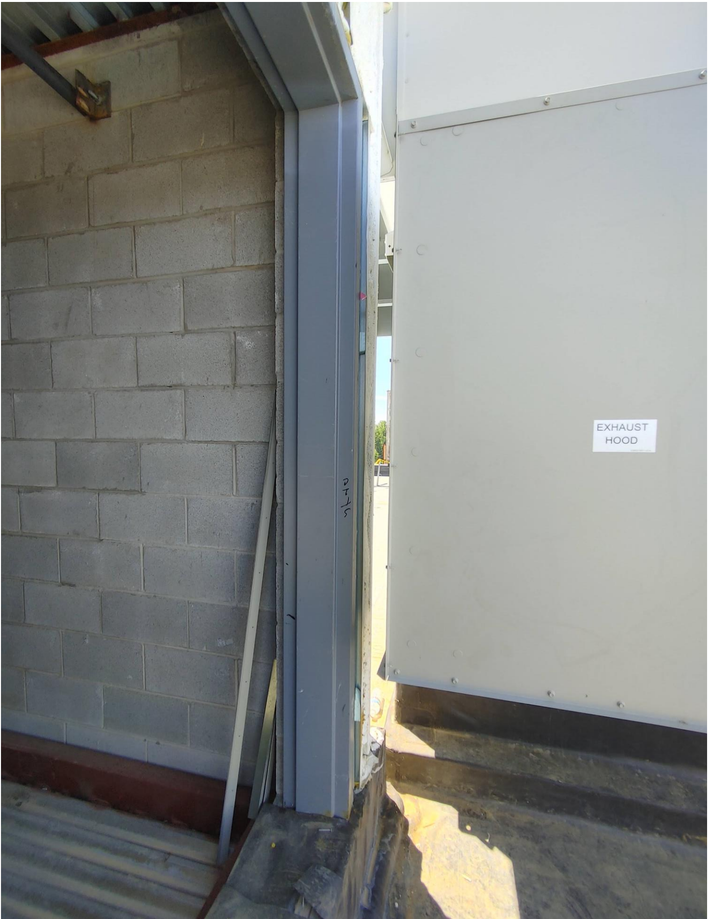
Photo 4 - HVAC Unit on the roof of Area A sits close to door frame.
