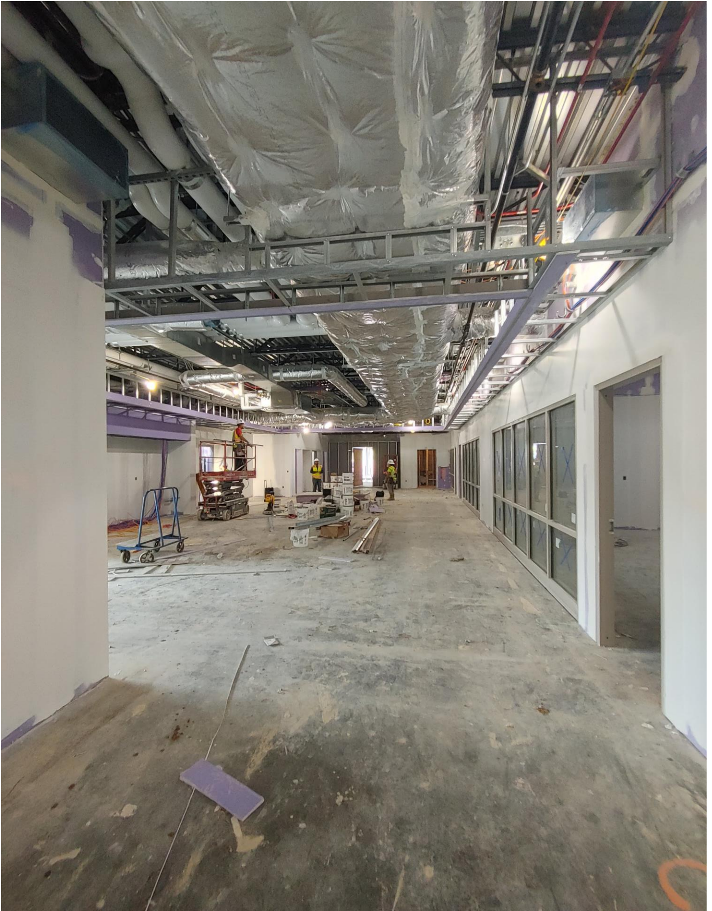
Photo 3 - Bulk Head is being framed on the 1st floor of Area A.
