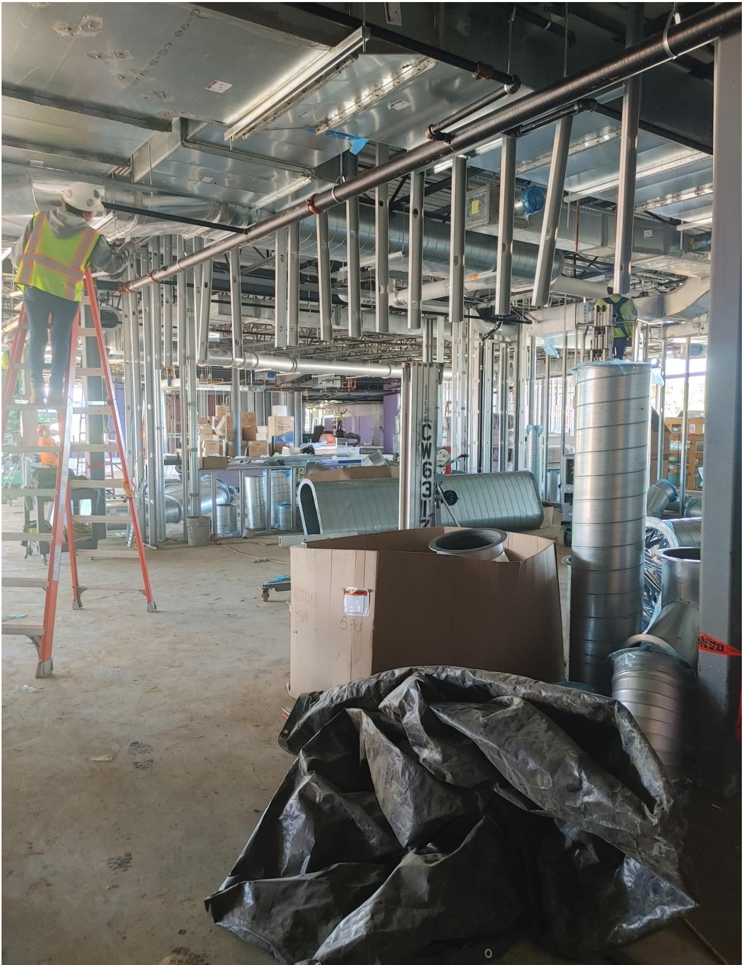
Photo 6 - Duct work is being sealed in the Administrative area of Area A.
