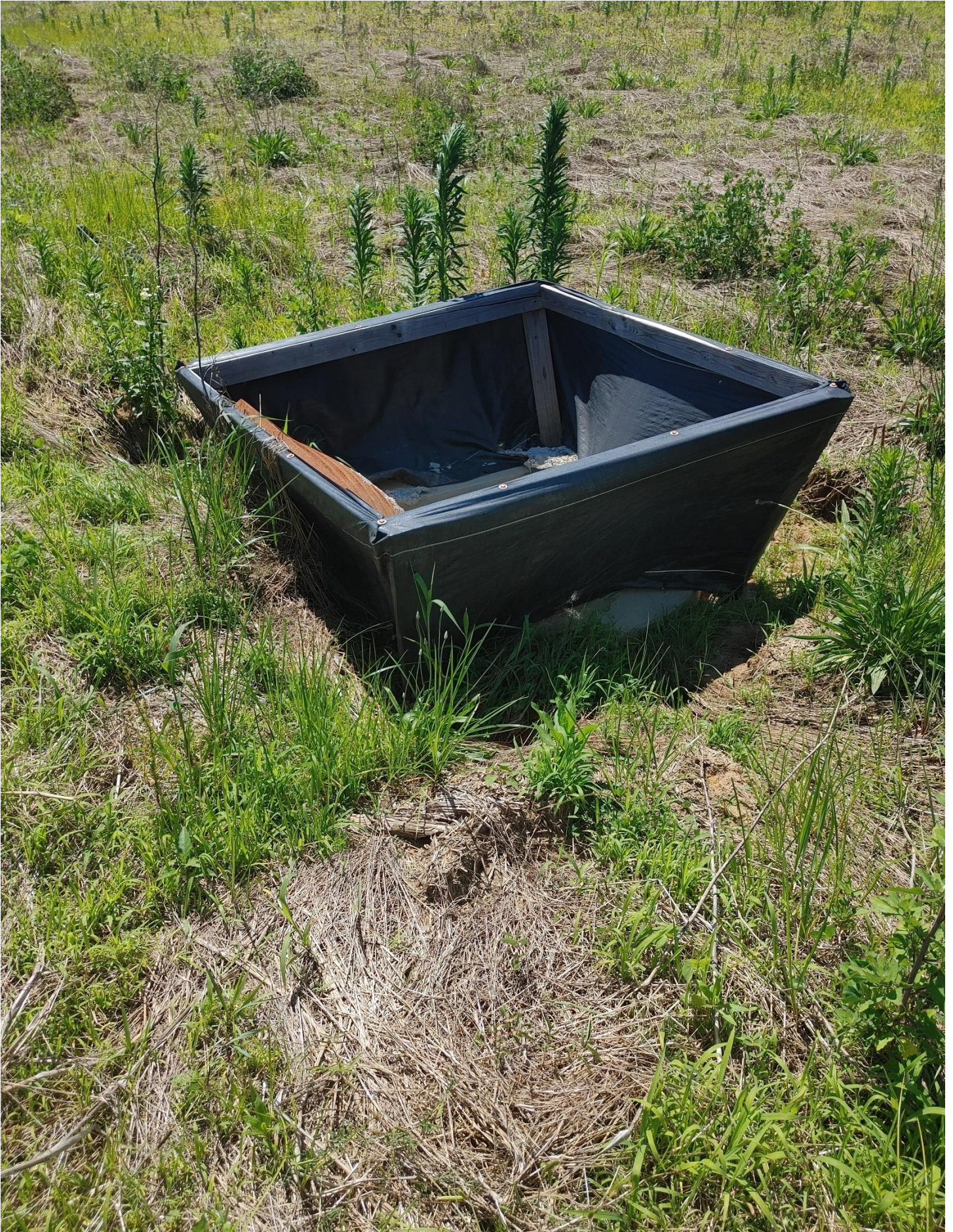
Photo 11 - Inlet protection needs attention.
