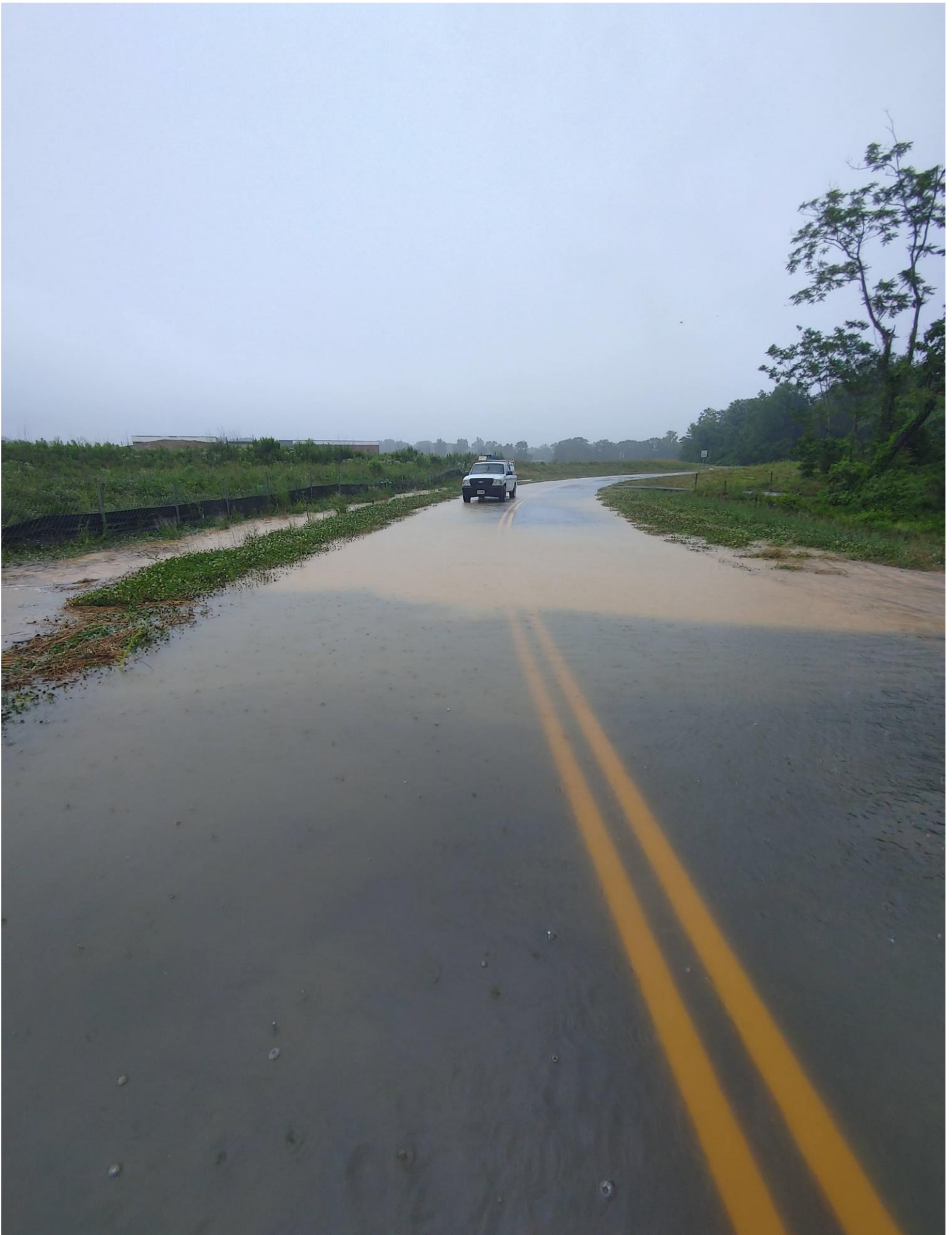
Photo 2 - Water sheeting across County Park Road. Drop inlet unable to handle volume of water overflowing from Retention Pond.
