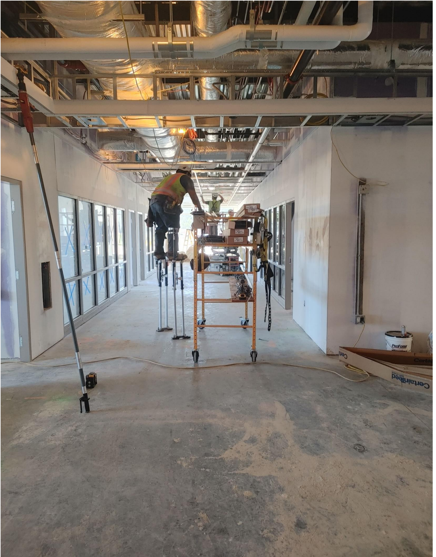
Photo 8 - Ceiling Grid is being run on the 1 st floor of Area A.
