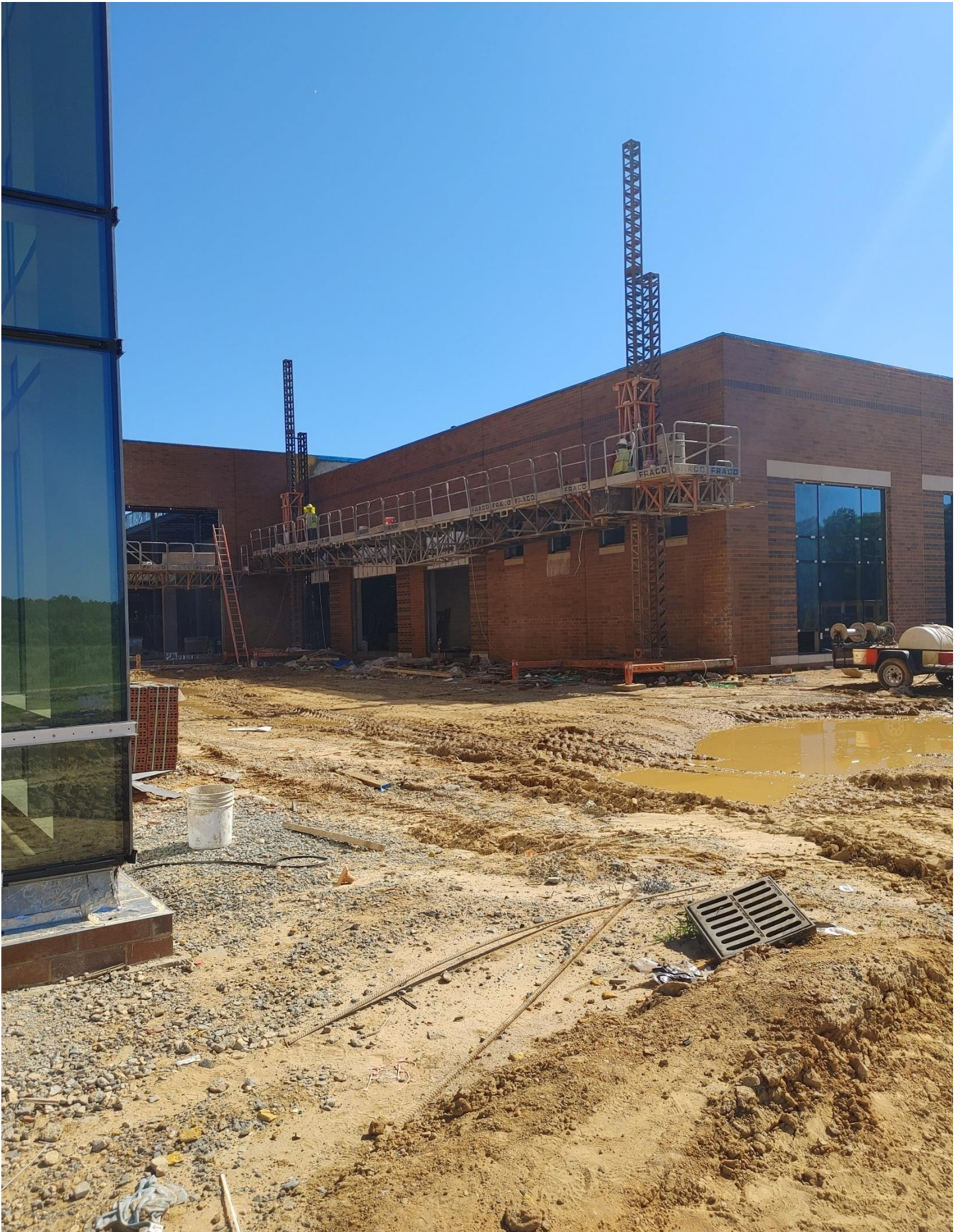
Photo 2 - Brick is being power washed on the West side of Area D.
