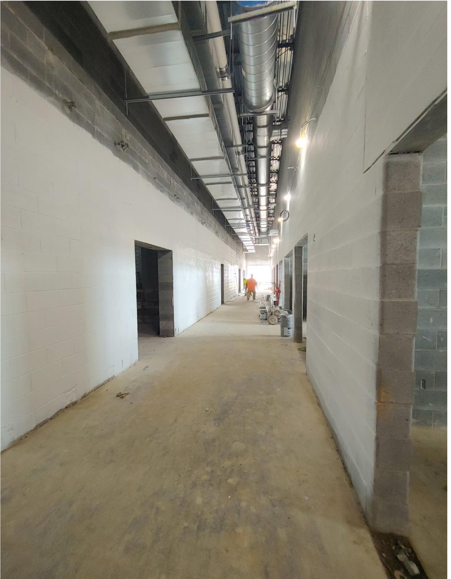
Photo 3 - Block Filler is being sprayed and rolled on walls in Area D.
