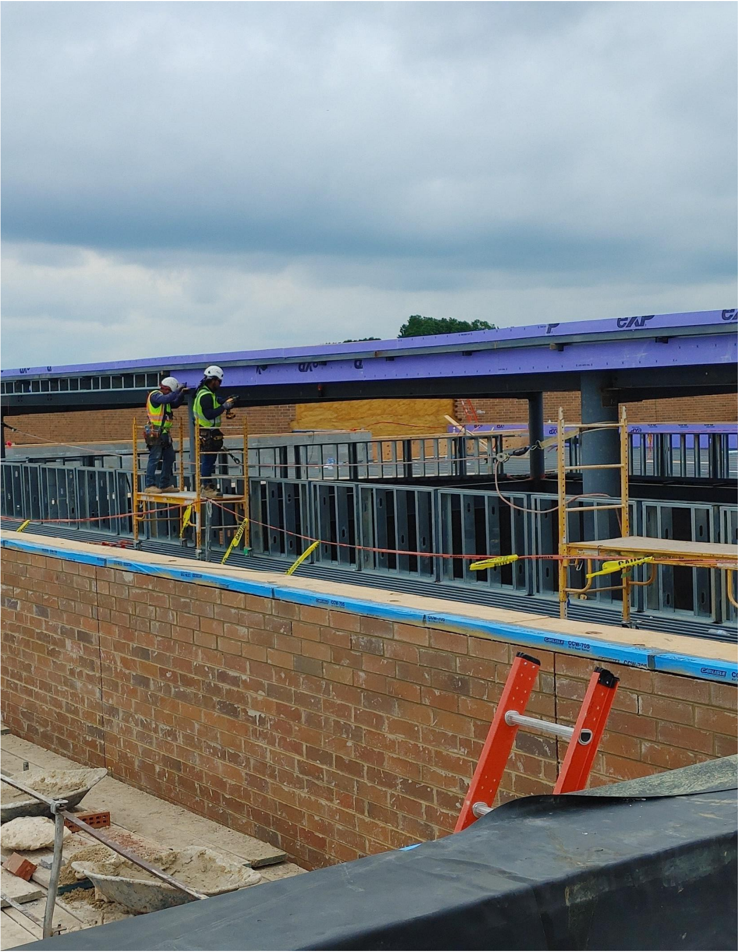
Photo 7 - Gyp Board is being hung on the East side of Area C.
