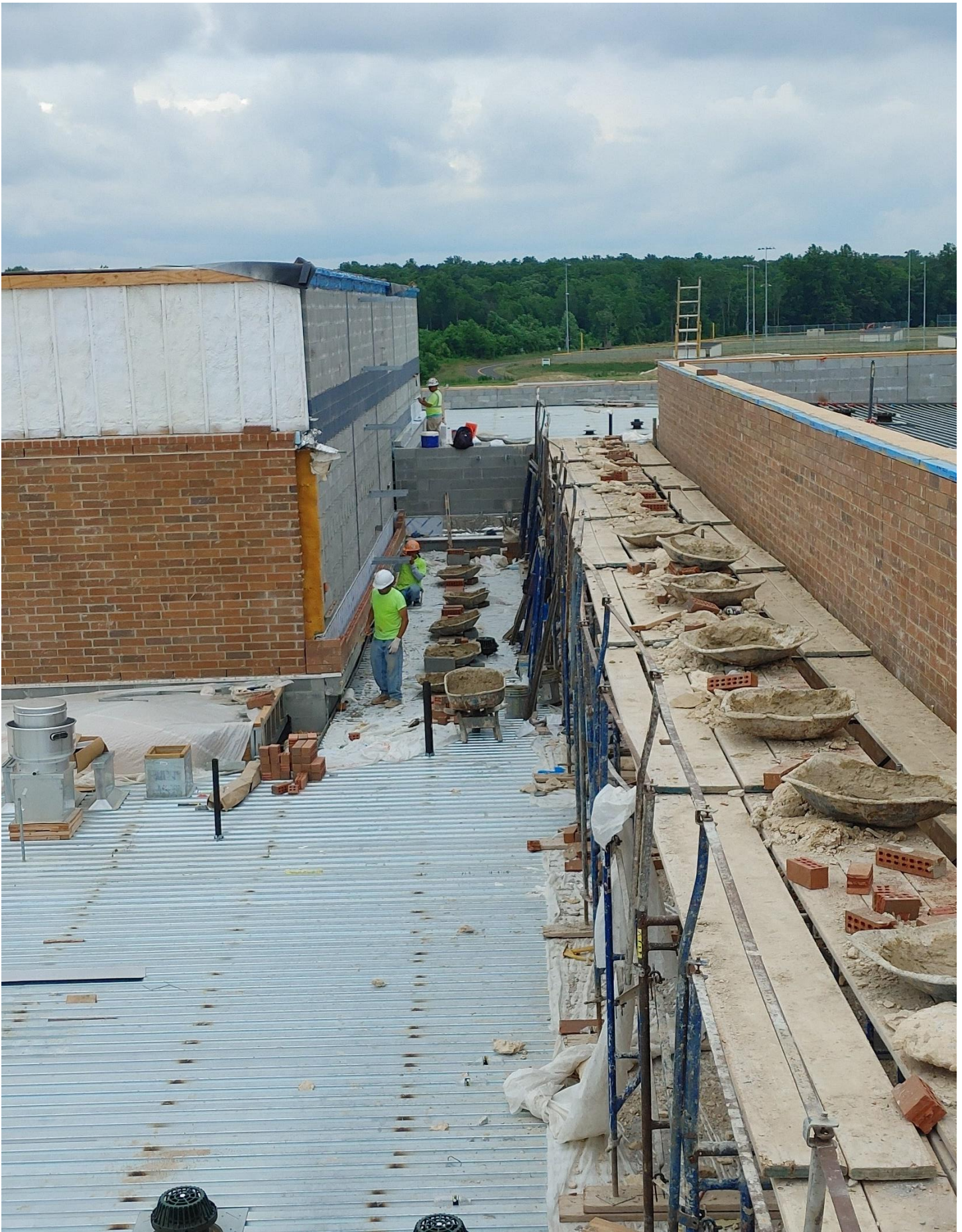
Photo 8 - Brick is being laid and flashing installed on the West side of Area D.
