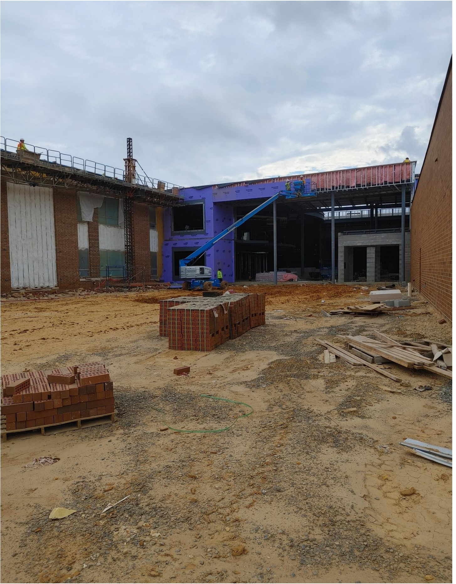
Photo 5 - Brick is being laid on the South side of Area B and Gyp Board is being installed in the West side of Area C.
