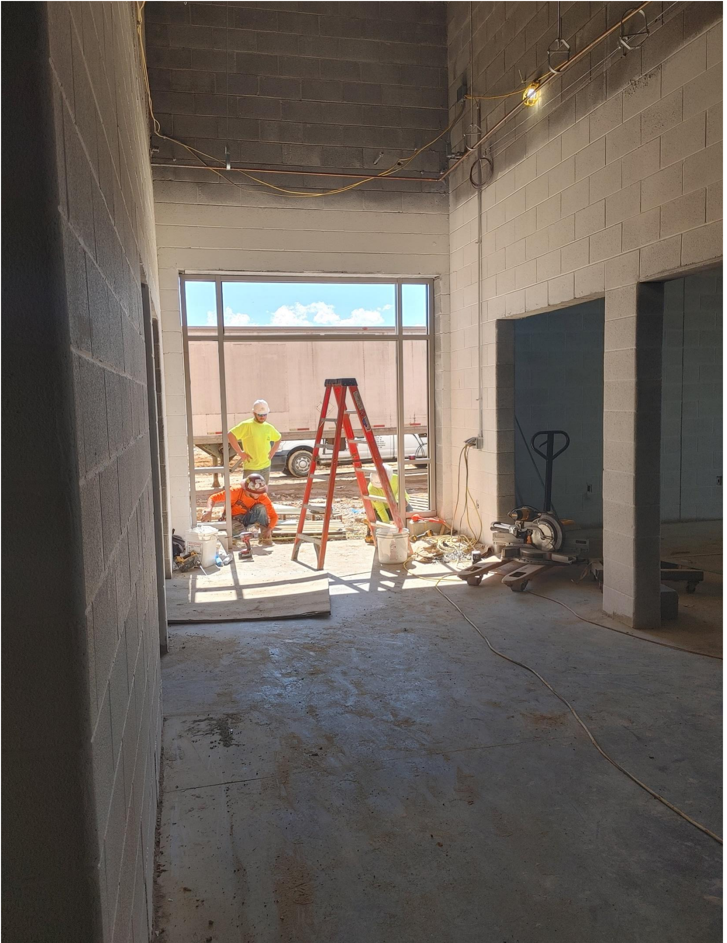
Photo 7 - Storefront SF21 is being set on the East side of Area D.
