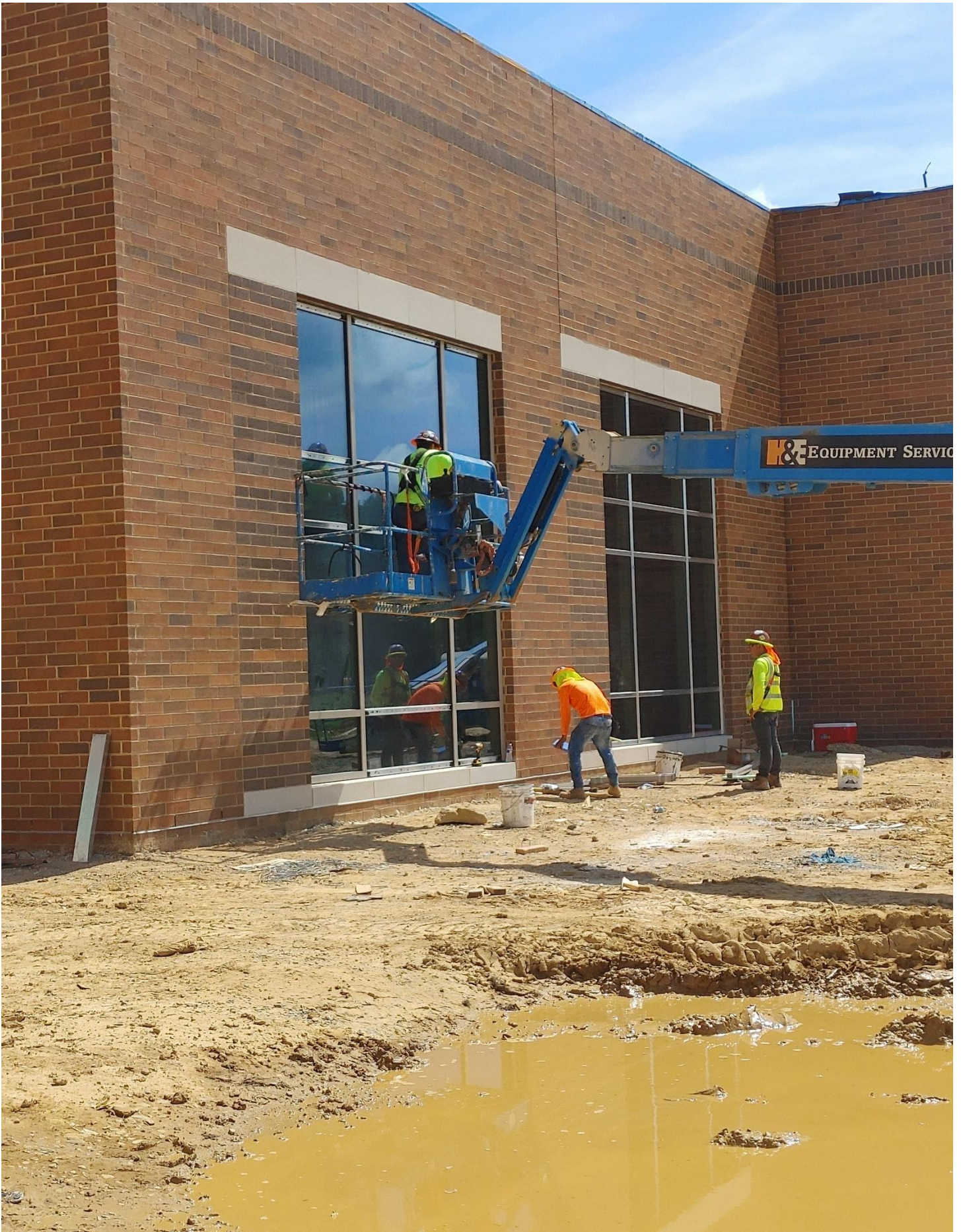
Photo 4 - FG&M are working on the Curtain Walls on the South side of Area D.
