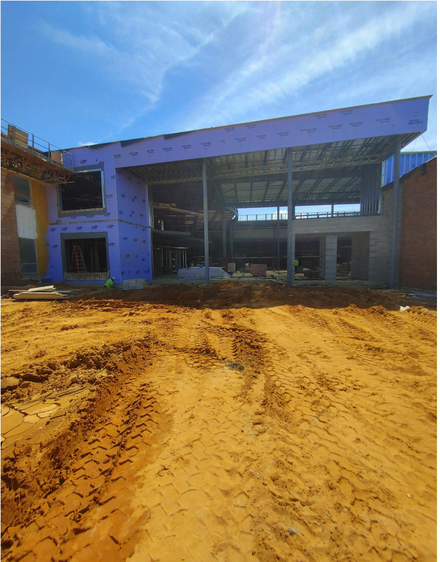
Photo 5 - Footer on the West side of Area C is being prepped for Precast.
