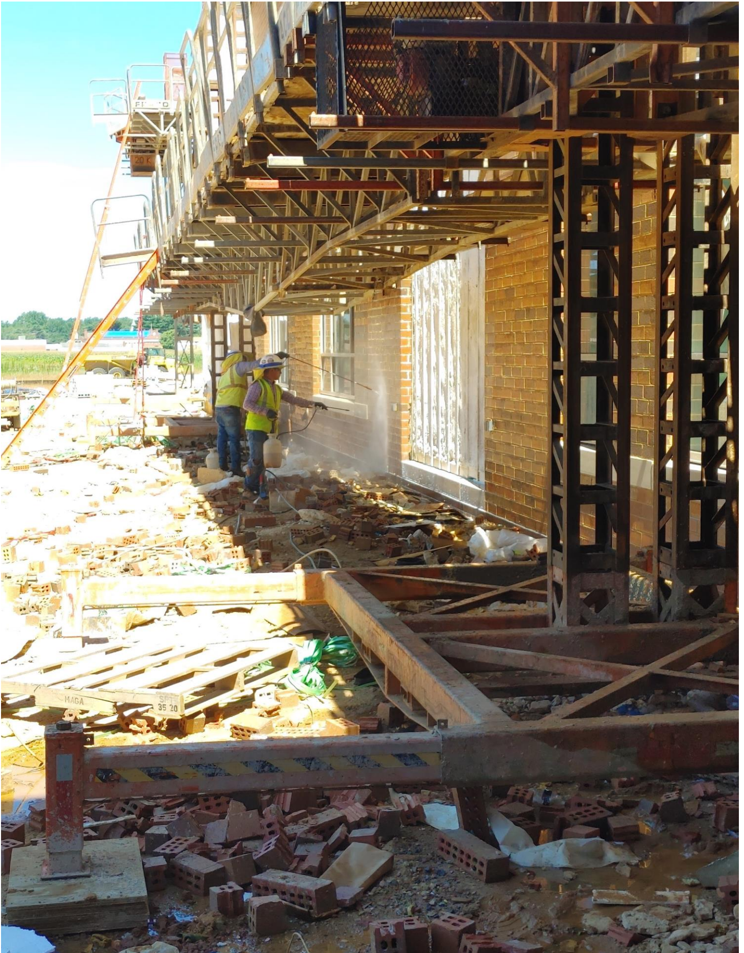
Photo 6 - Brick and Precast is being Power Washed on the South side of Area B.
