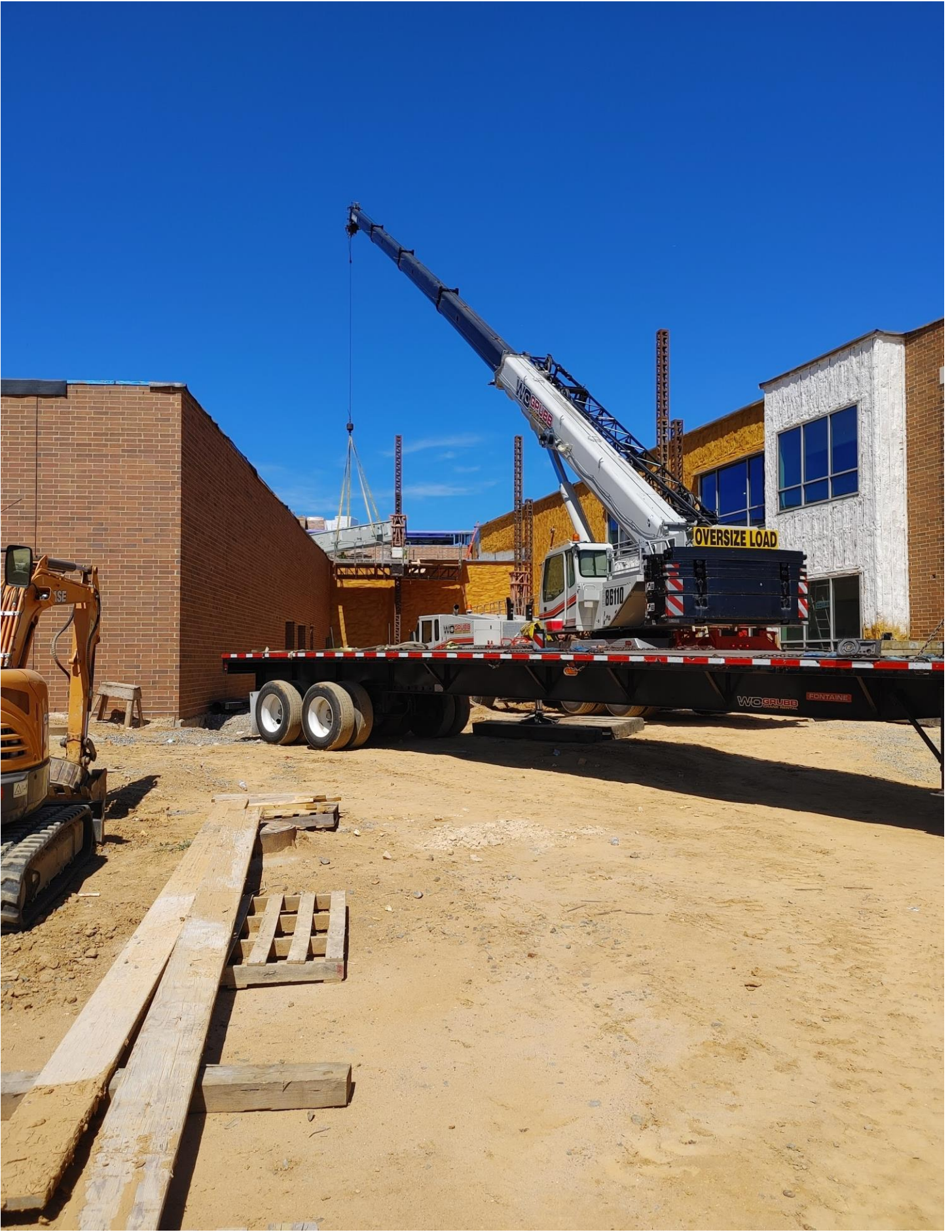
Photo 9 - Roof Top HVAC Unit is being set on the low roof of Area D.
