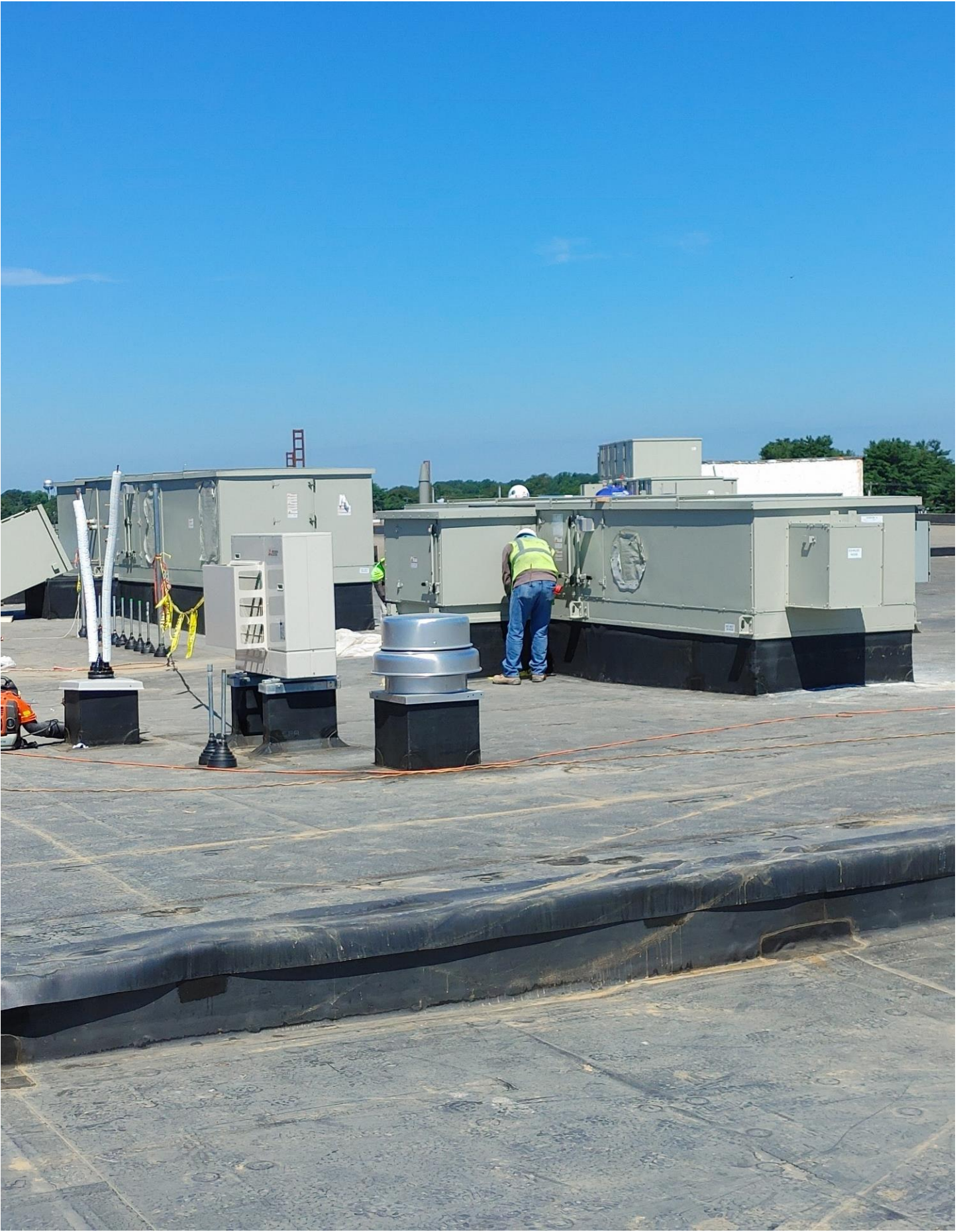
Photo 1 - Two Roof Top Units have been set on the Roof of Area A
