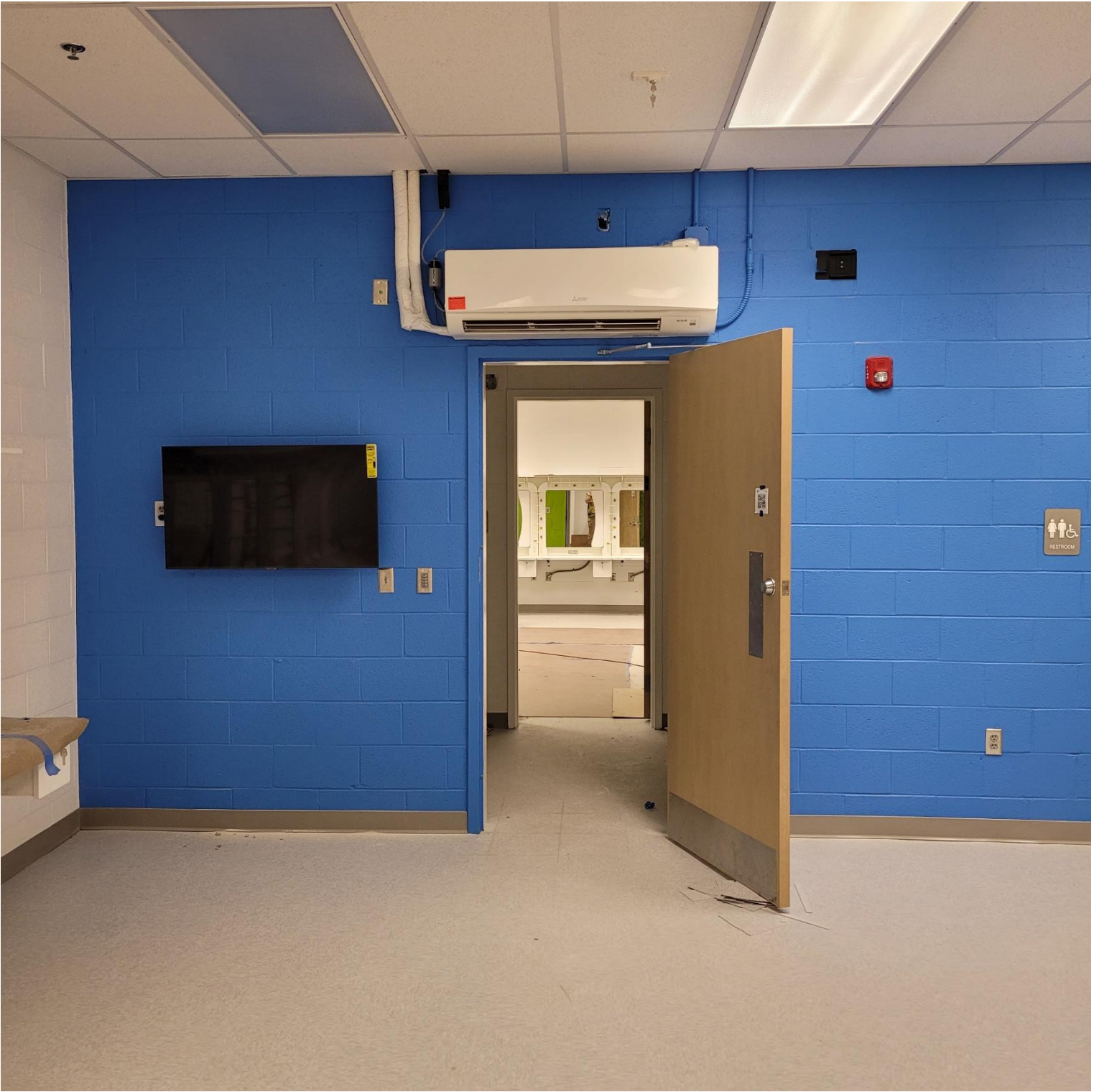
Photo 8 - HVAC Unit in Room #132 mounted on Door Frame.
