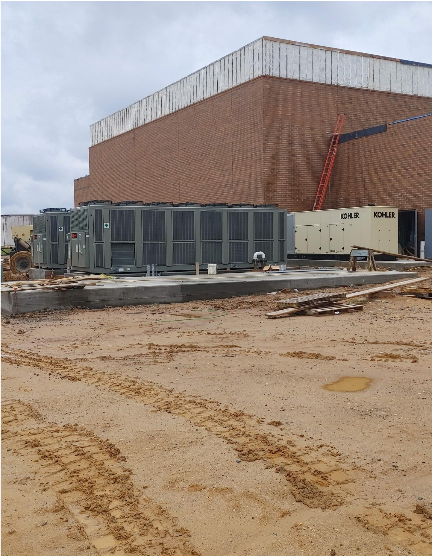
Photo 1 - Chillers and Generator have been set
