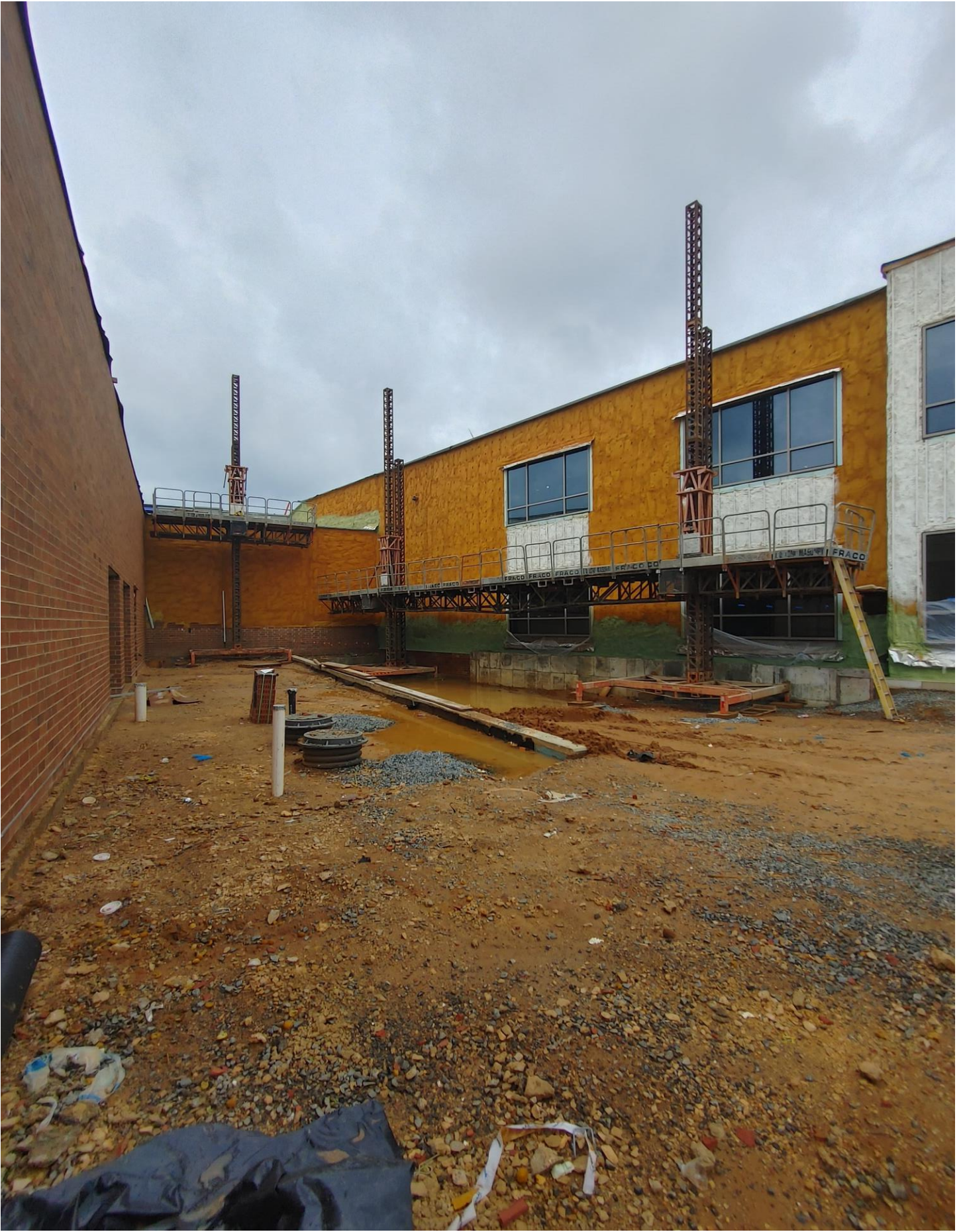
Photo 2 - FRACO has been set up on the South side of Area A
