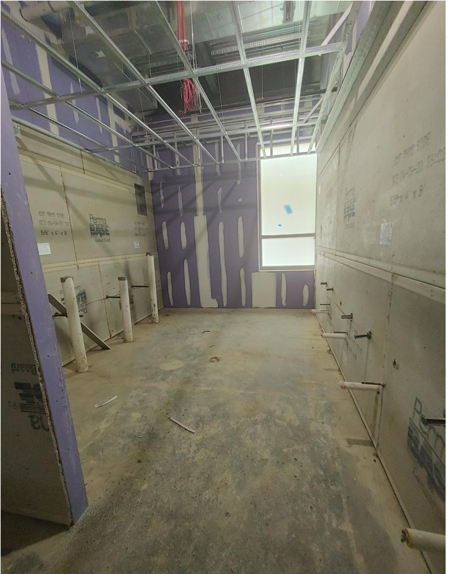
Photo 7 - Cement Board has been hung in the 1st floor bathrooms in Areas A & B.
