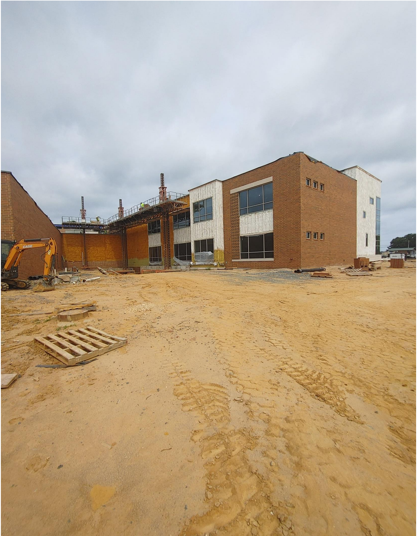
Photo 1 - Masons are laying brick above the low roof of Area C on the South side of Area A
