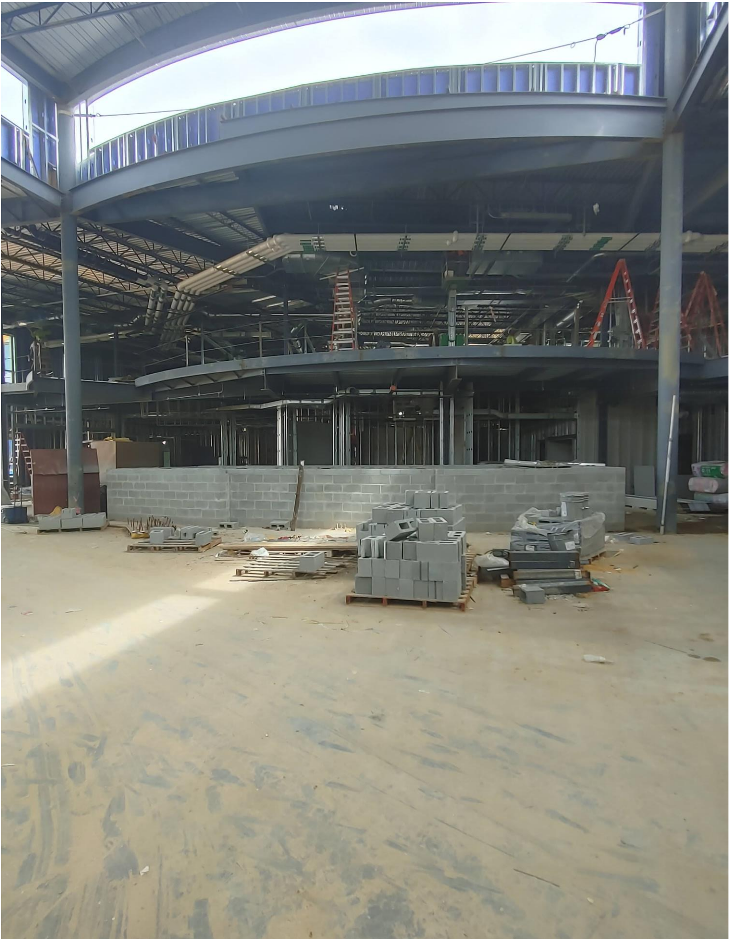
Photo 4 - Duct work is being run and pipe insulated on the 2nd floor of Area A.
