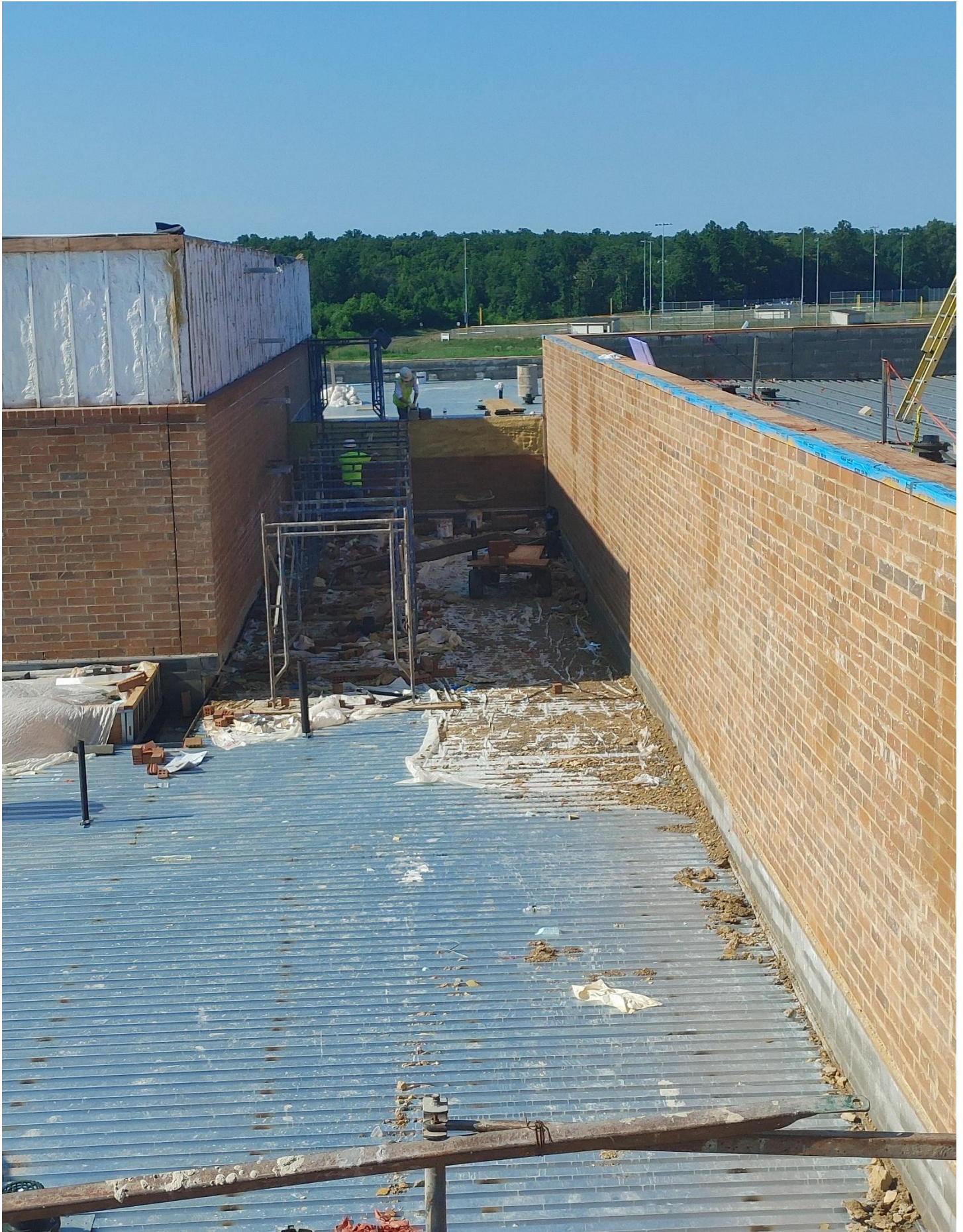
Photo 2 - Scaffolding is being taken down on the low roof of Area D.
