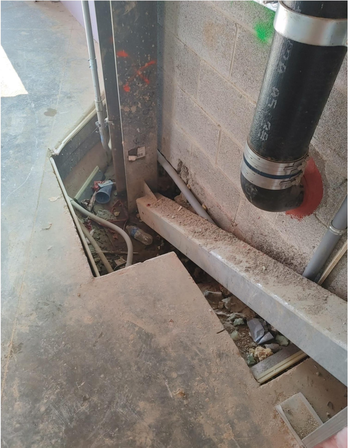
Photo 3 - Area in the North East Corner of Area A, Administrative Offices that still needs to be poured.
