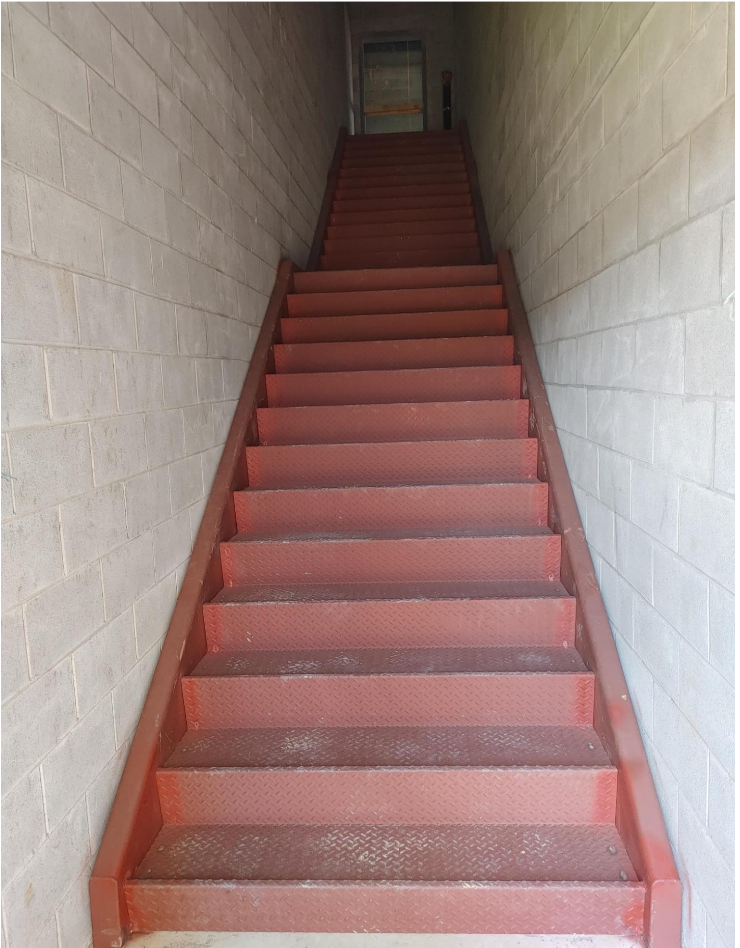
Photo 9 - The Stairs have been set in Stairwell #4. The top landing still needs to be completed.
