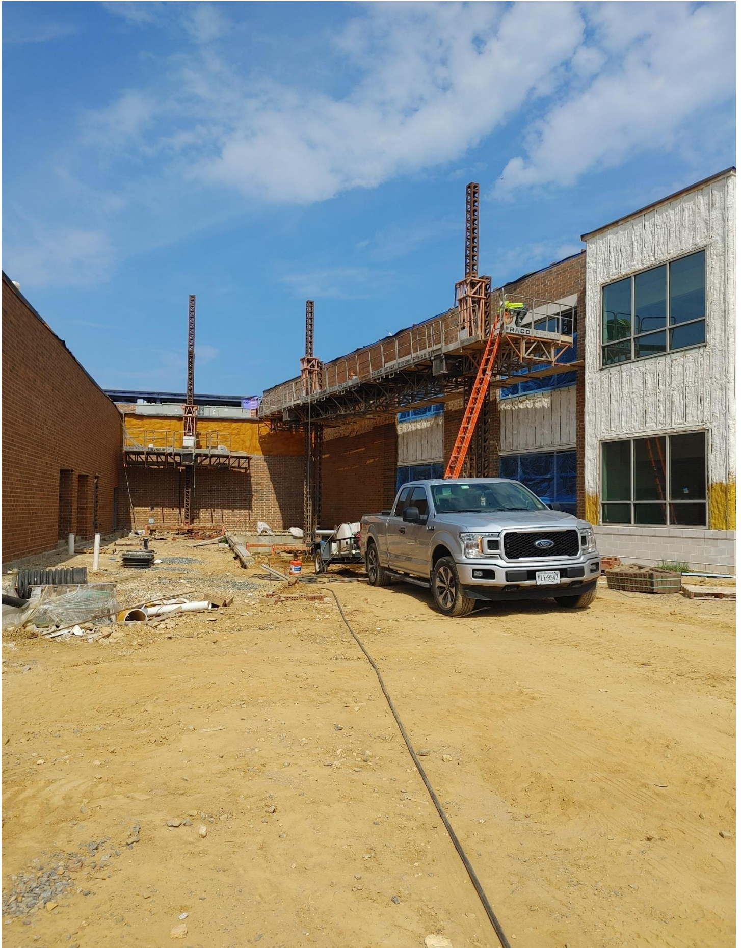
Photo 4 - Mason are Power washing Brick above the low roof in Area C
