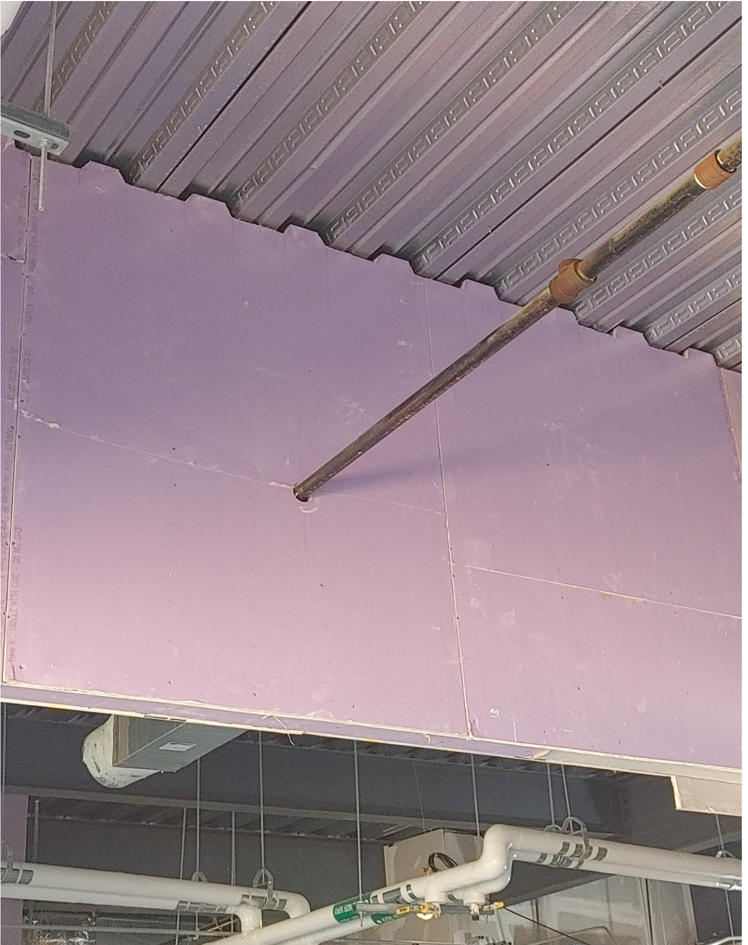
Photo 9 - Sheetrock being cut and hung to match contour of metal pan for fire proofing purposes.
