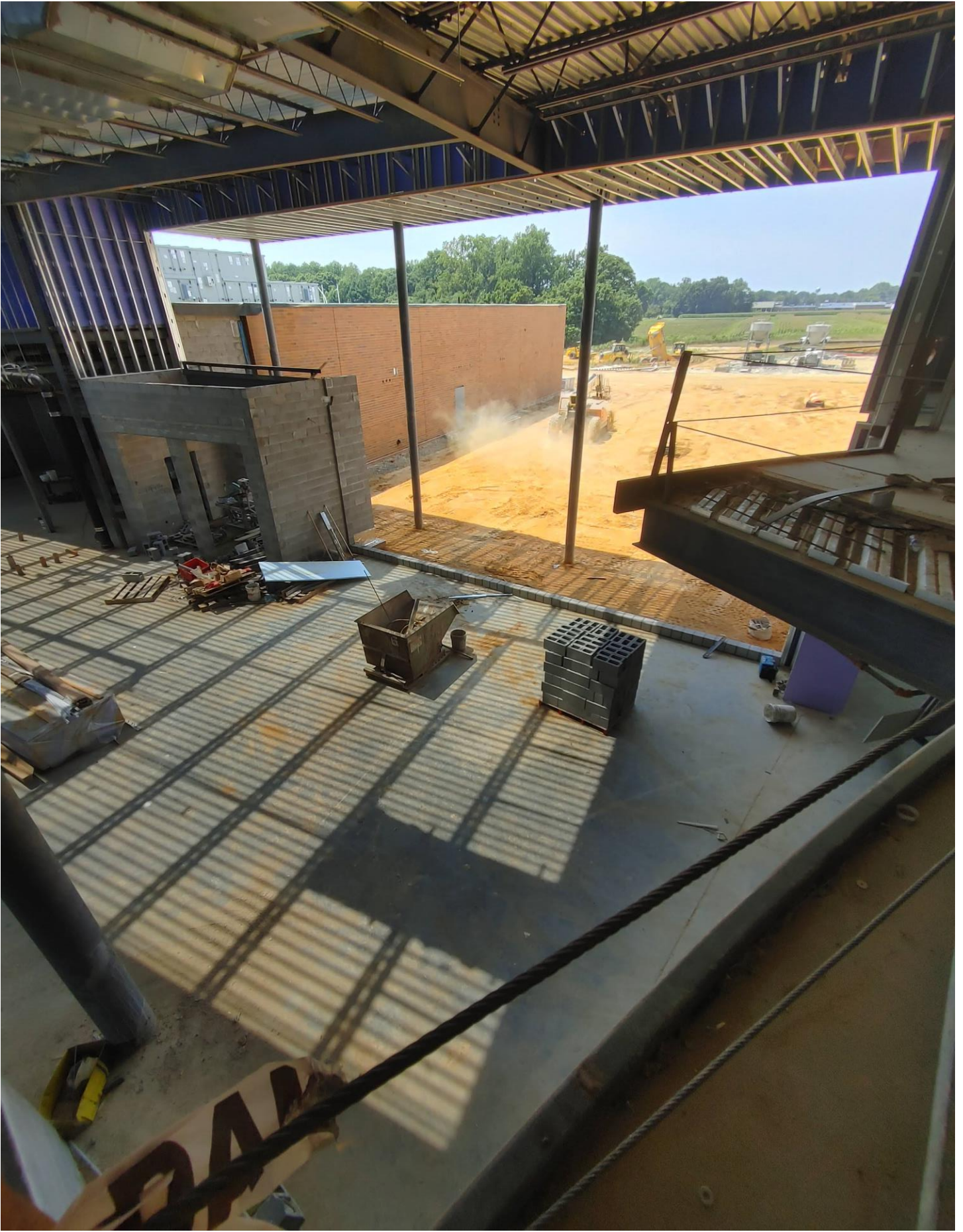
Photo 3 - The Masons have laid the block for Curtain Wall #2 in Area C.
