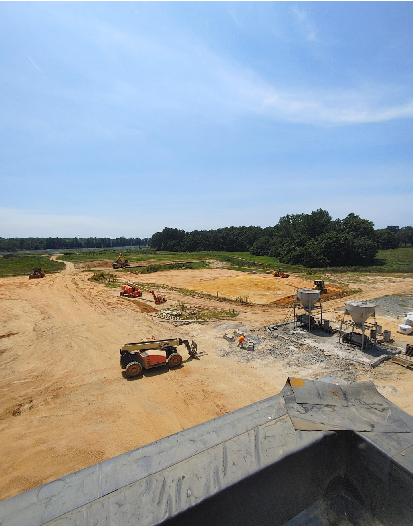
Photo 4 - Beuchert is working on the Retention pond on the West Side of the property
