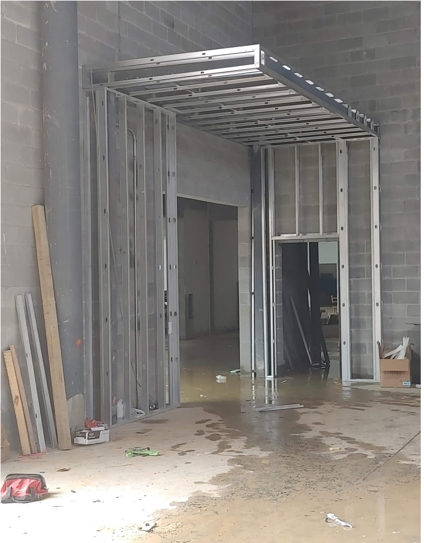
Photo 5 - Canopy has been framed in Area C as you enter Area E.
