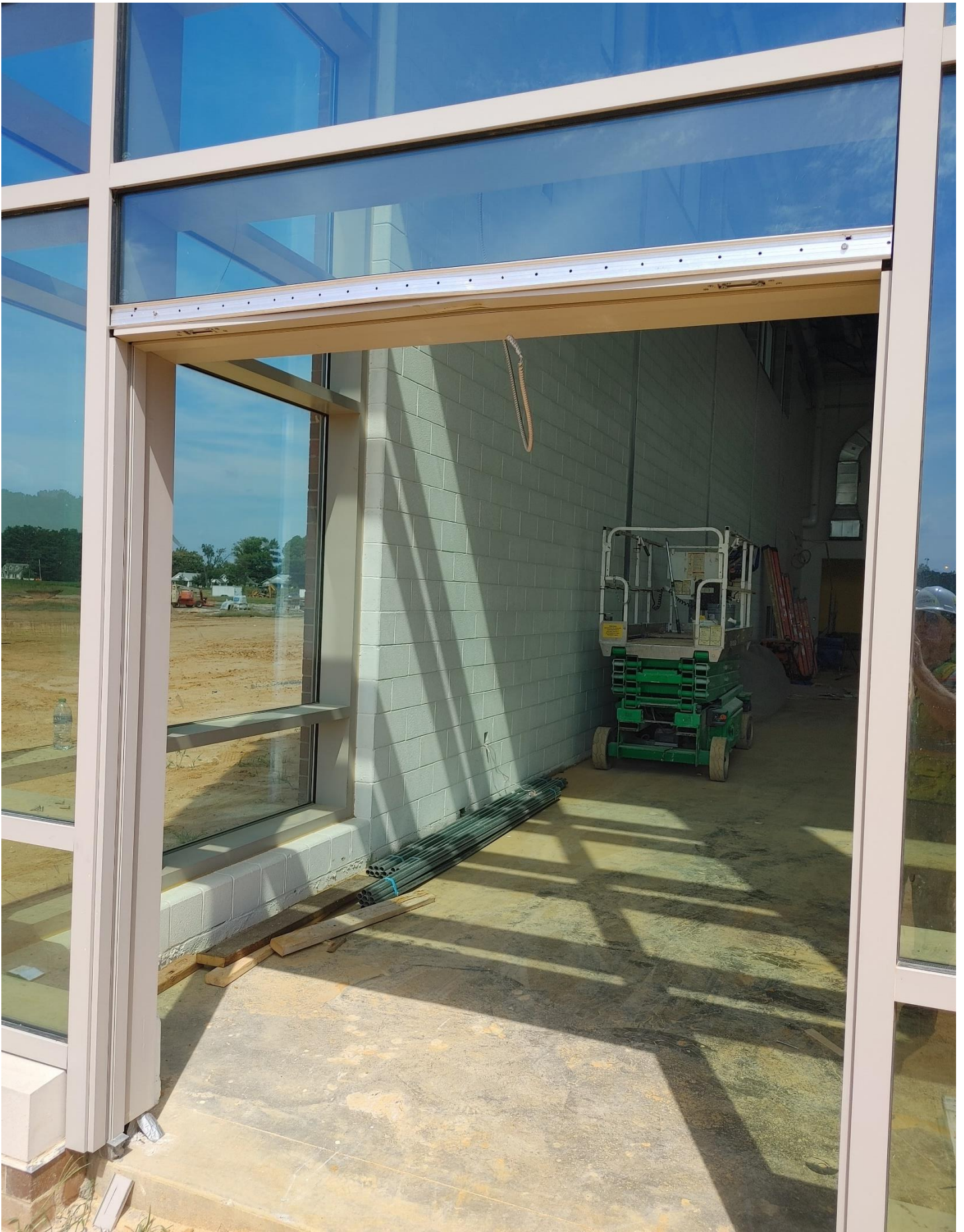
Photo 5 - Damage to XE03, CW4A
