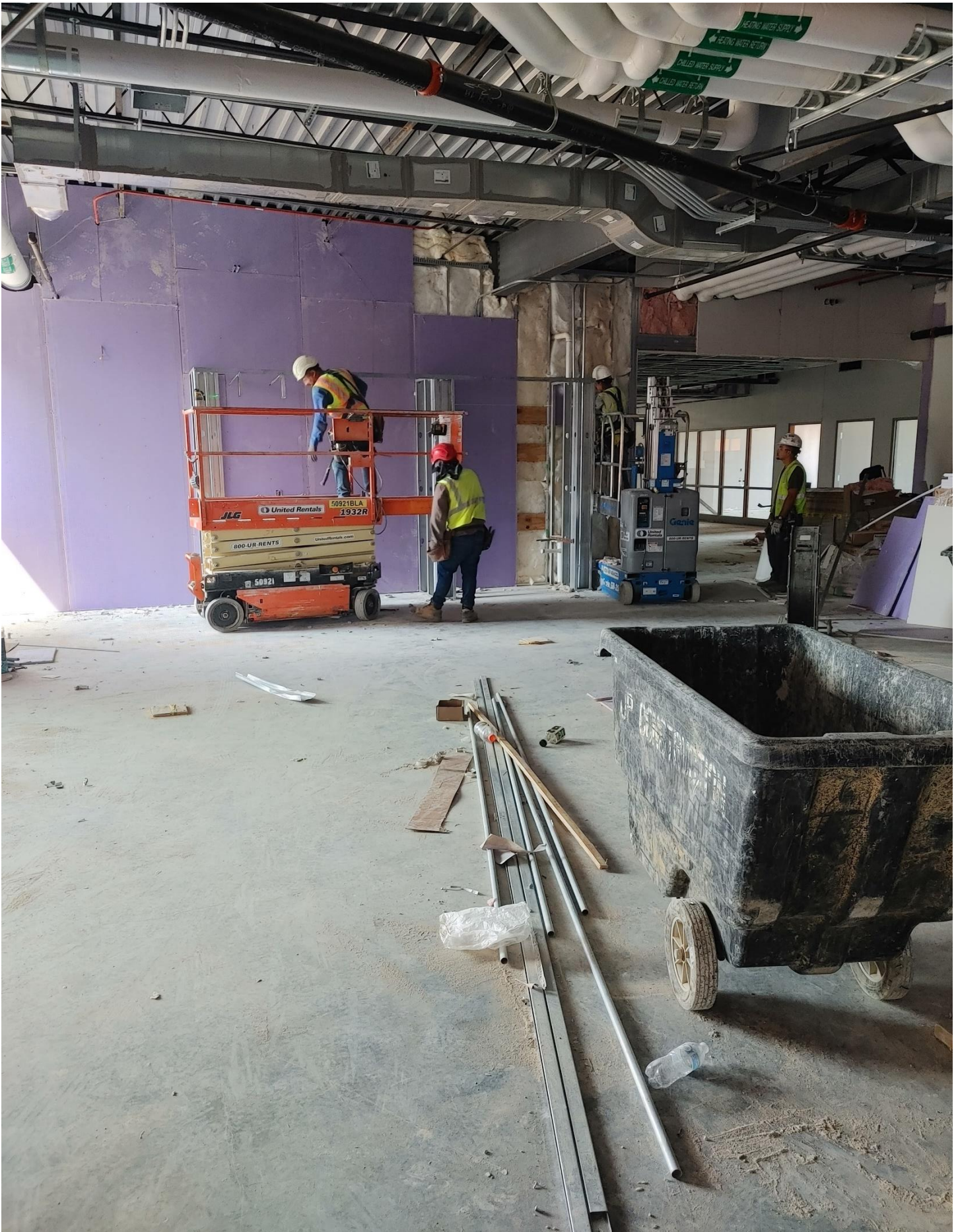
Photo 11 - Built-in Seating Nook and Sink Area on the 2nd floor of Area A is being framed.
