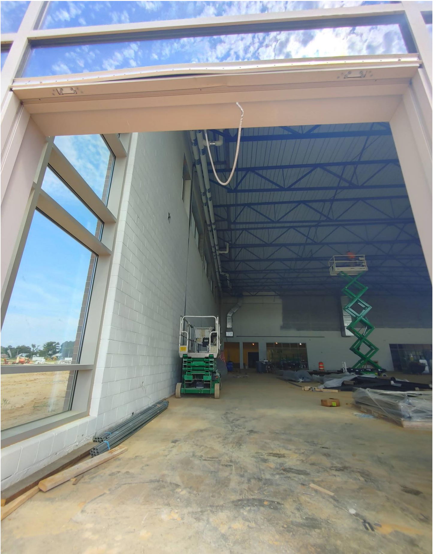
Photo 6 - Damage to XE03, CW4A
