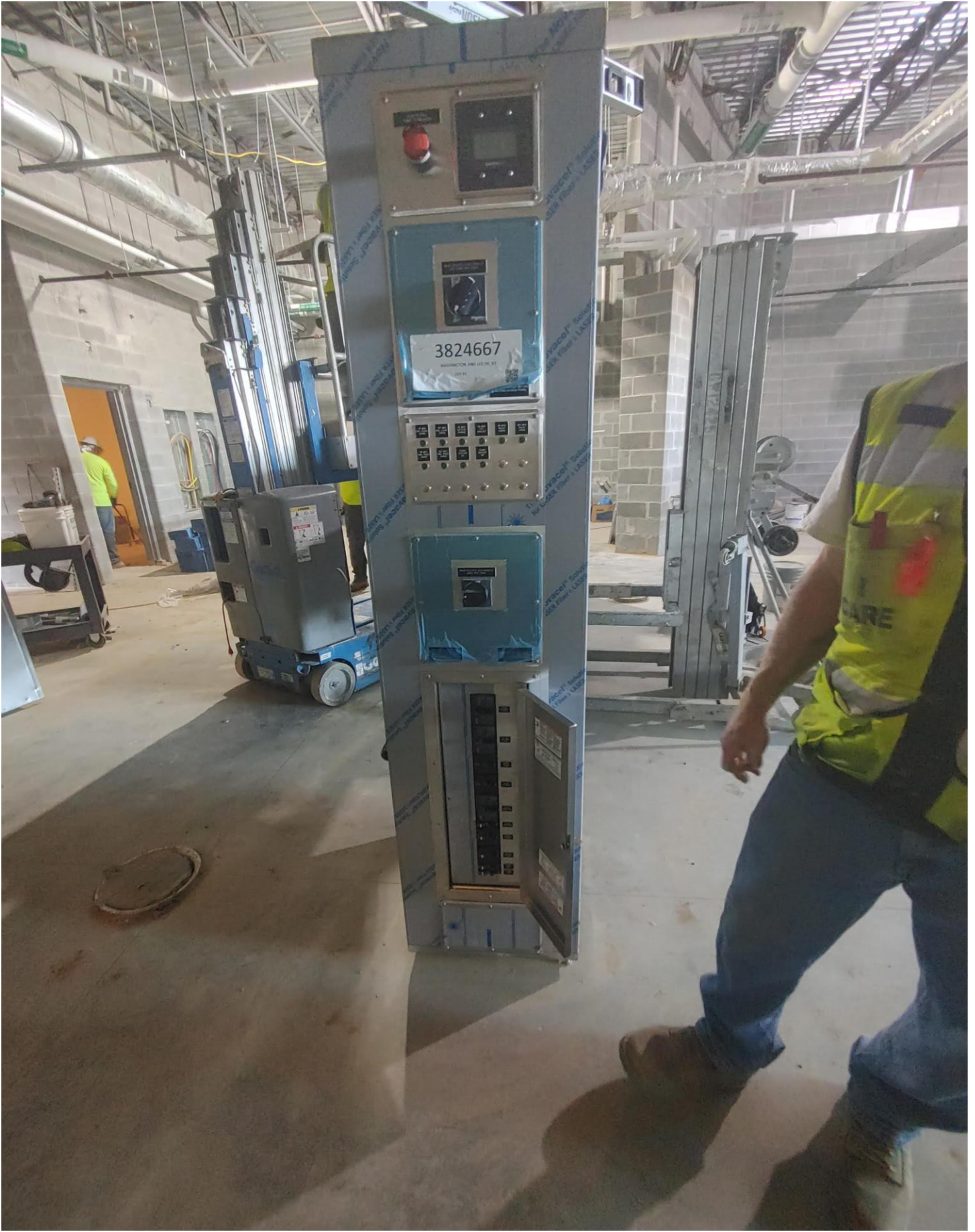
Photo 16 - Utility Distribution System
